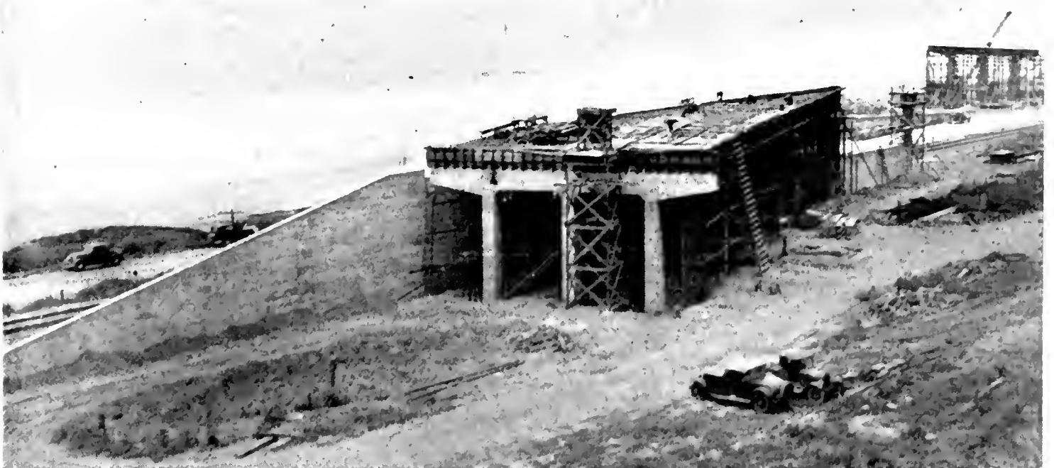
VENTURA OVERHEAD in course of construction. It will separate grades of railroad and highway.
