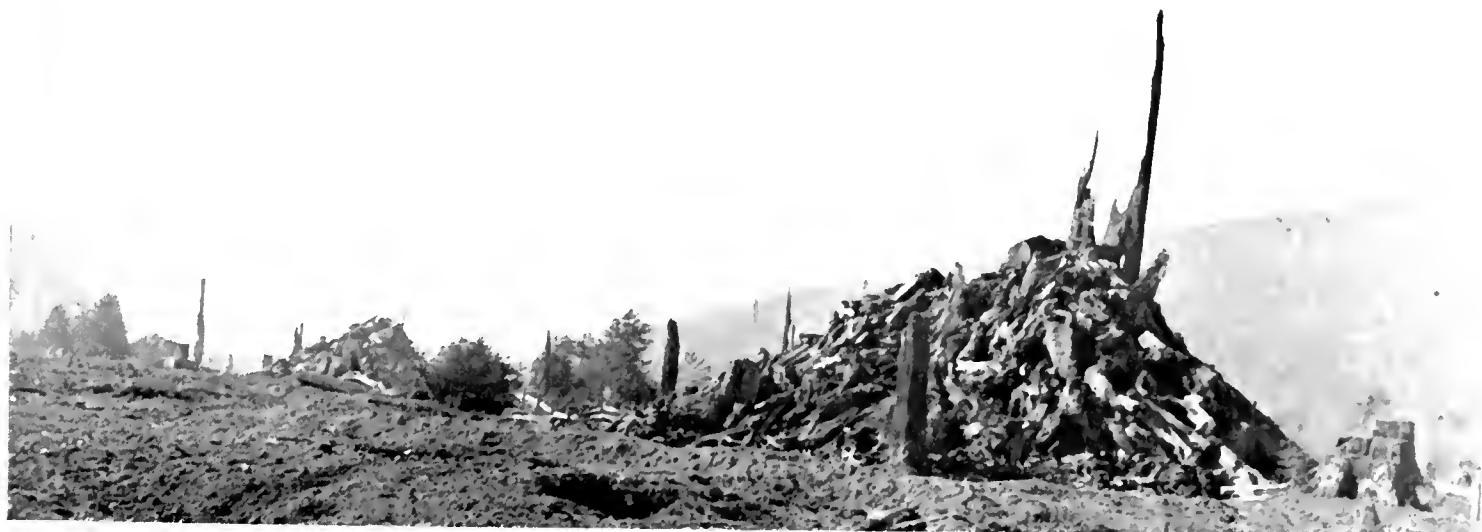
FLAMES LEAPED HIGH when these towering piles of stumps and roots were put to the torch after the clearing operations. There were eight such piles in a distance of 2500 feet.
