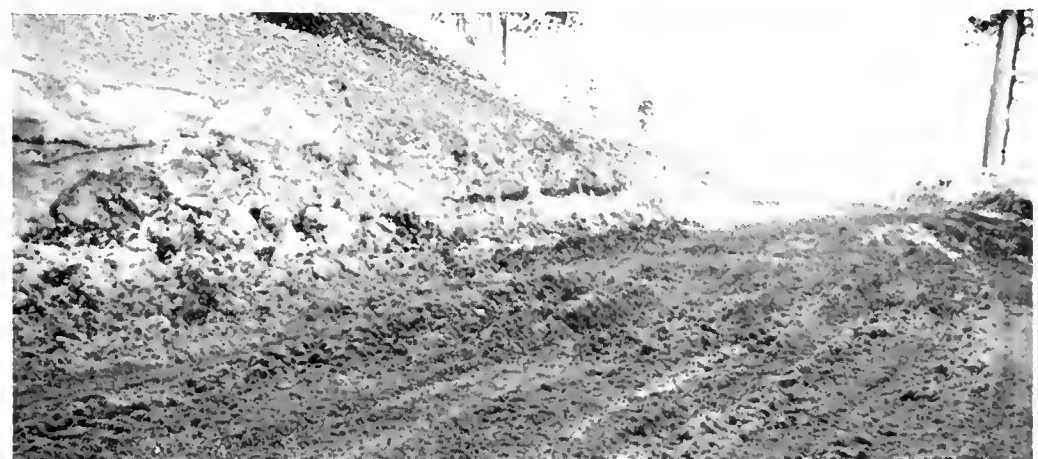
SURFACE FAILURE on State Highway No. 83 due to frost and heavy traffic.
