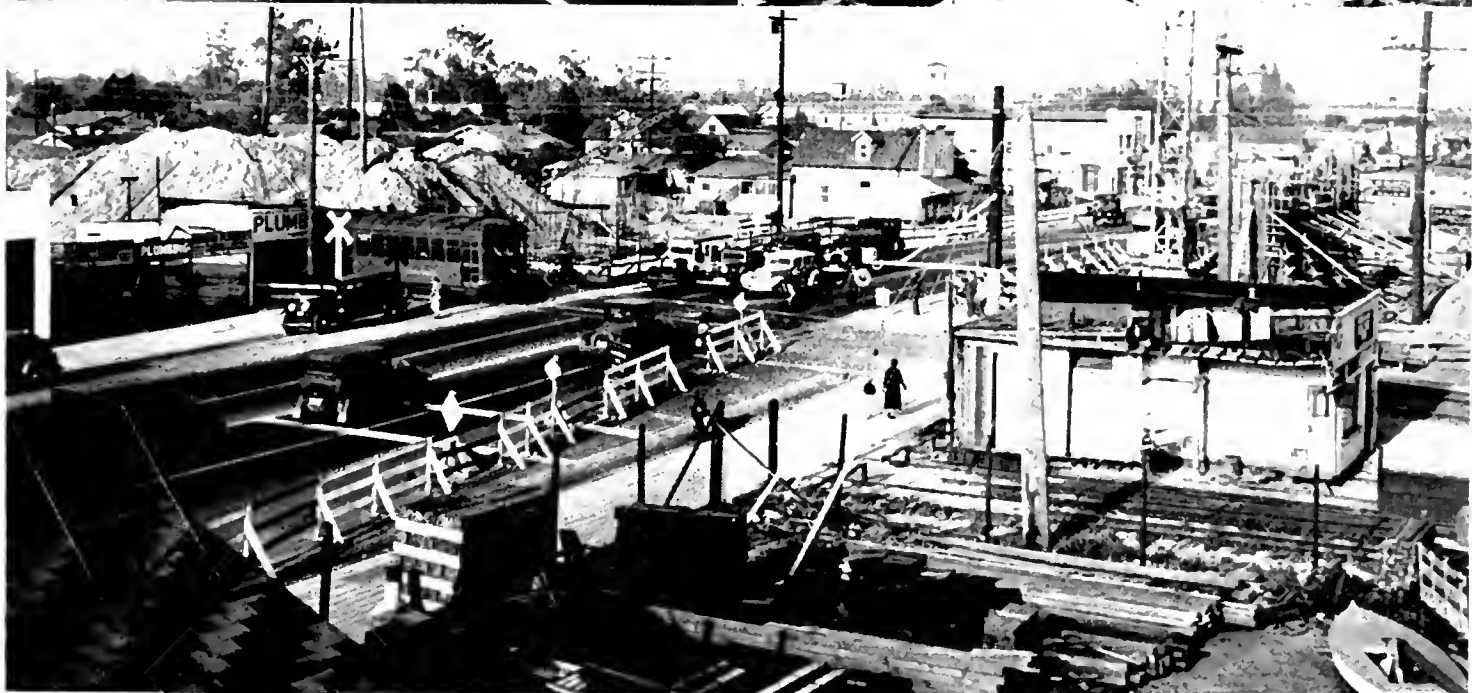
GRADE SEPARATIONS UNDER CONSTRUCTION —At top crossing on State Highway Route No. 19, (Jack Rabbit Trail) near Beaumont showing narrow existing overhead and new structure construction over railroad. Center—Present “s” curve crossing near Indio and new highway overhead structure under way. At bottom—Firestone Boulevard overpass being built in Los Angeles where 490 Pacific Electric trains will daily cross above highway.
