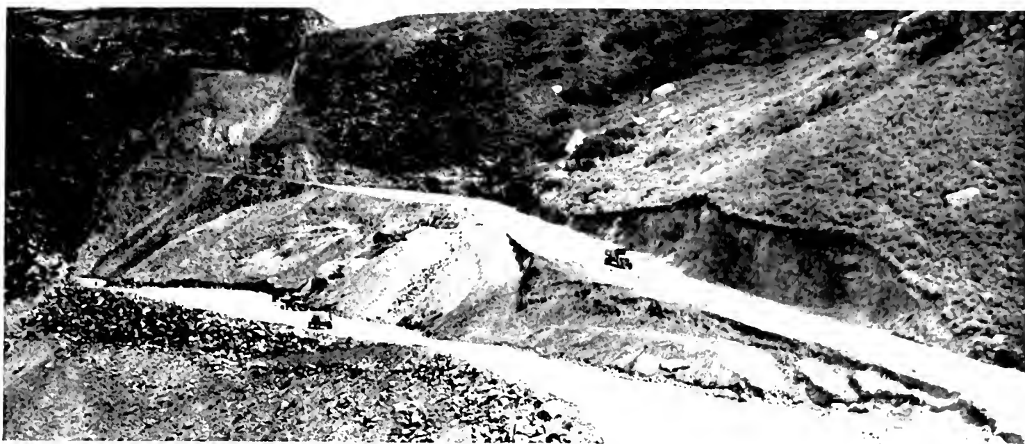
CONEJO GRADE REALIGNMENT—Left foreground, constructing base for big fill which will cover old highway. Upper left, new cut.
