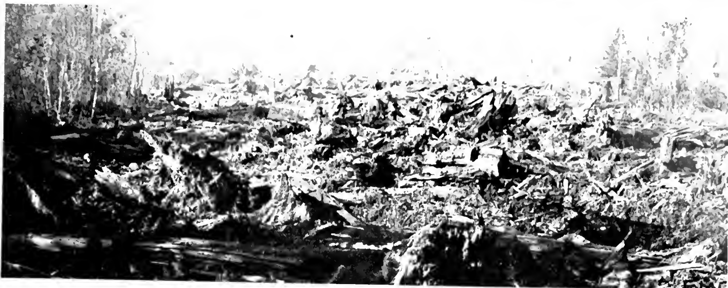
ROUGH GOING for highway builders was encountered on this portion of the Redwood Highway realignment between Jordan Creek and South Scotia Bridge where the debris of old logging days including many huge stumps covered the right of way.
