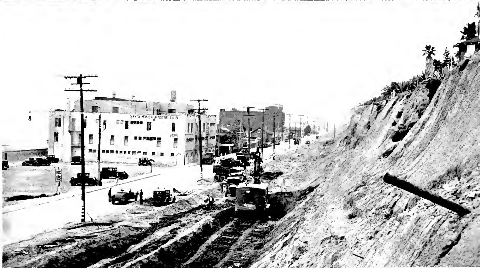
SANTA MONICA COAST HIGHWAY extension and widening operations—In the top picture workmen are constructing reinforced concrete slope protection for retaining walls that support walks and roadways on private property. Center picture shows a portion of the old Southern Pacific Railroad right of way through which the highway will be extended from the shoreline to Lincoln Boulevard by open cut and construction of a 400-foot reinforced concrete arch tunnel under Ocean Avenue and Colorado Avenue in Santa Monica. The tunnel will have a clear span of 56 feet and 48-foot roadway with sidewalks. In the lower picture steam shovel equipment is widening the right of way where the shoreline highway, at its lower end, starts to swing through the cut and tunnel and over Pennsylvania Avenue to the connection with Lincoln Boulevard.
