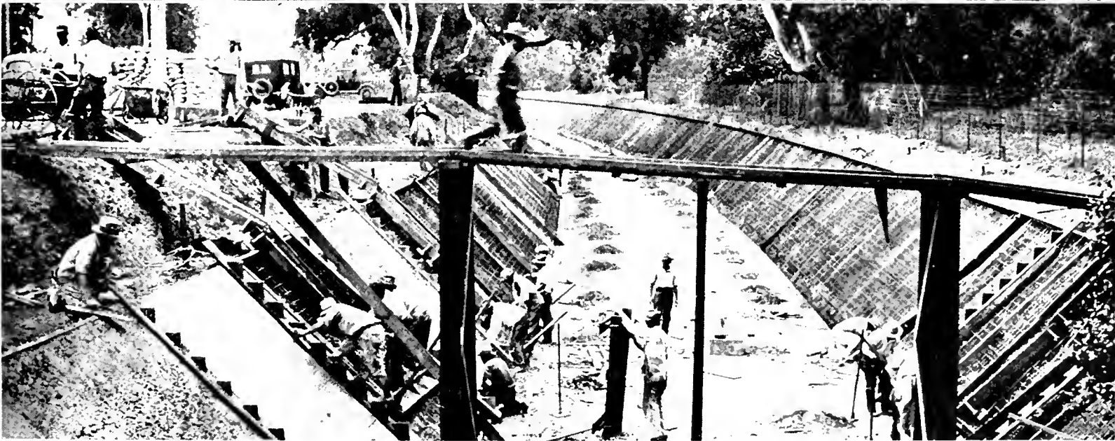
BUILDING TRUCK BY-PASS through the busy city of Santa Barbara. 1—Clearing operations for traffic separation structure. Note dangerous approach of old road to the underpass under railroad. 2—Grading operations near southerly city limits. 3—Constructing a reinforced concrete arch culvert at San Roque Creek. 4—Paving side slopes of new channel for Mission Creek. It will have a 20-foot bottom and 9-foot depth.
