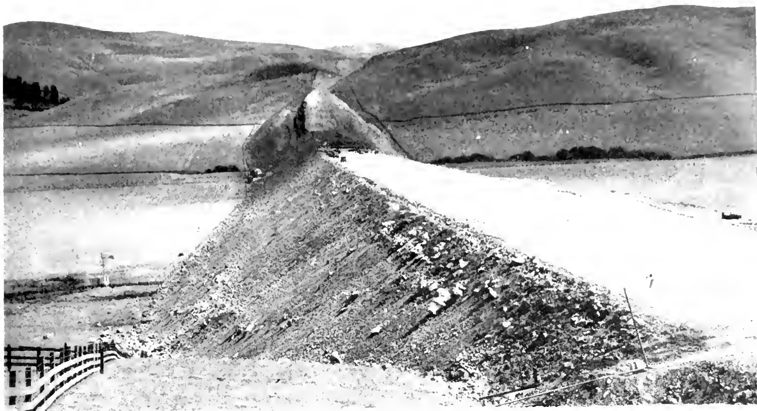
THE "BIG FILL" of the cut-off is rapidly growing to its designed proportions of 75 feet height and 2500 feet length with a width to accommodate a 40-foot pavement. Excess material from the Big Cut slides is being used to raise and widen the fill to its estimated volume of 605,600 cubic yards. In the center of the fill a timber and concrete bridge is being built.
