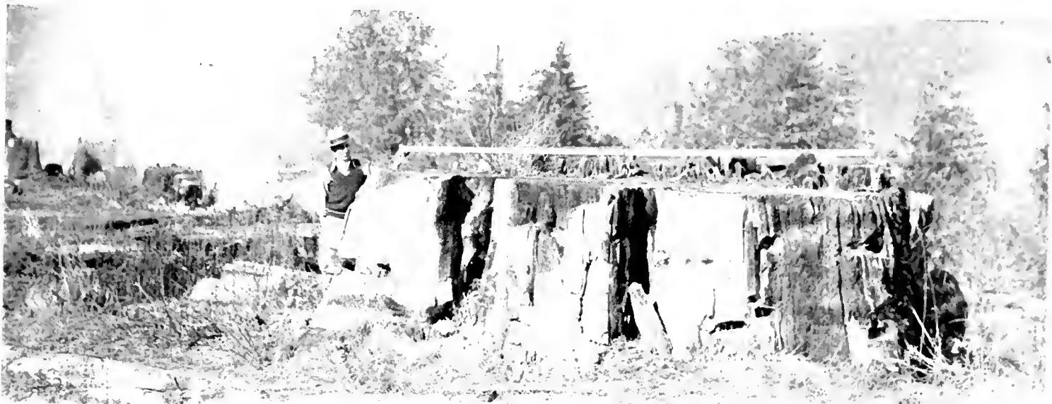
DYNAMITING OPERATIONS were necessary to remove ancient stumps of great redwoods left by the logging crews when the lumber companies were busy in this locality. The stump in the foreground measured over 13 feet in diameter as shown by the 13-foot rod held by the man.
