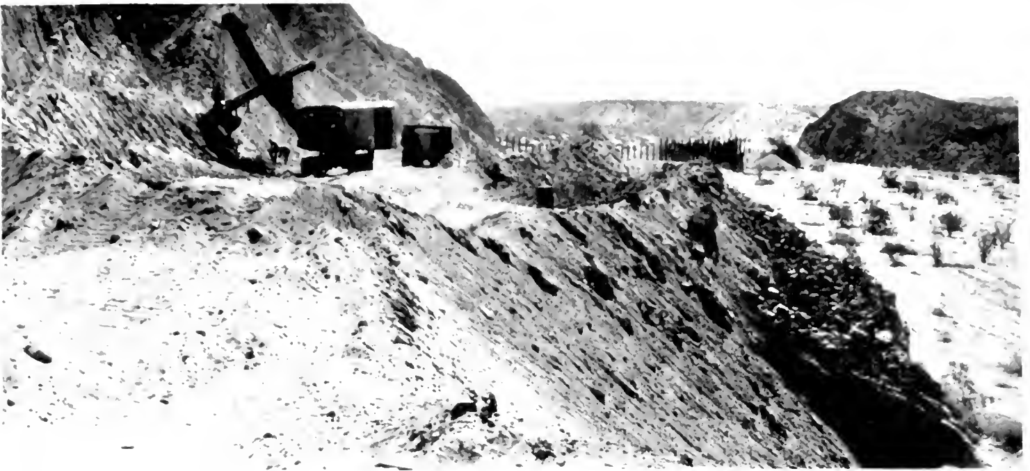
PIONEERING OPERATIONS are well advanced on the Indio Cut-off from Shaver's Wells on the Mecca-Blythe highway to State Highway 26 just south of Indio in Riverside County. The new road is being cut through desert hills as shown in the above picture. Preliminary construction for one of the bridges over a wash is seen in the background.
