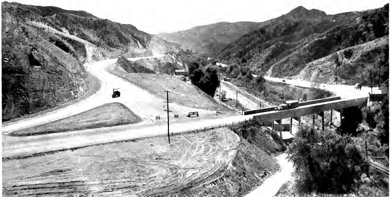
AN IMPORTANT BRIDGE RECONSTRUCTION PROJECT recently completed at Tunnel Station on State Route 4 connects this Los Angeles-Sacramento main highway near its entrance to Weldon Canyon with the Newhall-Saugus route and the Foothill Boulevard cut-off near San Fernando. The widened rebuilt structure is shown at top and below the narrow old structure.
