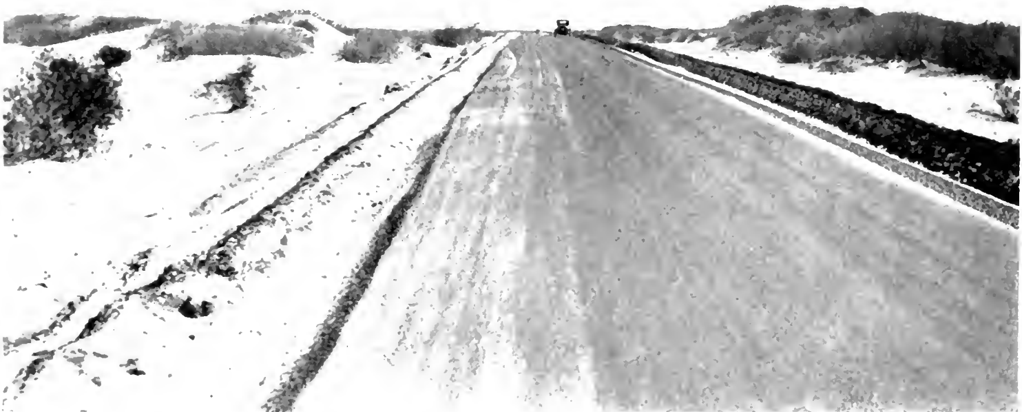
BUILDING DESERT HIGHWAY NEAR CALEXICO. Top—Excavating thousands of tons of ancient beach gravel to provide surfacing material. Center—Grading by tractor and roller scraper and, at right, oil mix subgrade provides substantial base for trucks delivering plant mixed asphalt surfacing. Bottom—Finishing surface course through sand dunes. Roadside not completed.
