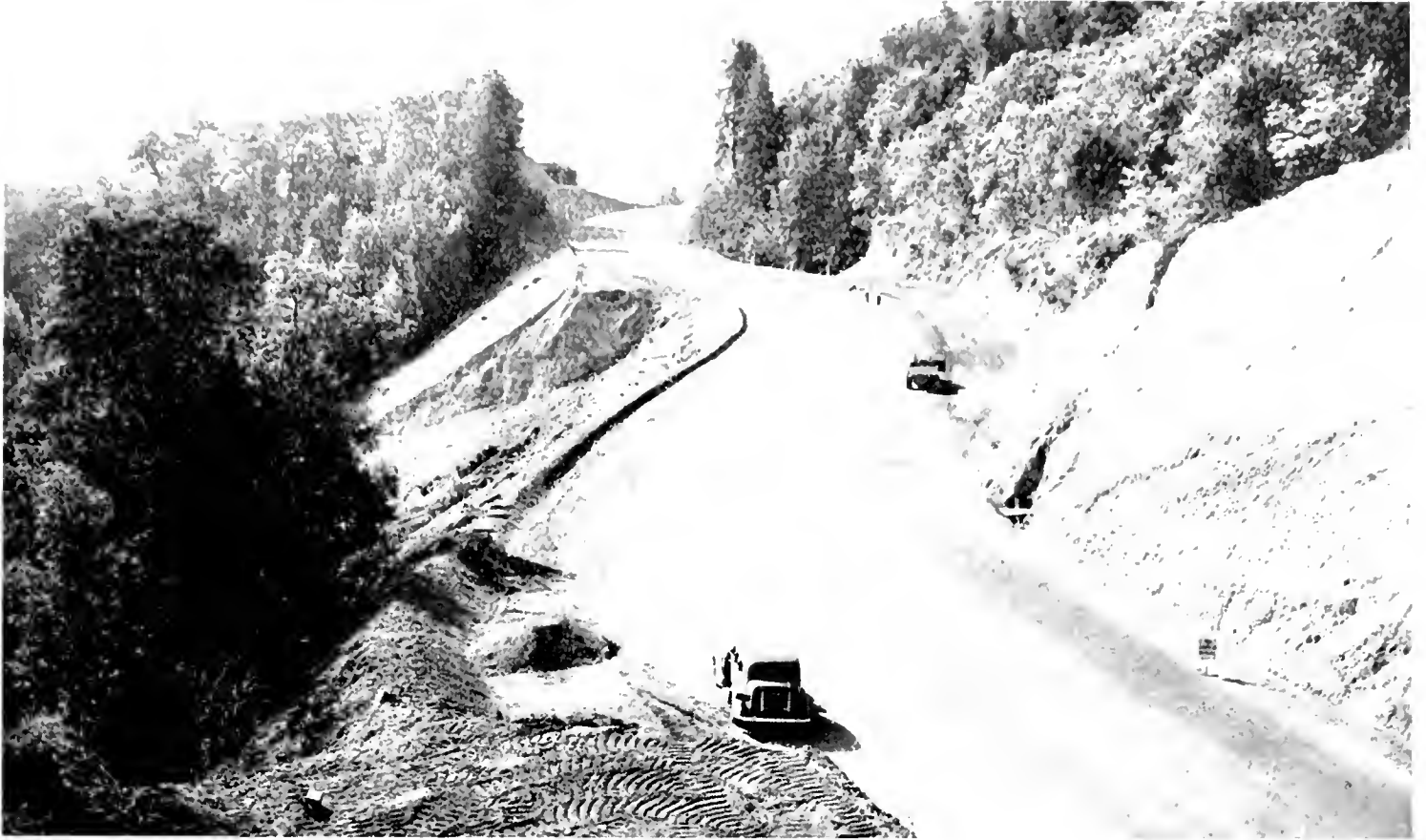
BIG FILL on the Los Gatos-Santa Cruz highway (State Route No. 5) showing where slide occurred threatening to entirely destroy the completed roadway last Spring
