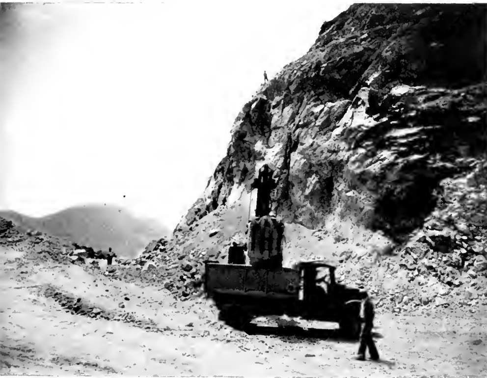
WIDENING OPERATIONS call for heavy work on mountain spurs encroaching on the alignment.
