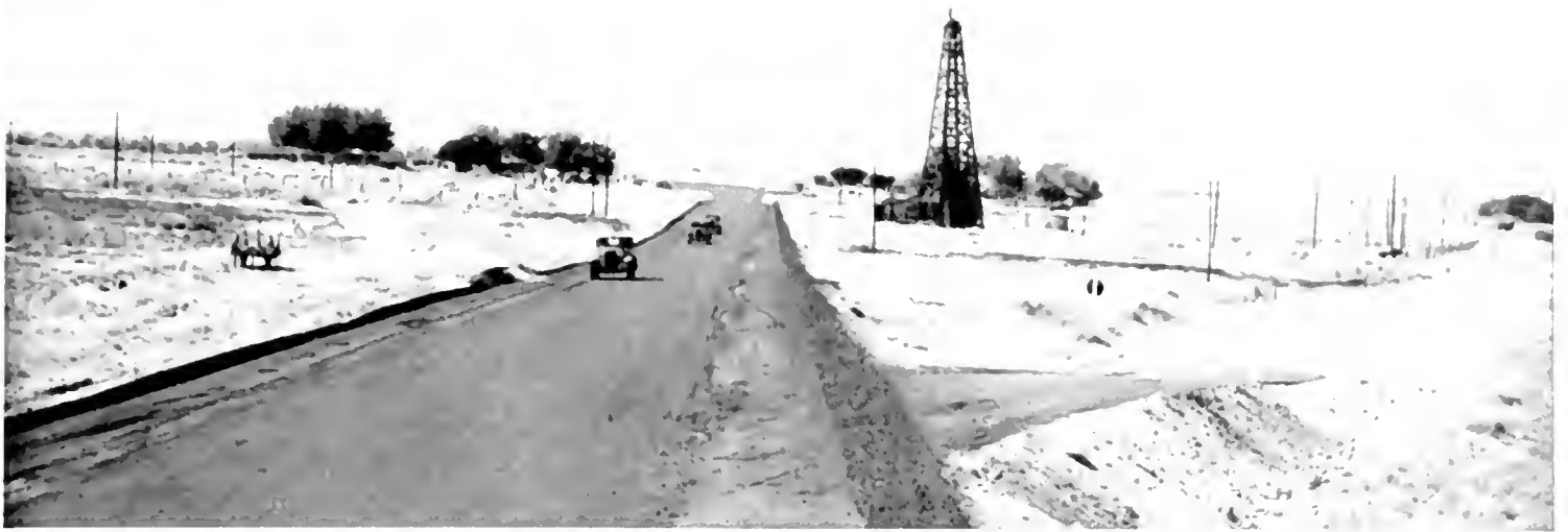
NEW HIGHWAY LINK on a portion of the State Route 138 between Coalinga and Ventura. The photograph shows the east end of the Taft relocation project where it crosses the old highway.
