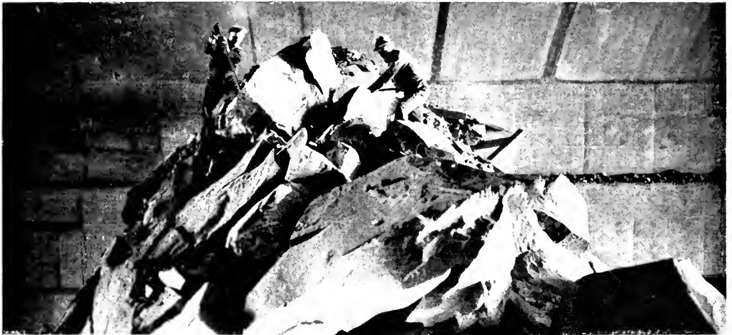
REMOVING LAST OF CORE —A horseshoe shaped excavation was made through the rock which was then concrete and steel lined before the inside or core of the tunnel was dug out.
