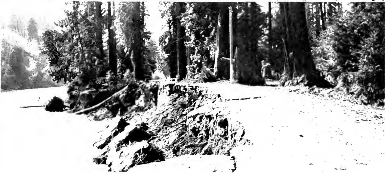
SLIDES AND WASHOUTS of the past winter. At top—A typical slide removal job in Trinity County. Center—Rock slides closing San Marcos Pass. Bottom—Washout on Van Duzen River, State Route 35.
