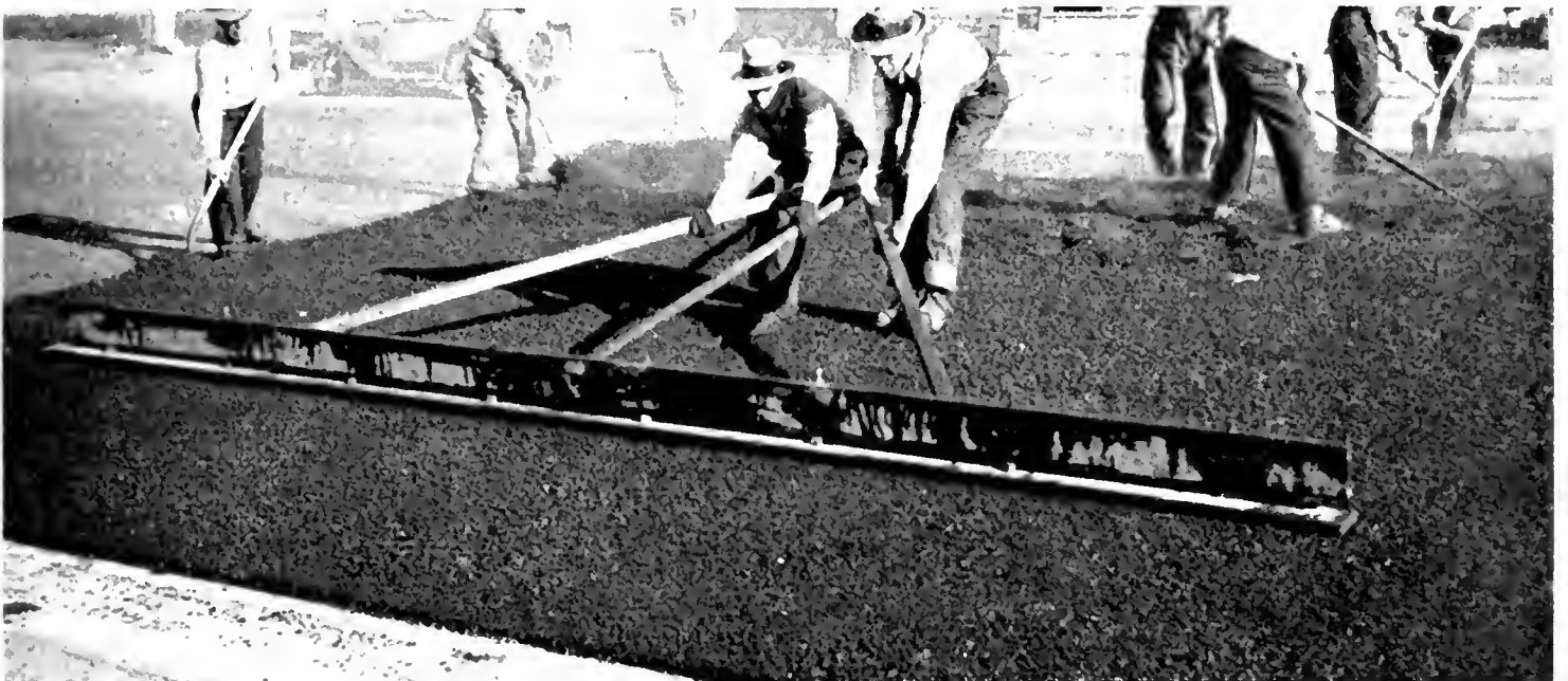
HAND FINISHING warped intersection pavement at Fresno street with 14-foot pole push float.
