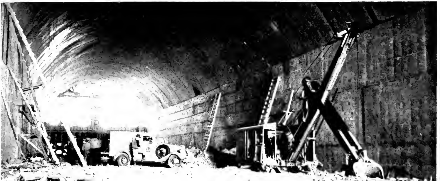
UPPER DECK CONSTRUCTION is begun at far end of tunnel to accommodate six lanes of fast automobile travel. Lower deck will have three truck lanes and two railroad tracks.
