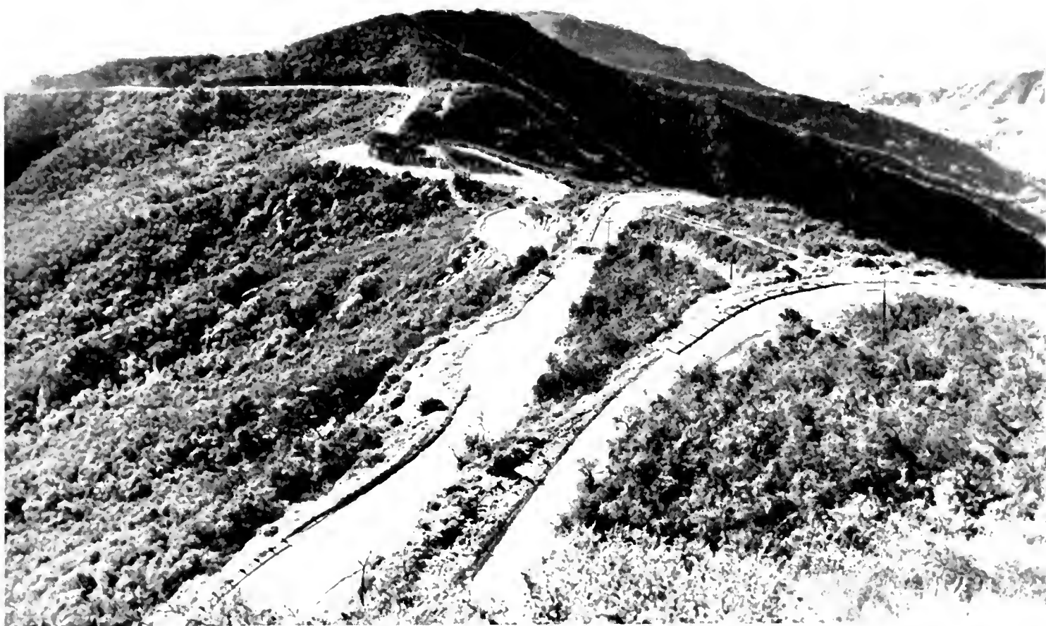
"HAIRPIN" CURVES ON SAN MARCOS PASS road soon to be abolished by realignment. A beautiful ocean panorama is afforded at this point embracing the Santa Barbara Channel Islands shown by dark line at top of picture.
