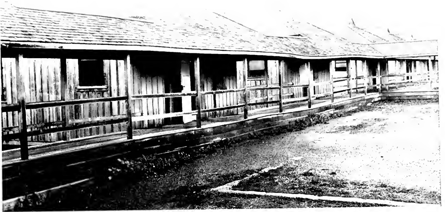
INSANITARY DILAPIDATED WOODEN SHACKS , known as the Dozier cottages, built in 1907 as temporary structures at Napa Hospital, still house 386 women mental patients, including tuberculosis cases.
