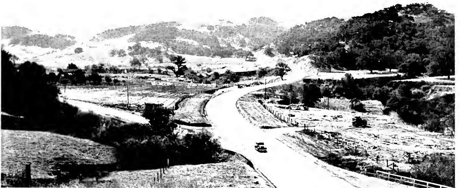
NEW ROUTE climbs through the hills on an easy 6 per cent maximum grade made possible by deep cuts representing 670,000 cubic yards of excavation and shortening the distance by nearly a mile.
