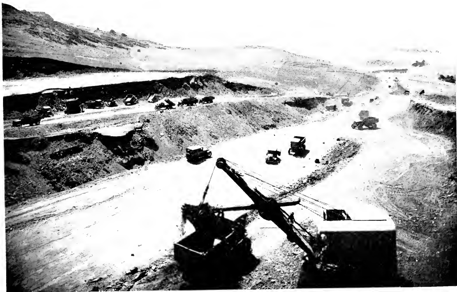
THE "BIG CUT" of the American Canyon cut-off project is the scene of busy operations to prevent further slides of top soil underlain by blue clay that lies in planes at abrupt angles. Power shovels and trucks are at work making broad terraces and removing material above the sliding planes back far enough to prevent further movement into the roadway.
