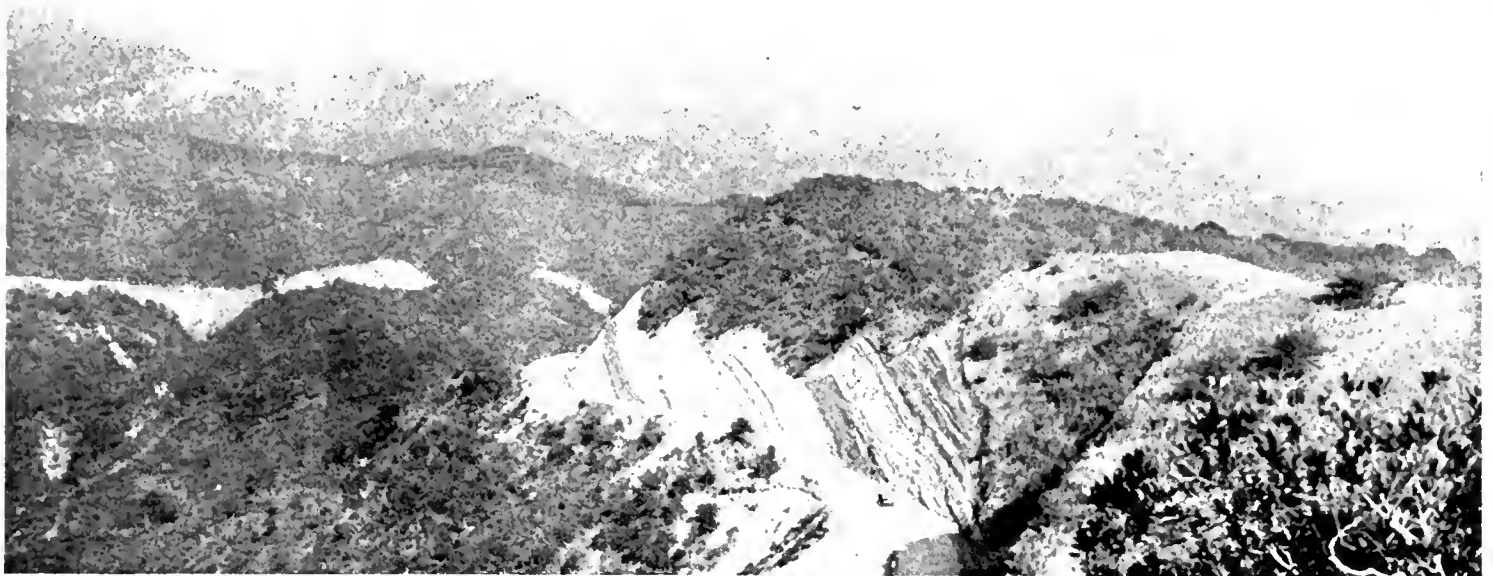
HEAVY SIDE HILL CUT one of several that permitted elimination of hairpin turns and steep grades.
