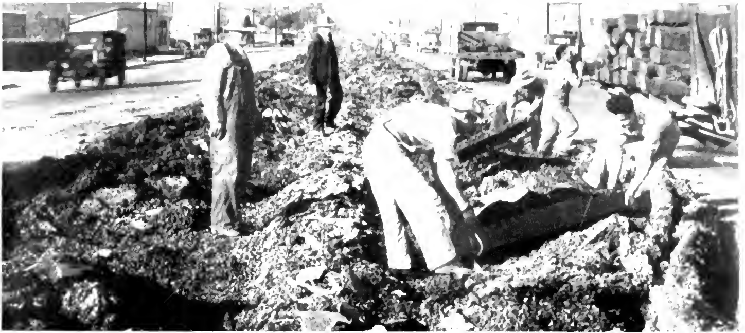
EXIT CAR TRACKS on San Pablo Avenue preparatory to repaving by State contract
