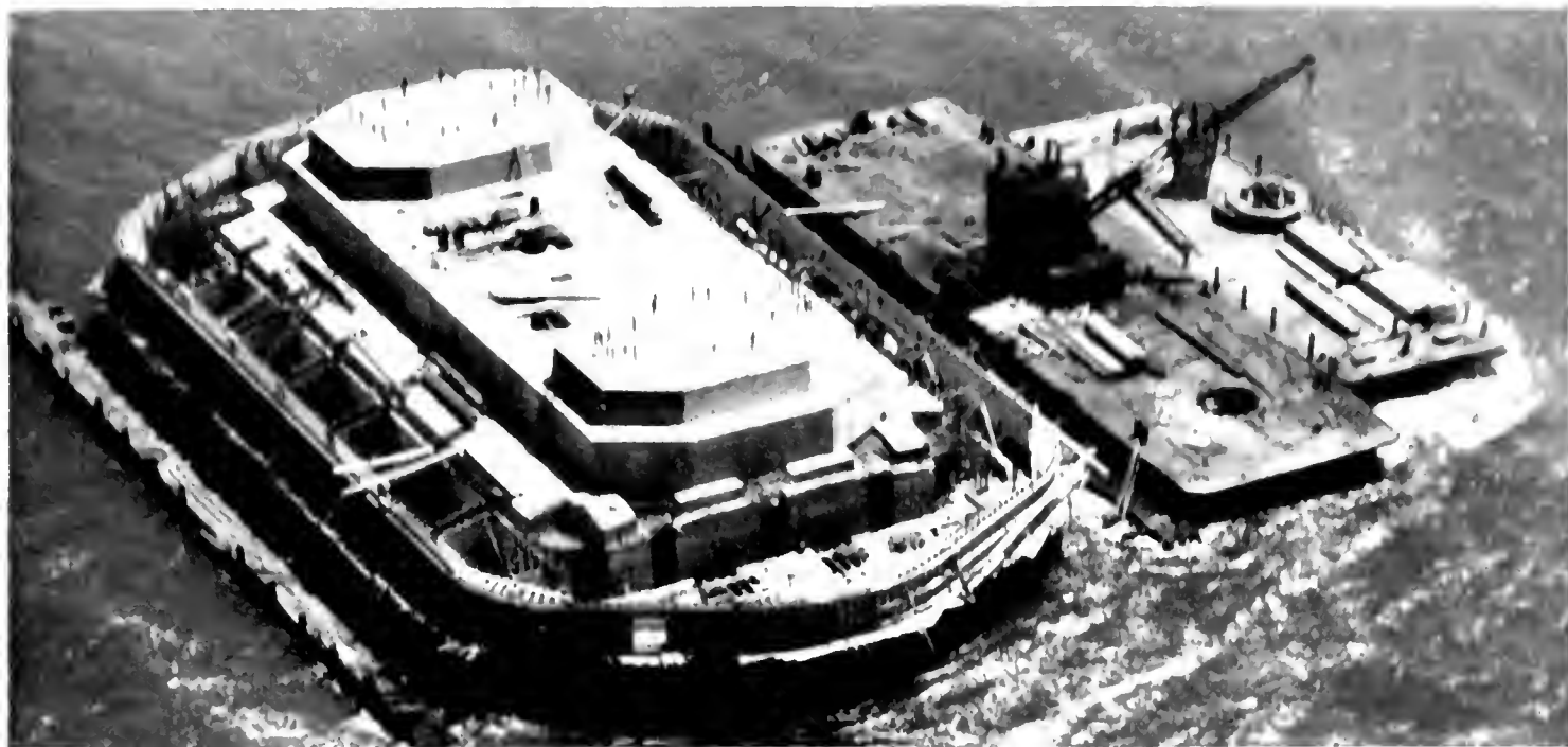
ANOTHER WORLD'S RECORD is represented by Pier W-6 of the Bay Bridge, located 1160 feet west of Yerba Buena Island; the first pier ever built and completed by the compressed-air-flotation caisson method.
