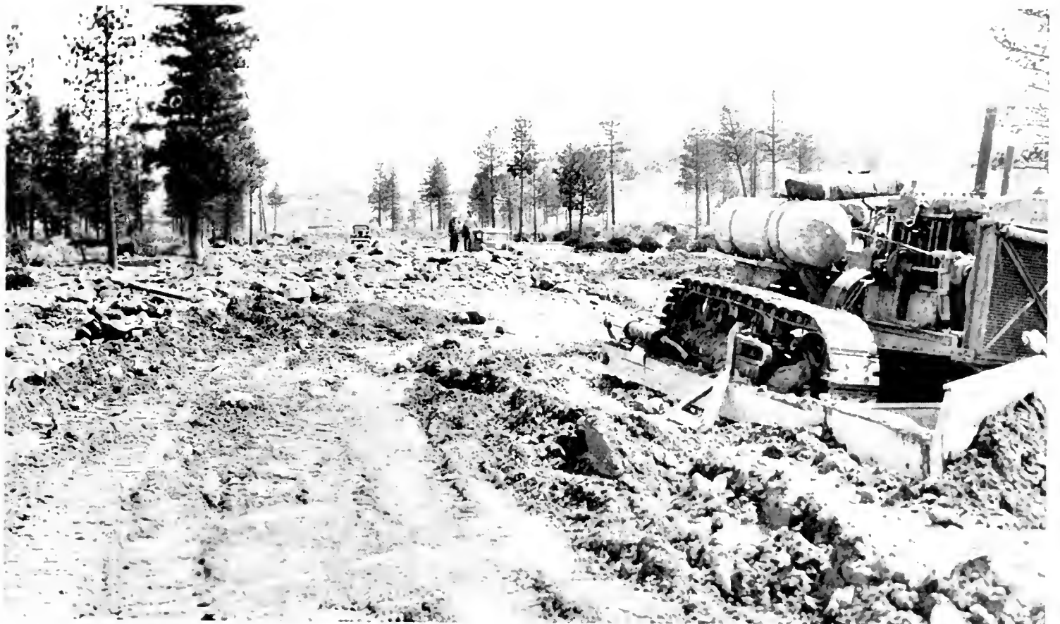
STATE HIGHWAY 72 BURIED under four feet of mud and boulders by flood waters from Mt. Shasta Glacier and Whitney Creek was cleared and opened to traffic in two days following the storm of August 28. The debris covered the road for a distance of 400 yards.
