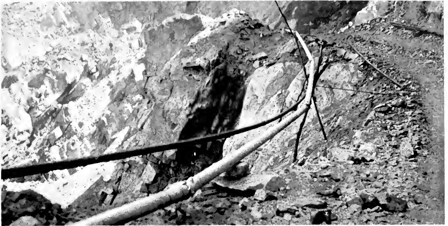
SPEEDY DRILLING is obtained on heavy rock work by the use of this light, large diameter, welded air pipe equipped with quick coupling device.
