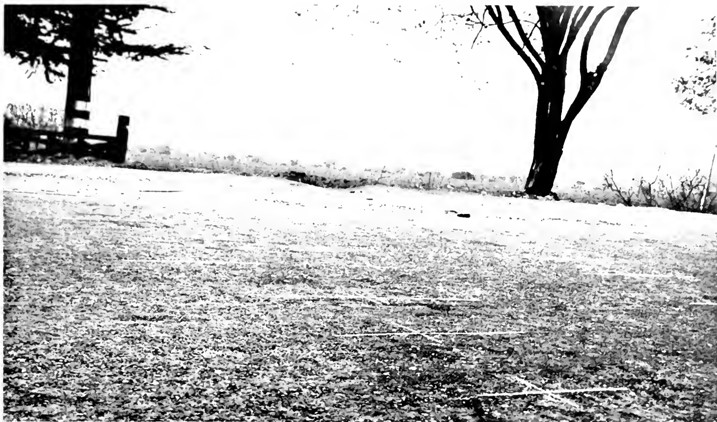
CROSSES MARK THE SPOTS where the "Roughograph" has detected high places in the newly laid asphalt concrete pavement which will be ironed out by cross-rolling.
