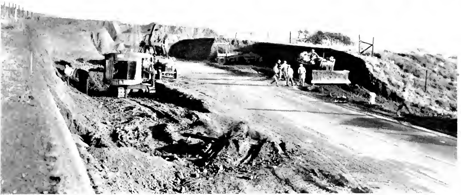
WIDENING THE COAST HIGHWAY between Santa Monica and Oxnard to meet traffic and safety requirements. At top—Grading to 80 foot width through scenic erosion area called the Little Grand Canyon. Below—Providing for addition of a fourth traffic lane on vertical curves where sight distance is short.
