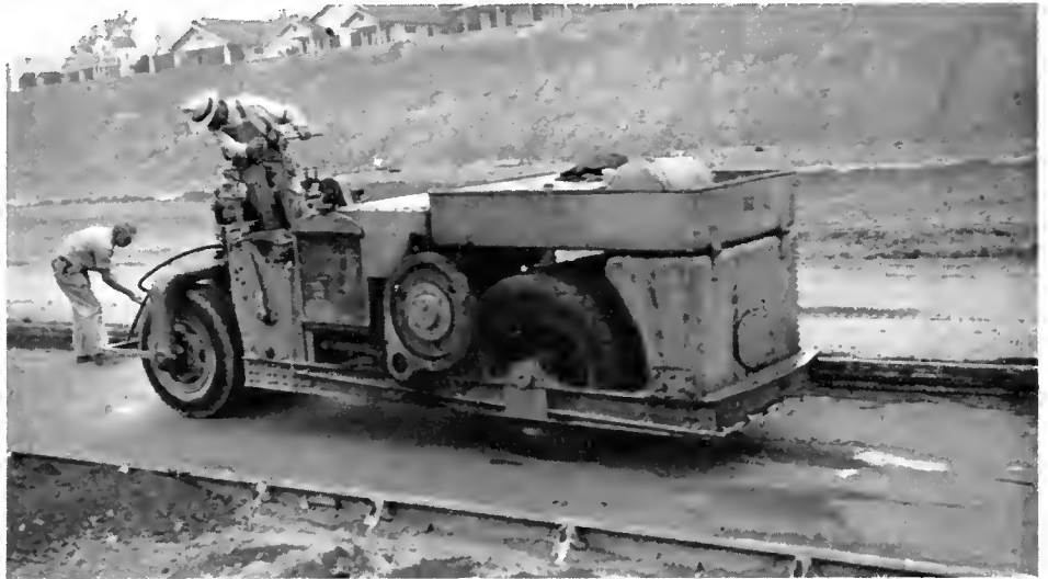
Rolling subgrade, after cutting to finish grade, with converted rubber-tired tandem roller
