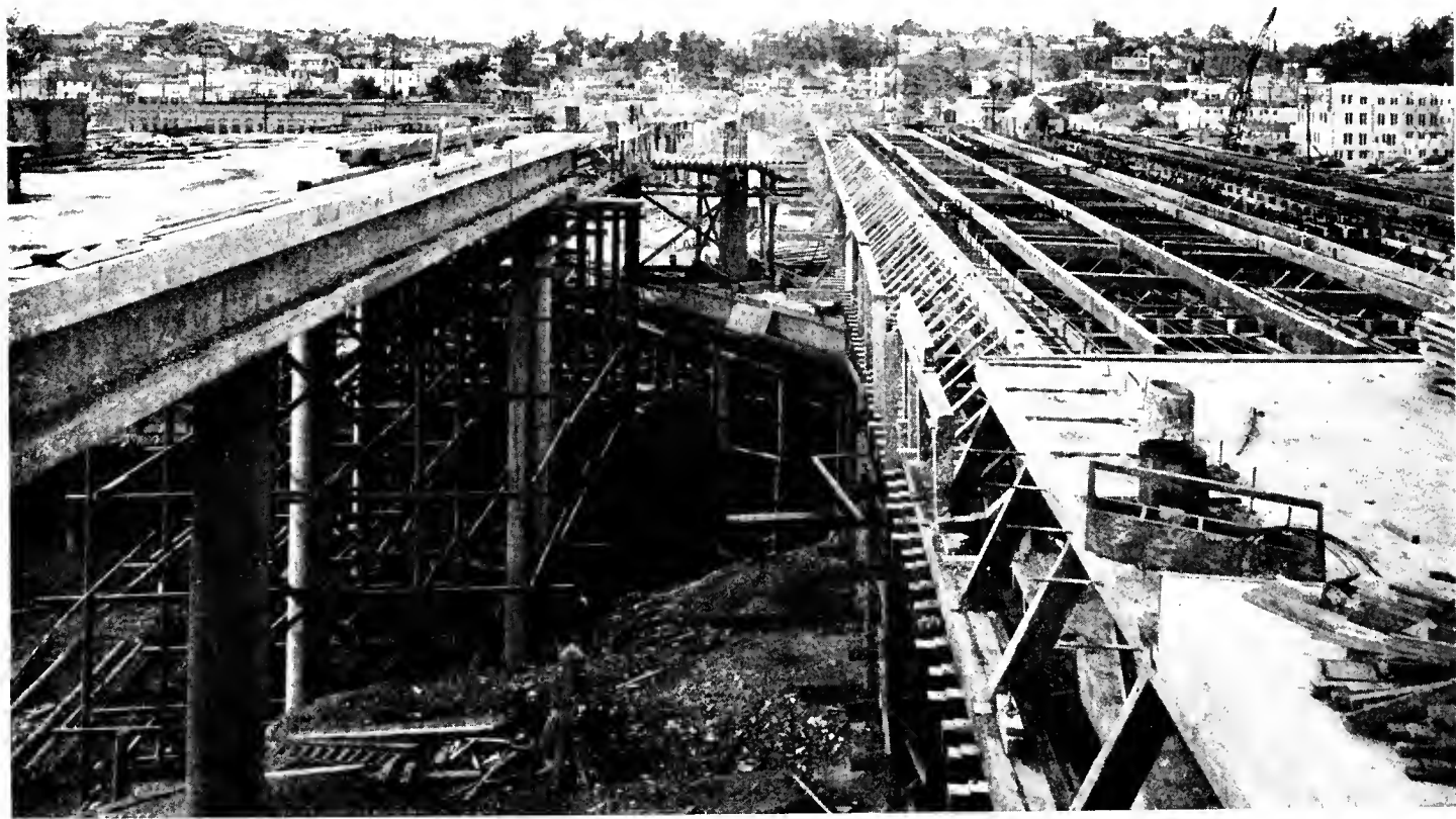
Upper—Figueroa Street undercrossing as viewed looking northwesterly with the Four-Level structure at left in the distance
