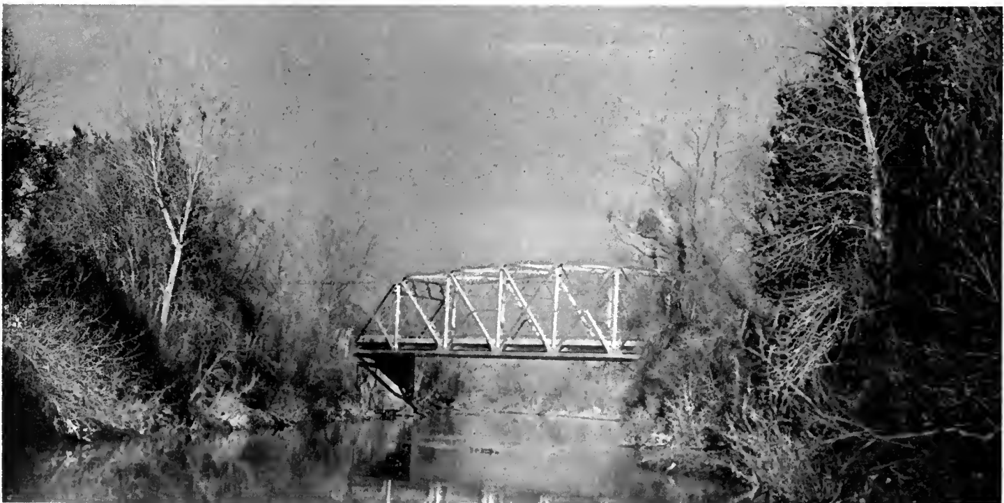
Span of new Mokelumne River bridge. This view is looking northwest and down the stream
