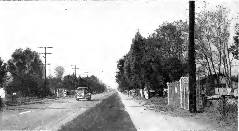
UPPER—Once a two-lane road between a railroad track and row of eucalyptus trees; now a four-lane divided highway. CENTER—Etiwanda Avenue now under construction. Foundation material in place. LOWER—Mail boxes attest to rural character of East Fifth Street
