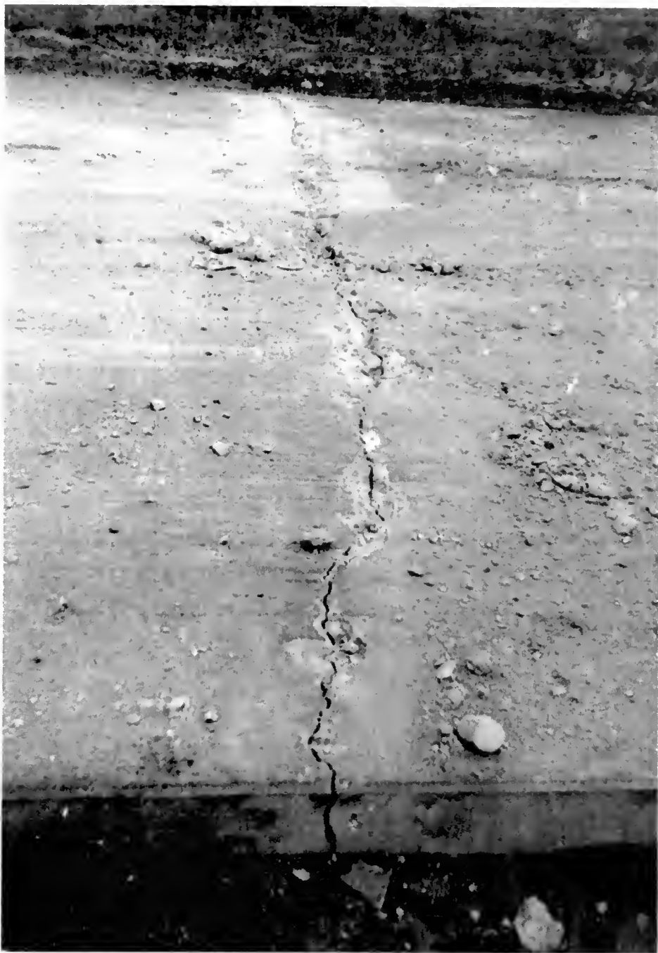
This photograph shows one of several similar cracks that developed between 80 and 300 feet from an unrestrained end of a long unreinforced concrete pavement. No expansion joints were provided
