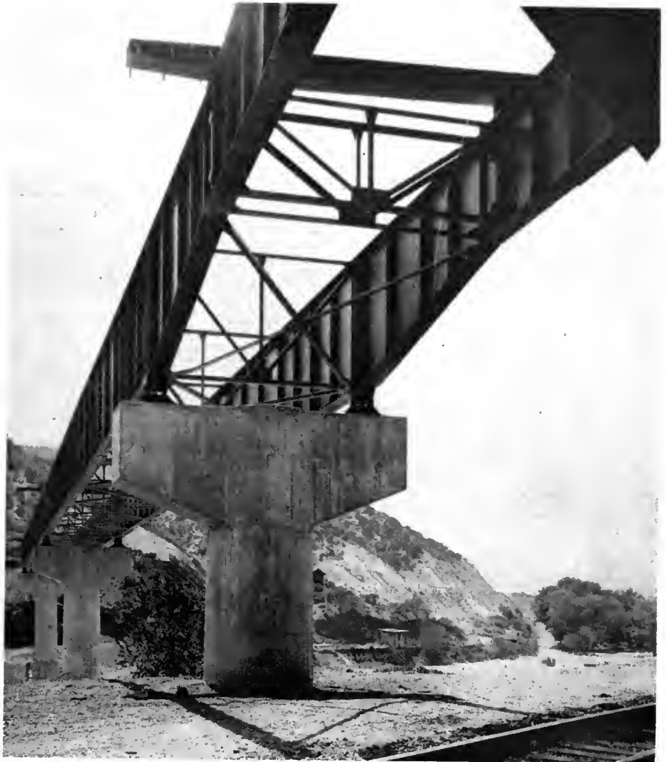
This photo shows close up of single leg cylindrical piers used in construction of Santa Clara River bridge
