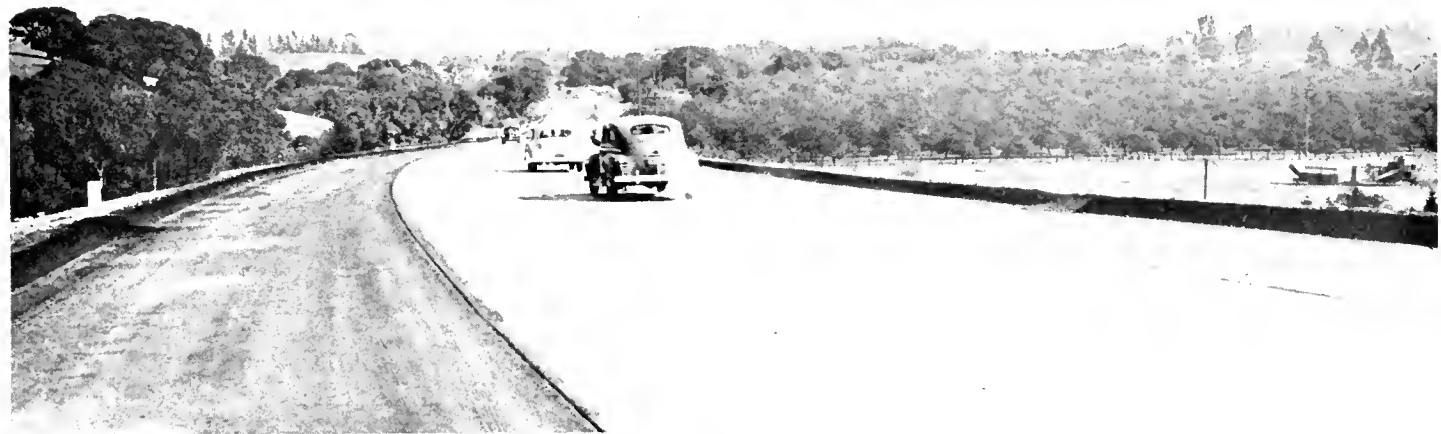
Sections of completed Crow Canyon Road. The center photo is a view of summit cut, where slides develop
