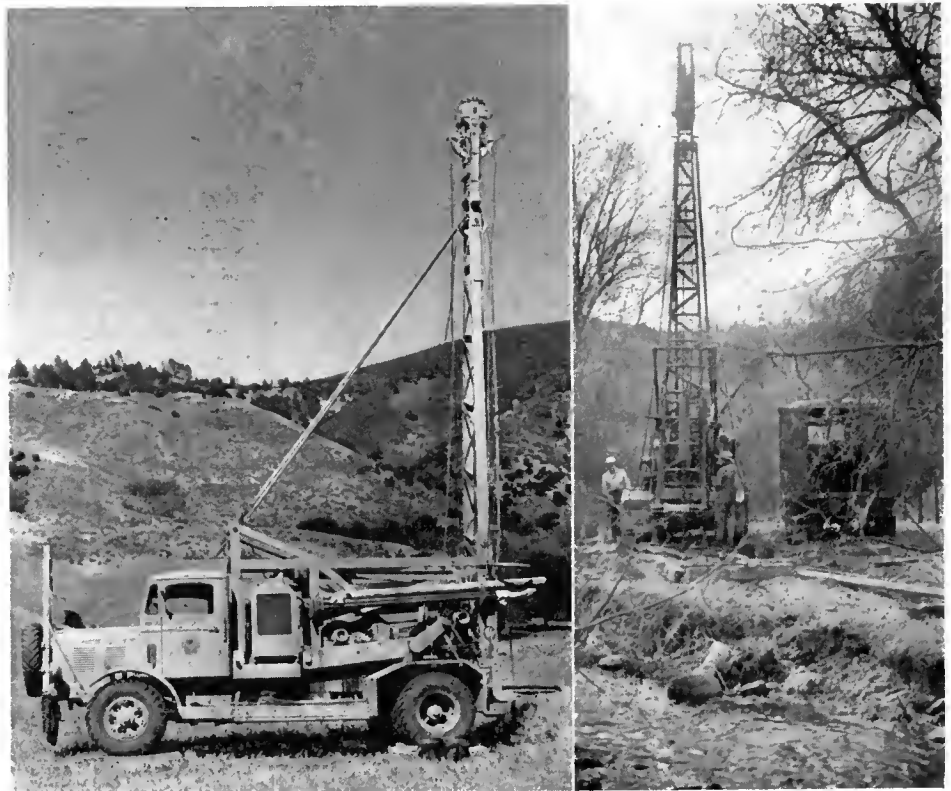
Left—Views of combination drillrig during exploration of foundation for proposed heavy embankment. As a result of an adequate preliminary investigation the unstable nature of the foundation was revealed and embankment failure prevented by foundation stabilization with vertical sand drains and controlled rate of loading. Right—Drill rig making foundation borings for proposed 120-foot high embankment
