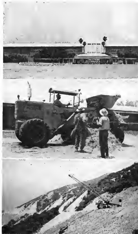
Upper—Race track. Center—Loading straw at stables. Lower—Rolling first application of straw with truck crane and tamping roller
