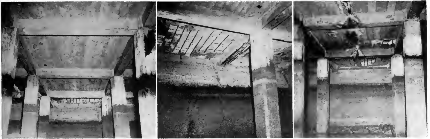
Figure 13. Showing condition of 36-year-old concrete in piles, bulkhead and underside of floor of a portion of Pier 17, San Francisco Harbor, January 6, 1948. Concrete in excellent condition throughout except where affected by rusting of steel reinforcement as shown which resulted from alternate wetting and drying due to splash of water against the concrete bulkhead at the shore end of the pier. Picture taken at low tide. Average tidal range approximately six feet.
