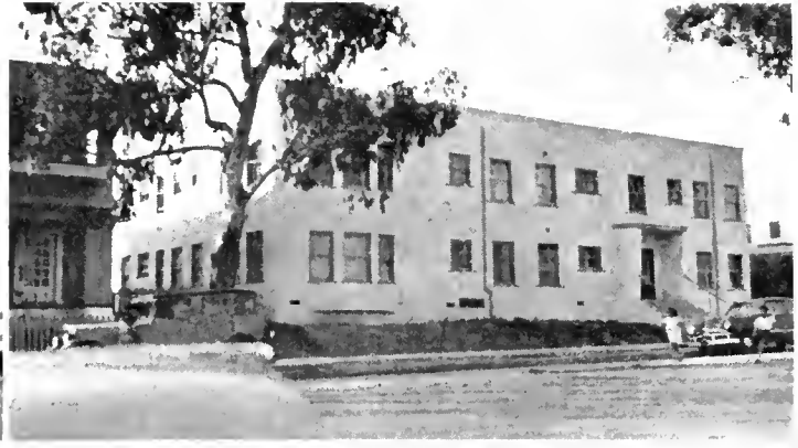
AFTER —This is the same building as it looks today, located at 209 North Boylston Street outside of the freeway limits. The stores were removed from underneath, the two upper stories were cut vertically into two sections and lowered to the ground.
