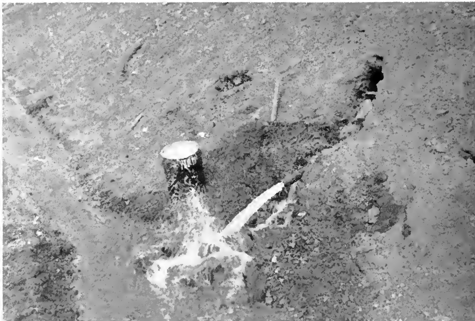
Flow from horizontal drain in Claverdale slide at rate of six thousand gallons per hour
