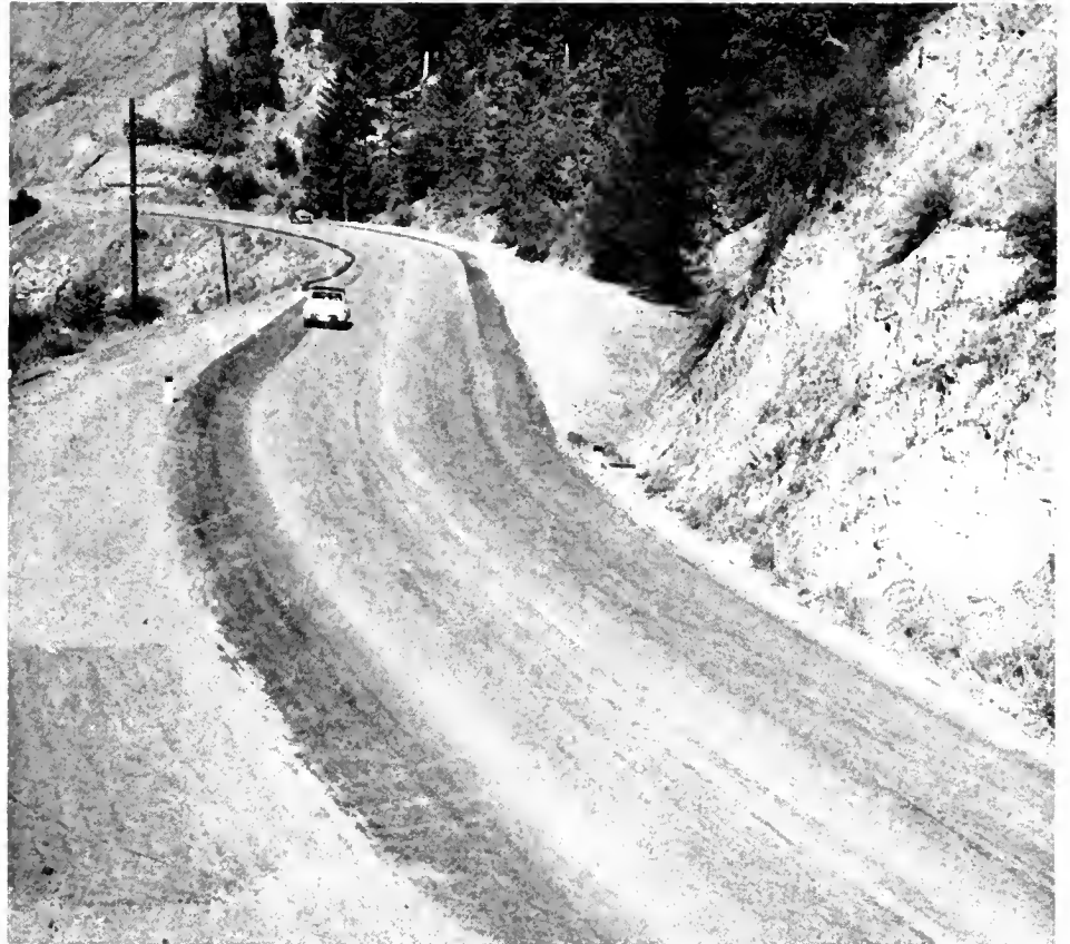
Upper—Wide roadway replaces former narrow road through unstable area. Lower—Easy curves along Eel River replace former winding road
