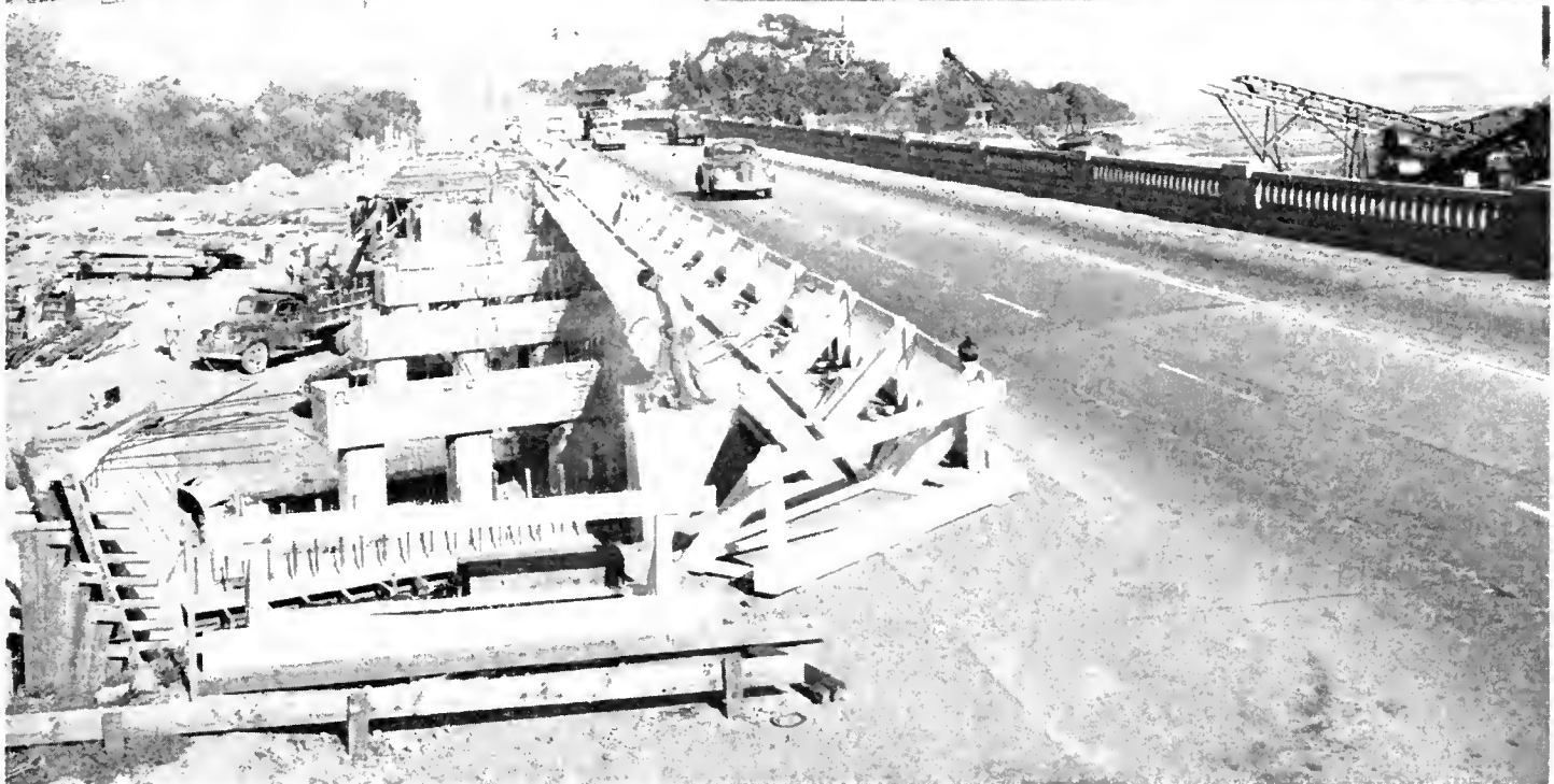
Upper—Showing oil treatment of portion of sandy slope where widening was carried out along high cut bank easterly of Malibu Creek. The dark portion of the cut slope indicates the portion that has been oil treated. Lower—Looking easterly along the Coast Highway, showing widening operations under way on Malibu Creek Bridge
