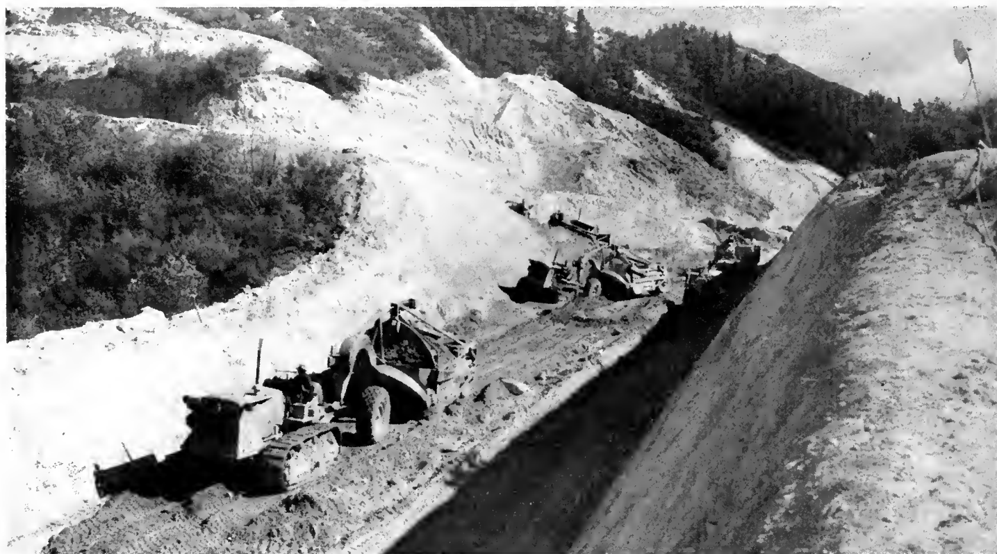
Typical view of grading operations on the Second Unit of the City Creek Road now under construction in San Bernardino County
