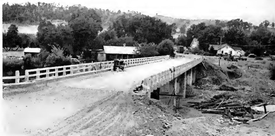
UPPER—Reeds Creek Bridge. CENTER—Paynes Creek Bridge. LOWER—Thomes Creek Bridge at Paskenta, showing wreckage of old span on right
