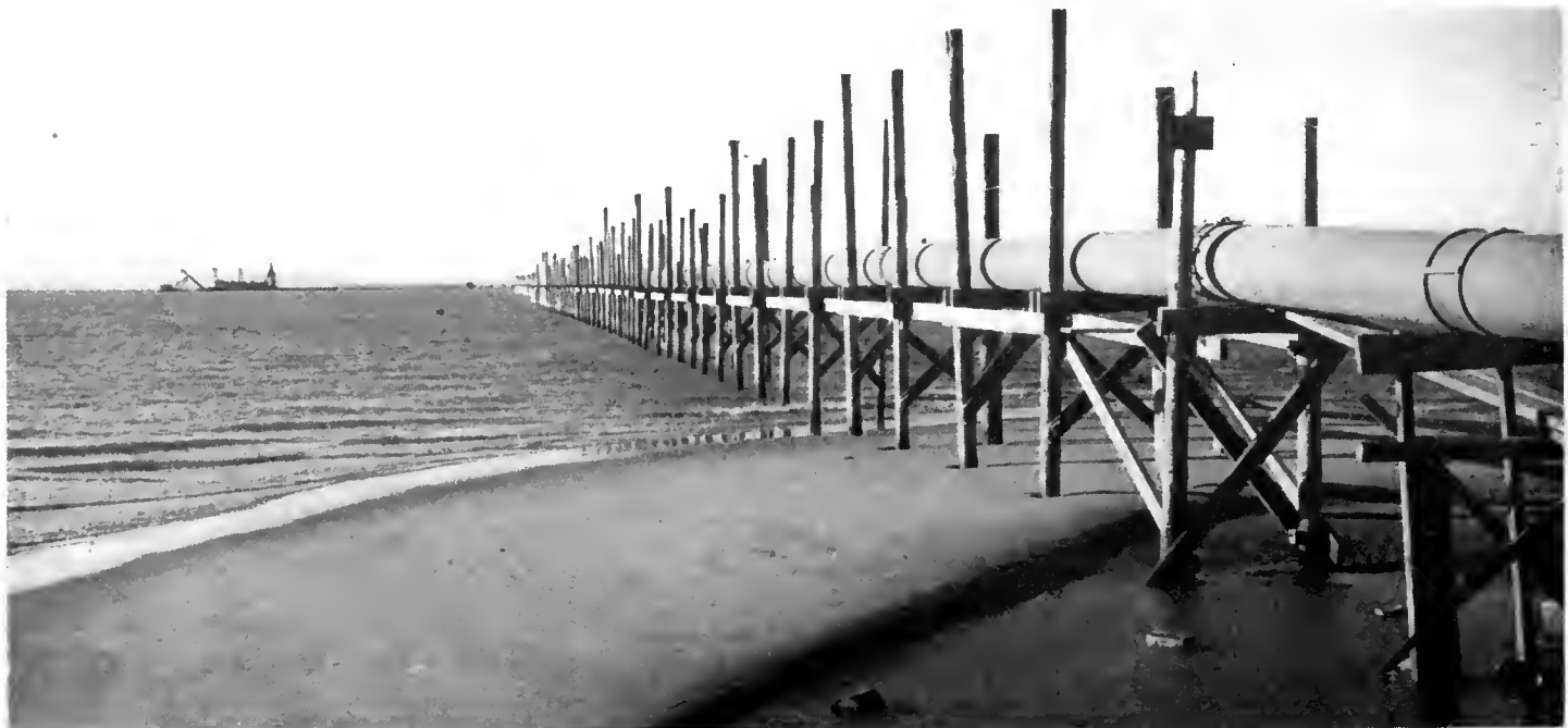
Levee on Bay Farm Island, looking west and showing trestle for dredger pipe. Suction dredge and floating line in background.
