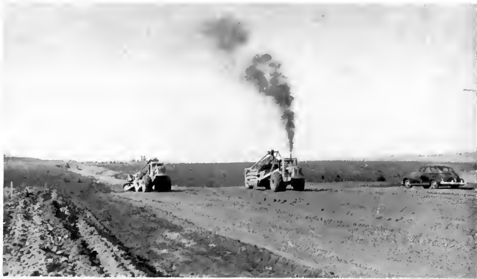
Modern earth moving equipment—tornapuls in foreground—power shovel and trucks in background. Free operators and inmate labor are working on this project in Modoc County in 1949
