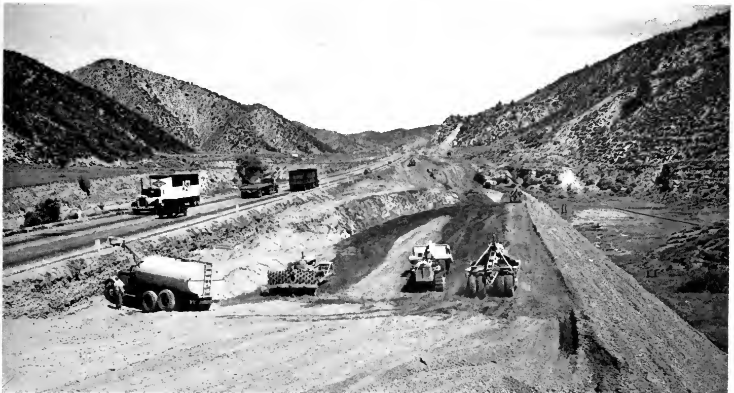
Portion of Ridge Route near northerly end, showing grading operations in progress. Existing 30-foot pavement now used for two-way traffic will become one-way roadway for southbound traffic after the new roadway for northbound traffic is completed
