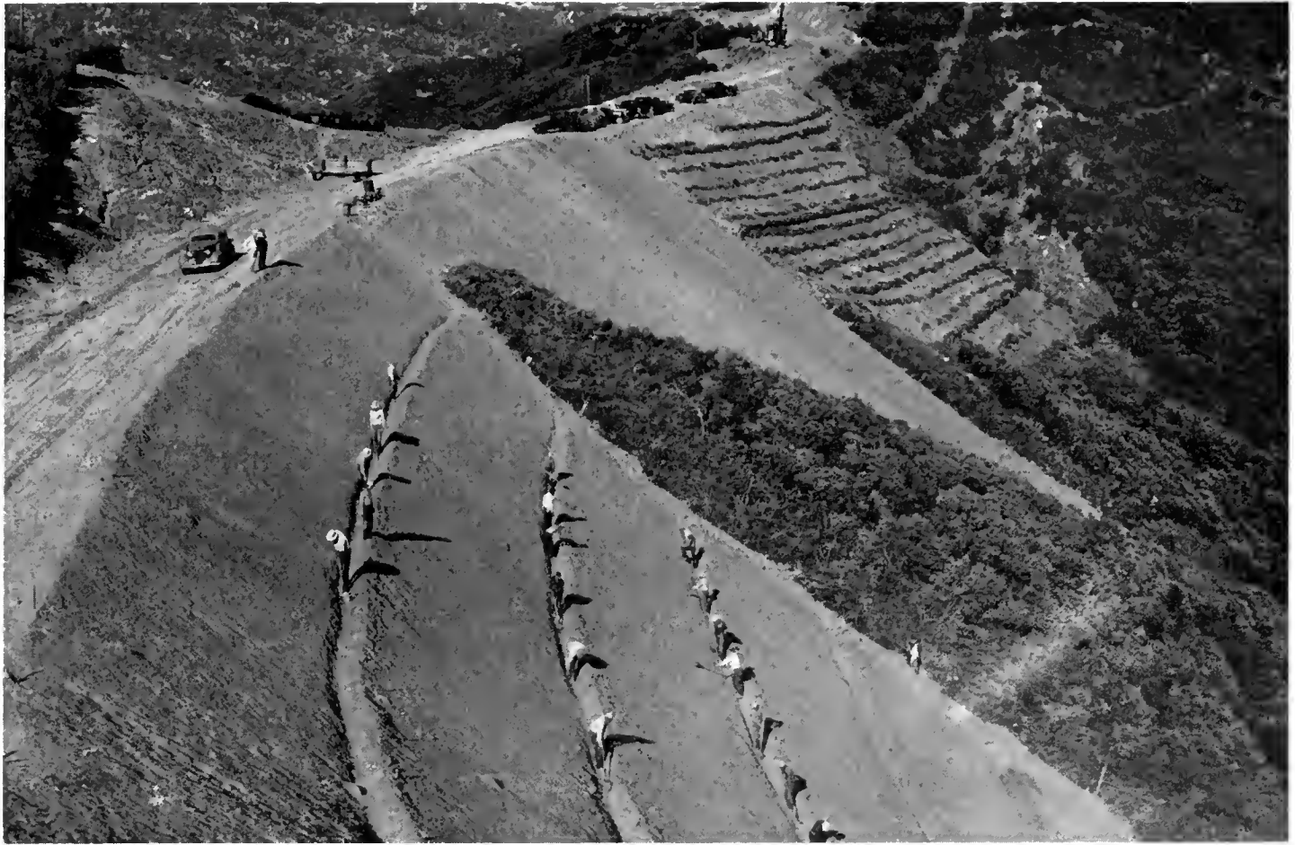
Erosion control with prison labor on Angeles Crest Highway, Los Angeles County, in 1938. Finished work is shown in background
