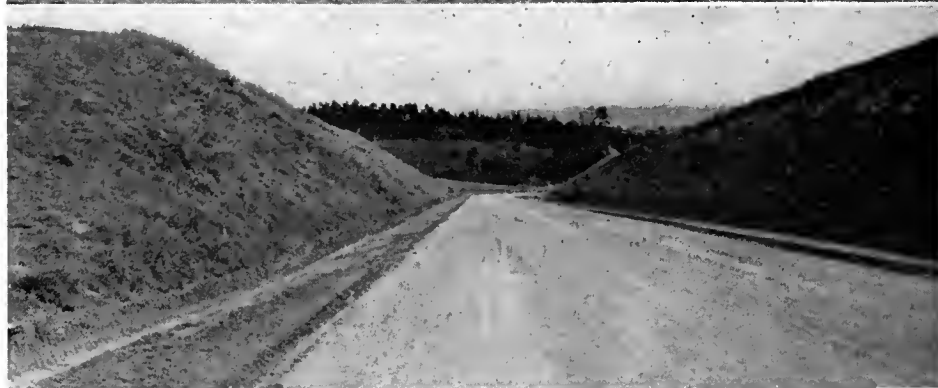
UPPER—Erosion caused by high-intensity storm during construction on untreated cut slope near Watsonville. Topsoil windrowed of top of slope. LOWER—Successfully stabilized cut slopes, same soil and locality as above, as they appear one year later. Treatment consisted of topsoil, straw and seed
