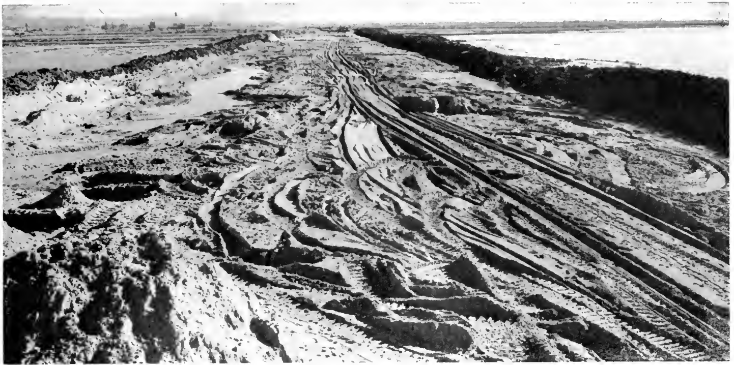
Damon Slough, looking south, showing completion of first link of hydraulic fill.
