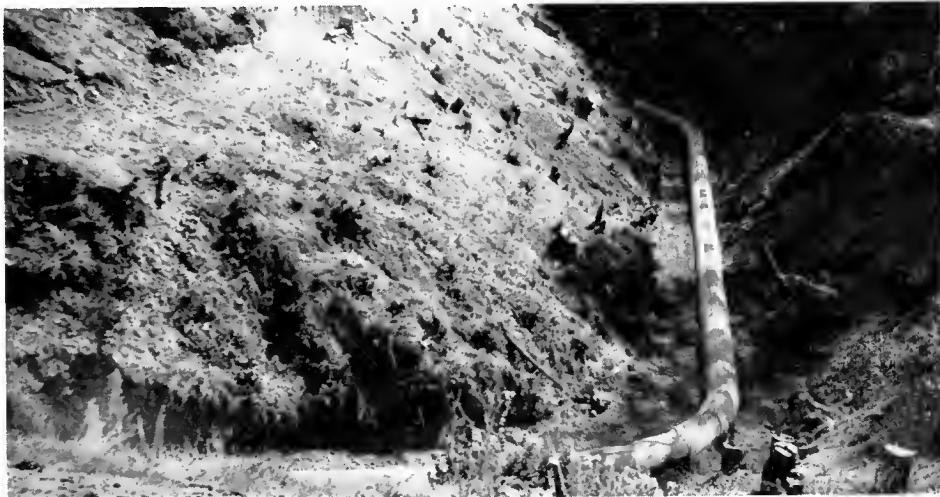
R. C. Arch culvert 462 feet long under 70,000 cubic yard embankment. Depth and winding alignment of creek prevented obtaining picture of entire installation in one photograph
