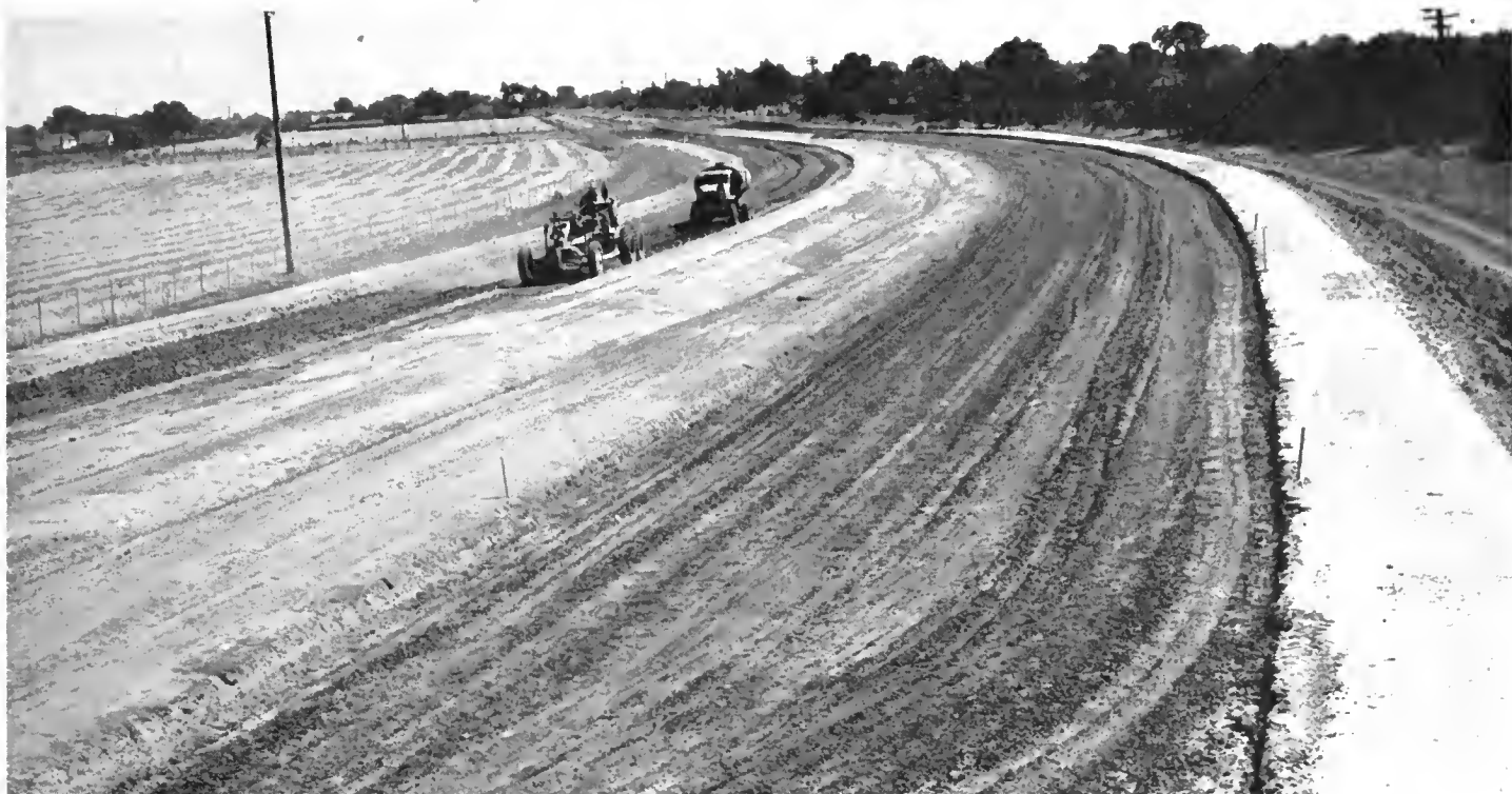
Grading for realignment of US 99, which will enable traffic to bypass Stockton and congested business section of city
