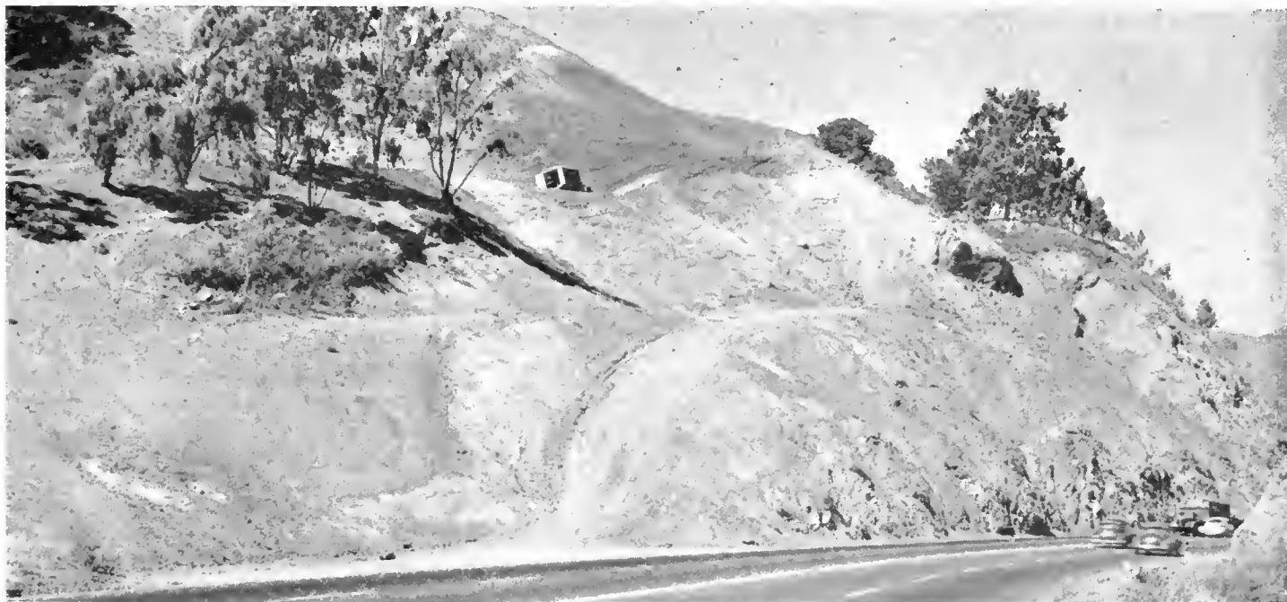
View of a large cut after unloading of slide and construction of flatter slopes with benches. Horizontal drains are being installed to complete the stabilization treatment
