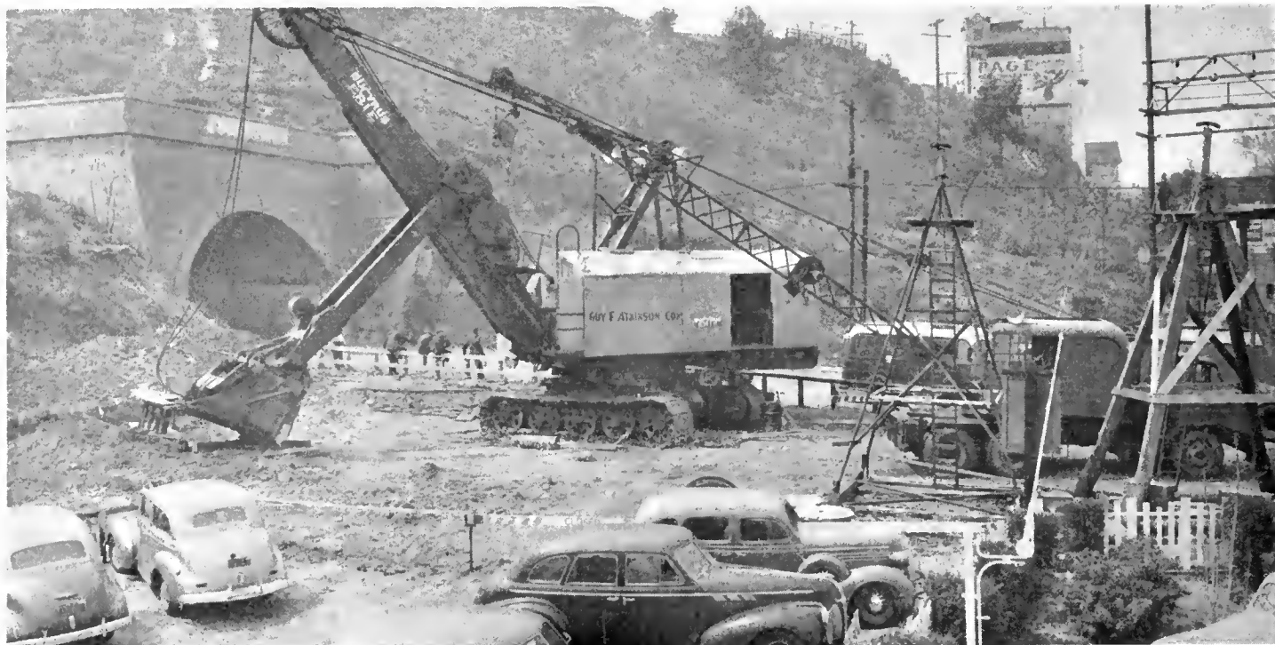
View of north portal of Broadway Tunnel before start of excavation operations. The contractor's shovel is an electrically operated rig weighing 185 tons, supplied with a 2300-volt current. Capacity of the dipper is six cubic yards
