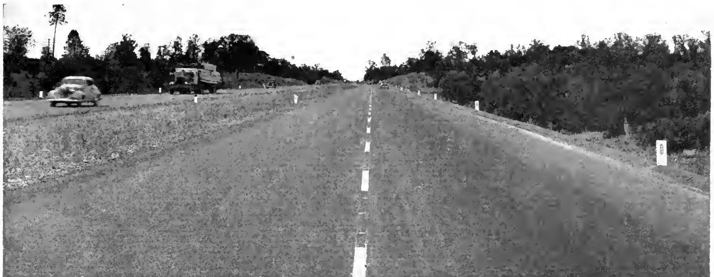
Plant-mixed, machine-shaped and finished drainage dike. Reflectorized guide posts outline road edge even in the fog
