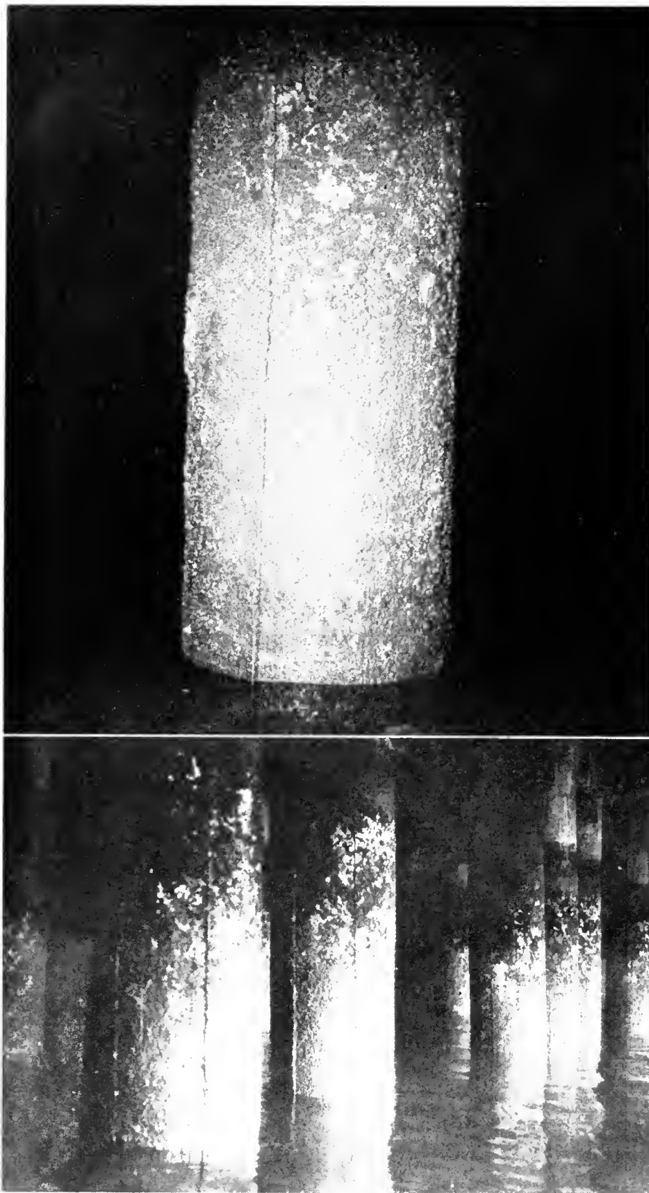
Figure 12. Showing condition of 36-year-old precast reinforced pile jackets. Pier 17, San Francisco Harbor, January 6, 1948. Constructed in 1912. Picture taken at low tide
