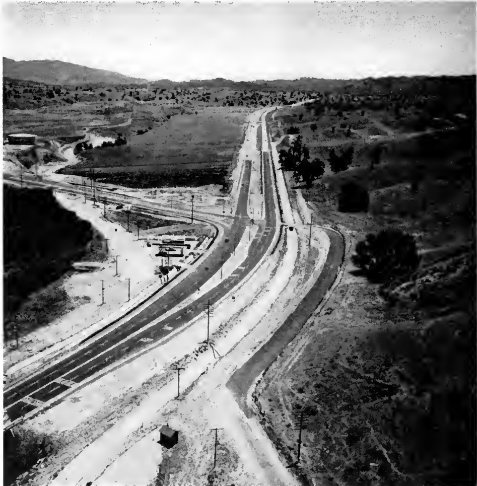
Completed section of Ridge Route looking southerly from the Santo Clara River crossing, showing channelized intersection with State Highway Route 79 to Sougus
