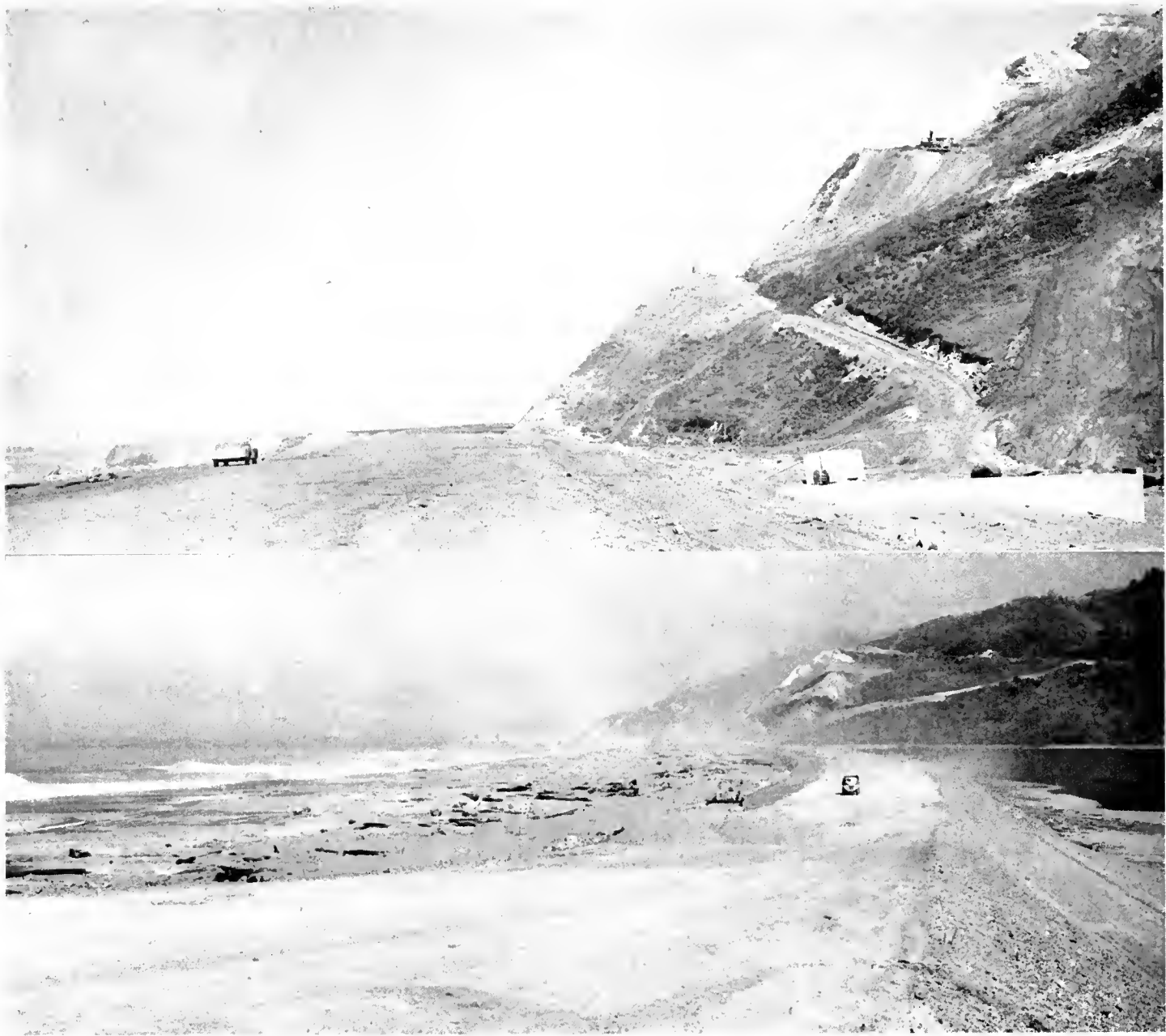
UPPER—View of completed 220-foot-high cut at Lookout Point near the north end of the project. This point was the location of the ancient Indian burial ground unearthed during construction operations. In the foreground is the equalizer culvert to control the water elevation in Freshwater Lagoon to the right. LOWER—View of new location along the sand spit with Freshwater Lagoon on right and Pacific Ocean on left. In the far distance is Lookout Point. The old highway can be seen at upper right
