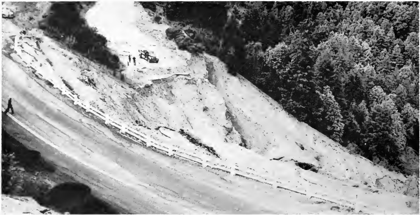
Large fill slipout was later corrected by combination of stripping, rock drains, toe support fill and horizontal drains
