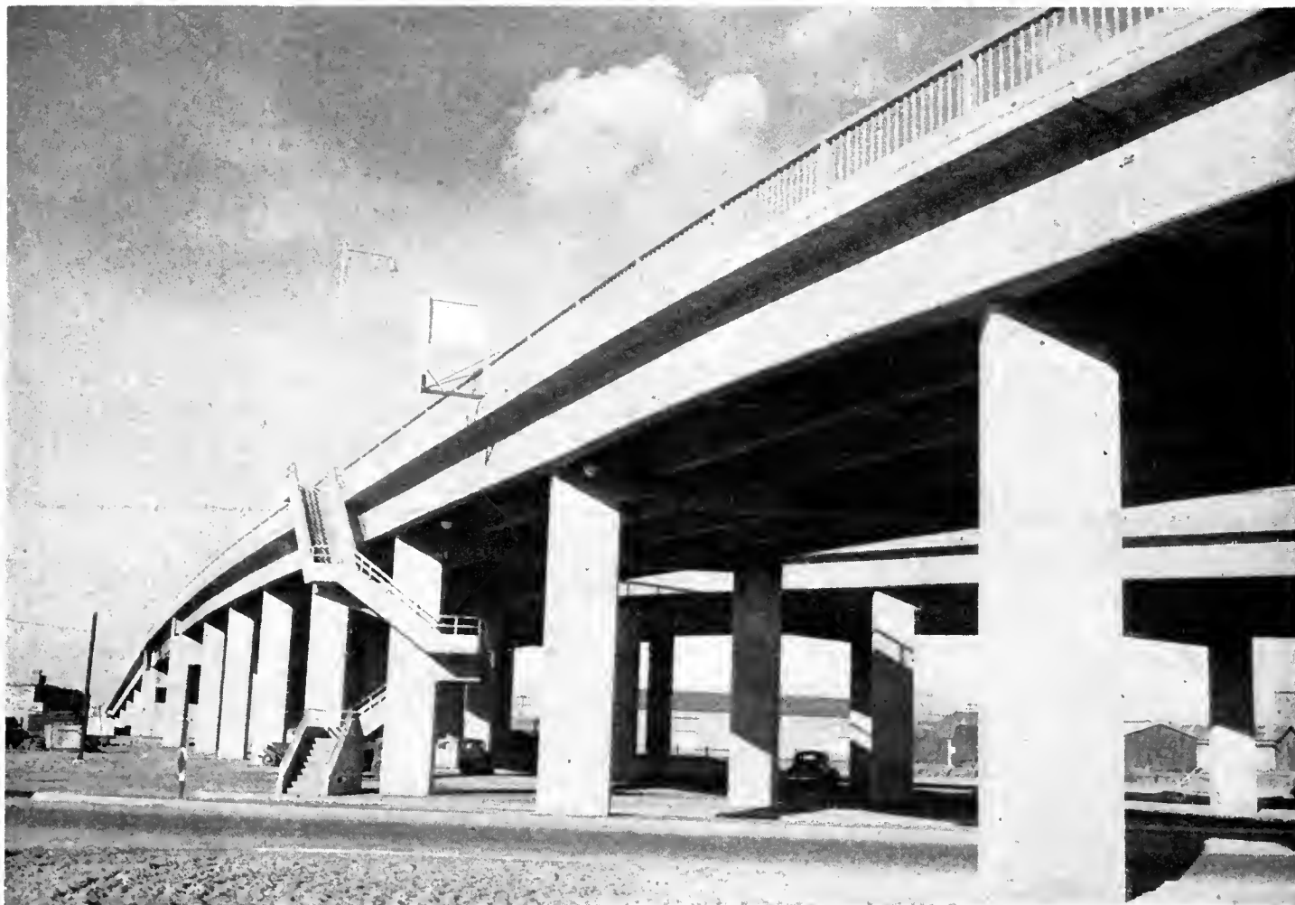
Intricate stairway construction at G Street crossing of southbound Monterey Street overpass structure
