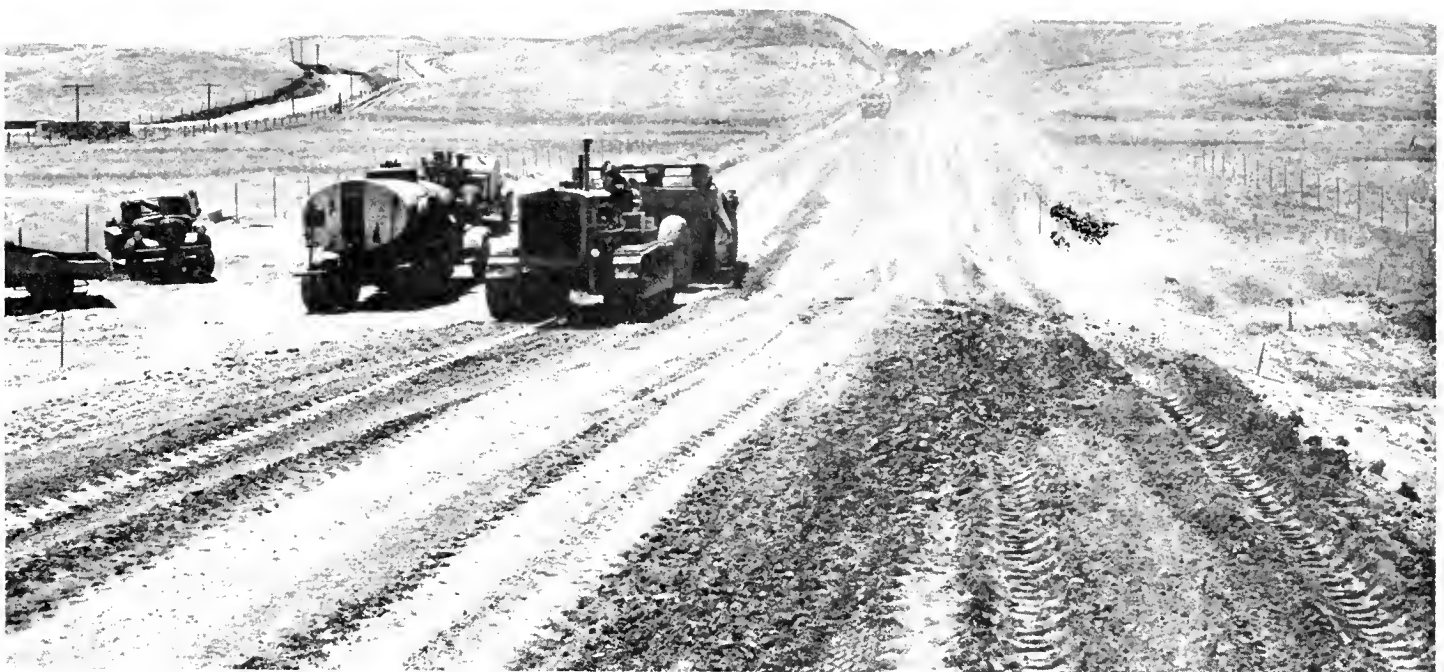
These two photographs show heavy equipment used in grading for the new Sacramento-Jackson Highway. Present winding road is shown at left of lower picture
