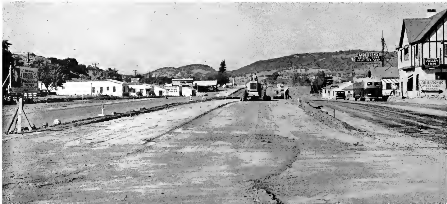
Looking northerly through Buellton, showing construction under way. All structures on right and left were moved back off the existing 60-foot right of way to provide a roadway width of 176 feet
