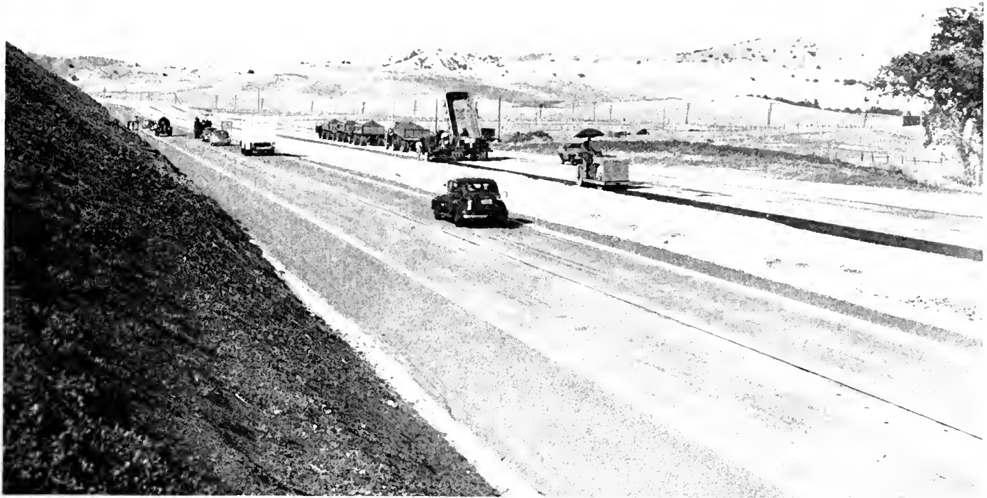
Fairfield By-pass under construction near the east end of project. Traffic is using southbound lane as a two-lane highway
