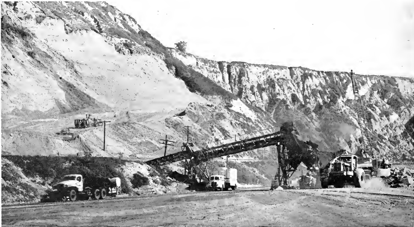
Borrow pit and belt conveyor at westerly end of project. Note that conveyor passes beneath railroad tracks through existing drainage culvert
