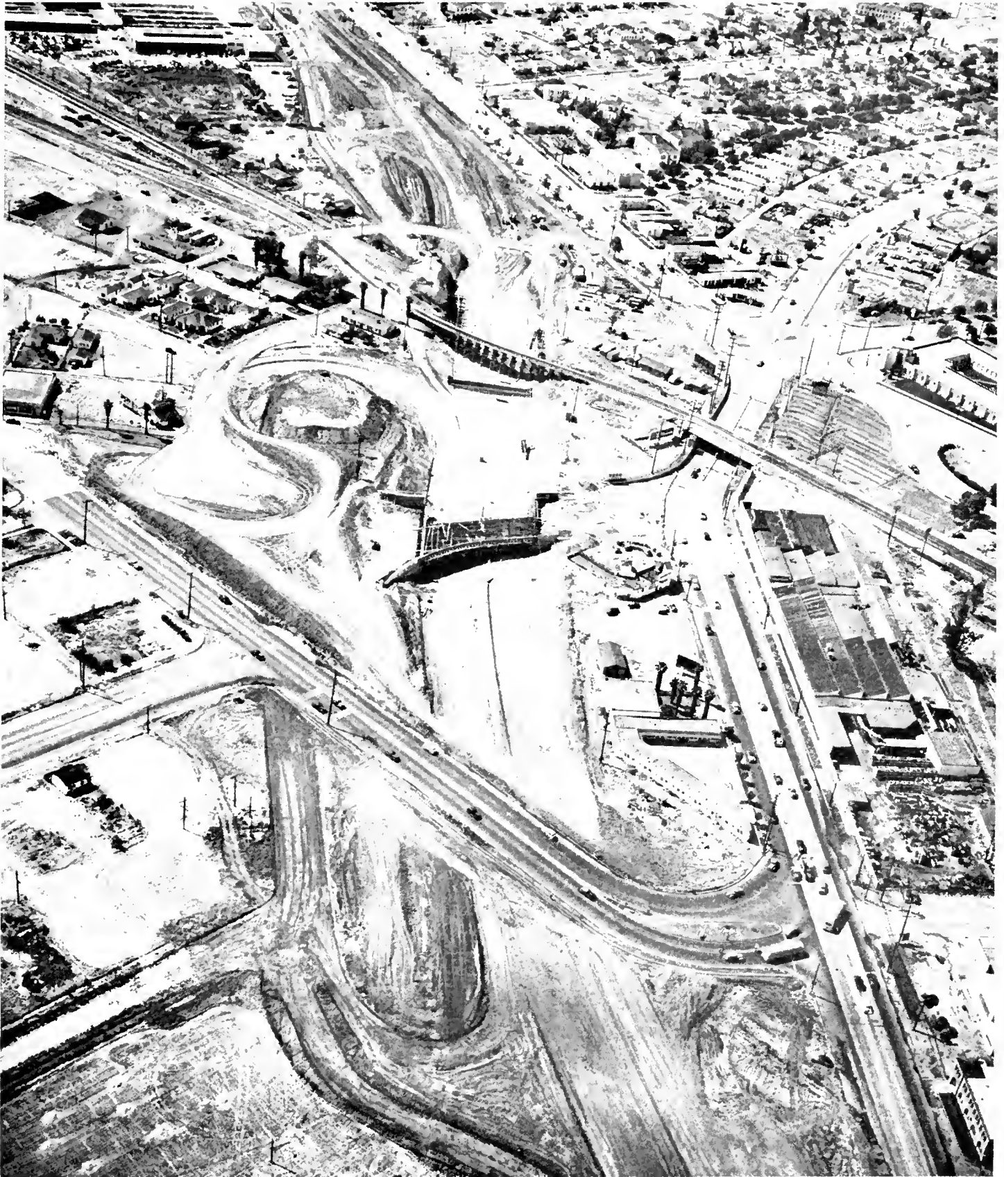
Aerial view of construction area on Santa Ana Parkway looking westerly. Atlantic Boulevard detour in foreground with new grade separation and Union Pacific Railroad shoofly trestle in center
