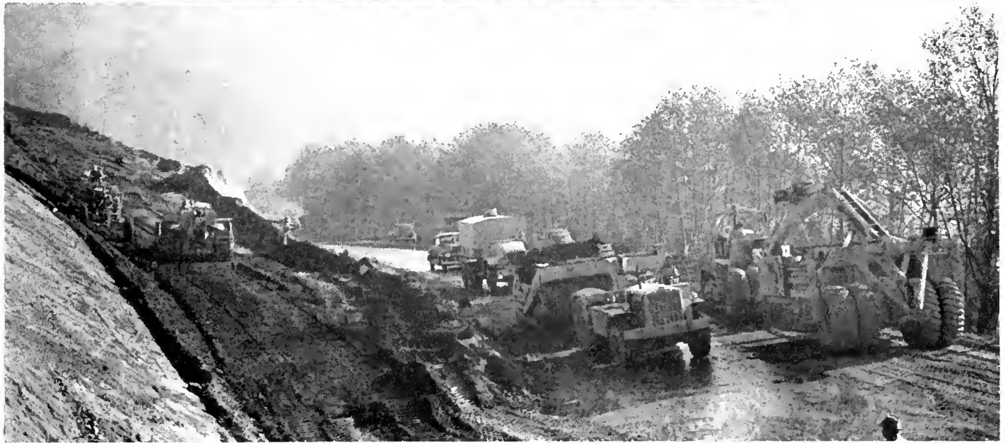
UPPER—Construction operations in progress just north of Stone Lagoon Summit. The new location through rugged country can be discerned in the distance descending to the sand spit, which can be seen at the extreme upper right edge of the photograph. LOWER—Grading operations at Stone Lagoon Summit at the south end of the project. The new location departs from the old highway at this point, the existing road being in the immediate foreground
