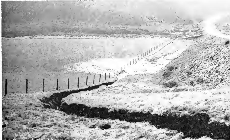
Adjacent property affected by debris from eroded highway drainage ditch. (On Coast Route, south of Half Moon Bay, San Mateo County)
