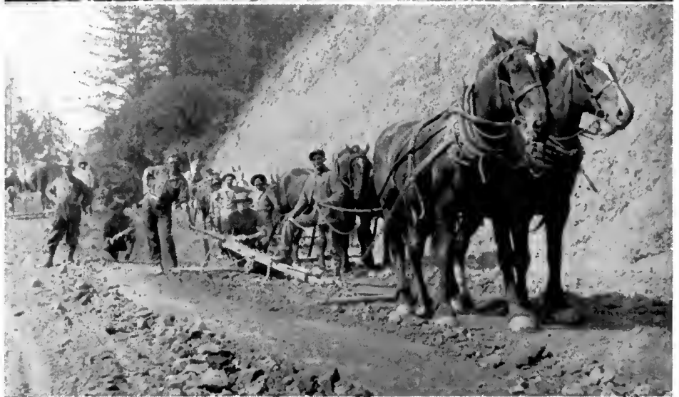
Hand labor methods of building highways in mountainous areas with inmate labor. UPPER—Track and dump car in Shasta County in 1916. LOWER—Teams, plows and Fresno scrapers along Smith River in Del Norte County in 1923
