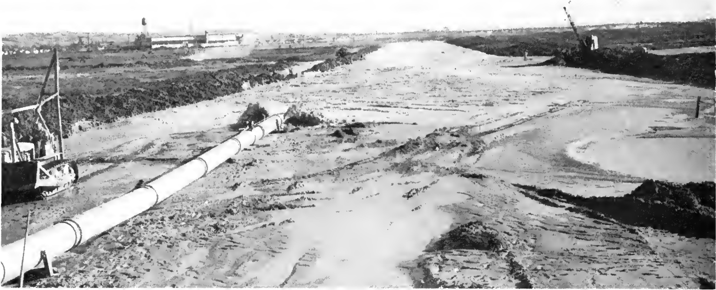
Elmhurst Creek, looking south and showing outlet of dredger pipe. Tractor on left used for moving and placing pipe and reinforcing levee.
