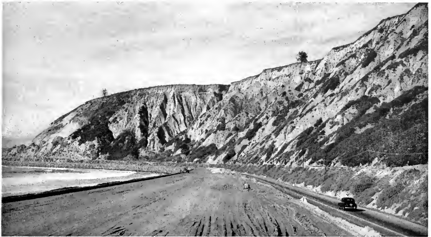
Northwesterly view showing left half of roadway to approximate final grade. Note riprap shore protection in left background
