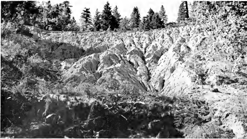
Roadway fill slope composed of disintegrated granite material after high-intensity rains. (Between Redding and Weaverville, Shasta County)
