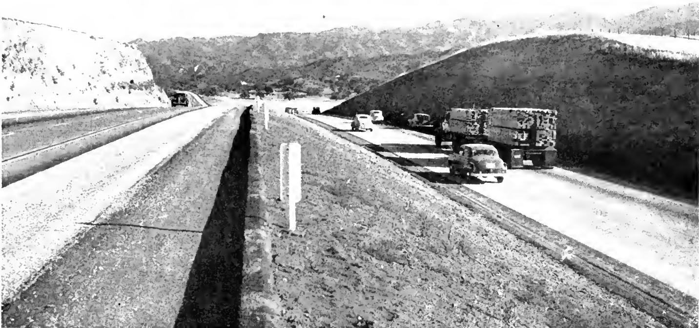
Upper—Completed section of Ridge Route north of Costaic. Lower—Completed section of Ridge Route between Santo Claro River and Pico Canyon, looking southerly, showing protection provided traffic where newly constructed pavement is lower in grade elevation than the existing pavement
