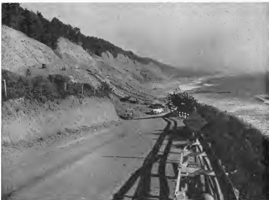
This photograph shows early stages of construction on Woddell Bluffs project as seen near the northerly end. Old road is on the left
