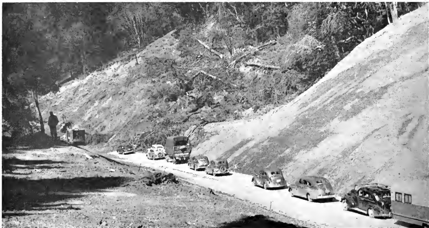
Road temporarily closed by slide occurring during construction. Subsequently flatter cut slopes with benches were constructed. Installation of horizontal drains is planned to complete the stabilization treatment
