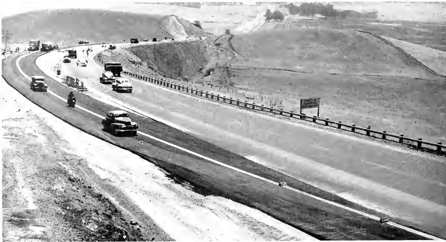
US 40 for a distance of 4.6 miles through the American Canyon is being widened to four-lane divided standards
