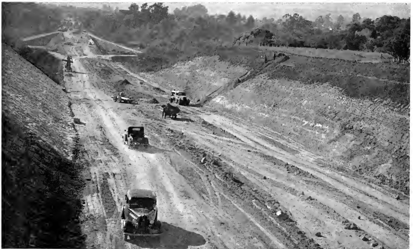
Deep excavation work in progress on new freeway near Soquel, looking toward Santa Cruz (see Page 10)
