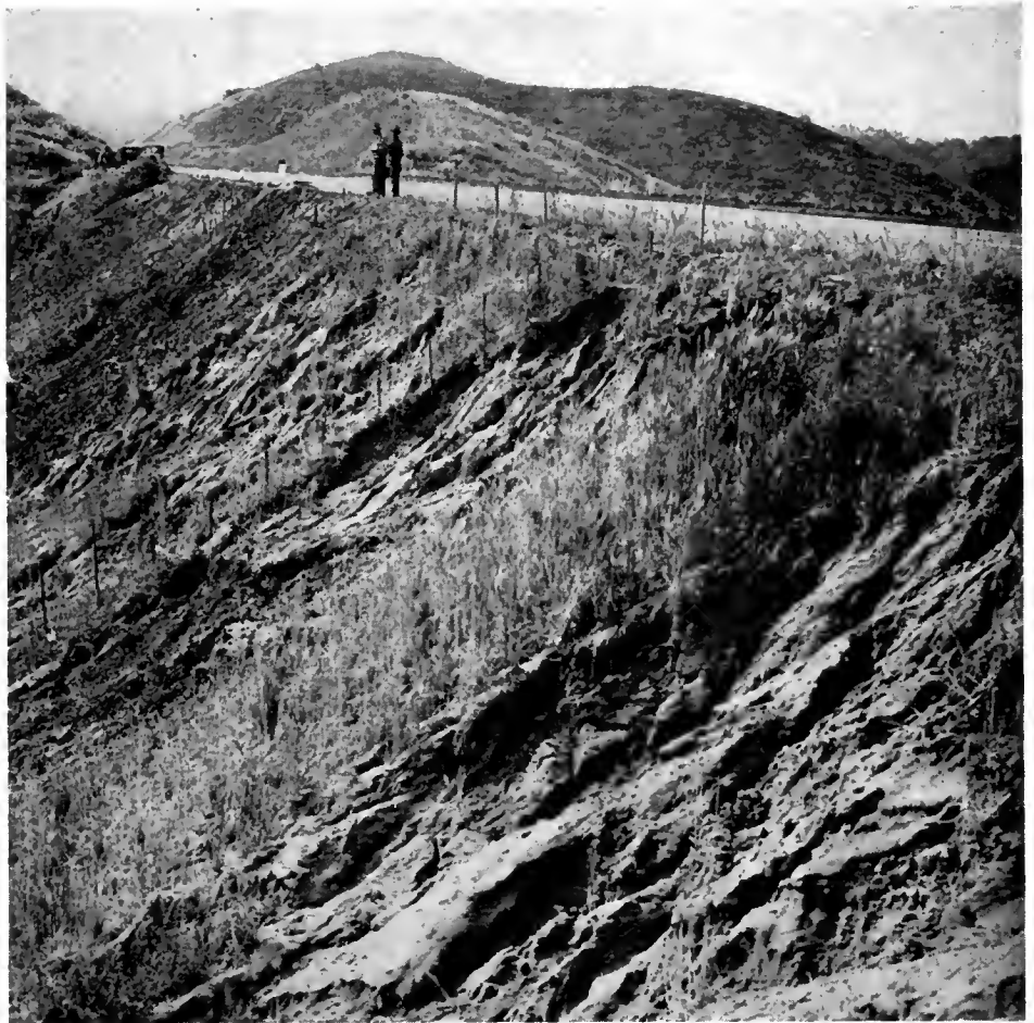
Damage on a 1½:1 fill slope seeded to borley. No straw mulch was used. The soil is of a sandy and highly erosive nature
