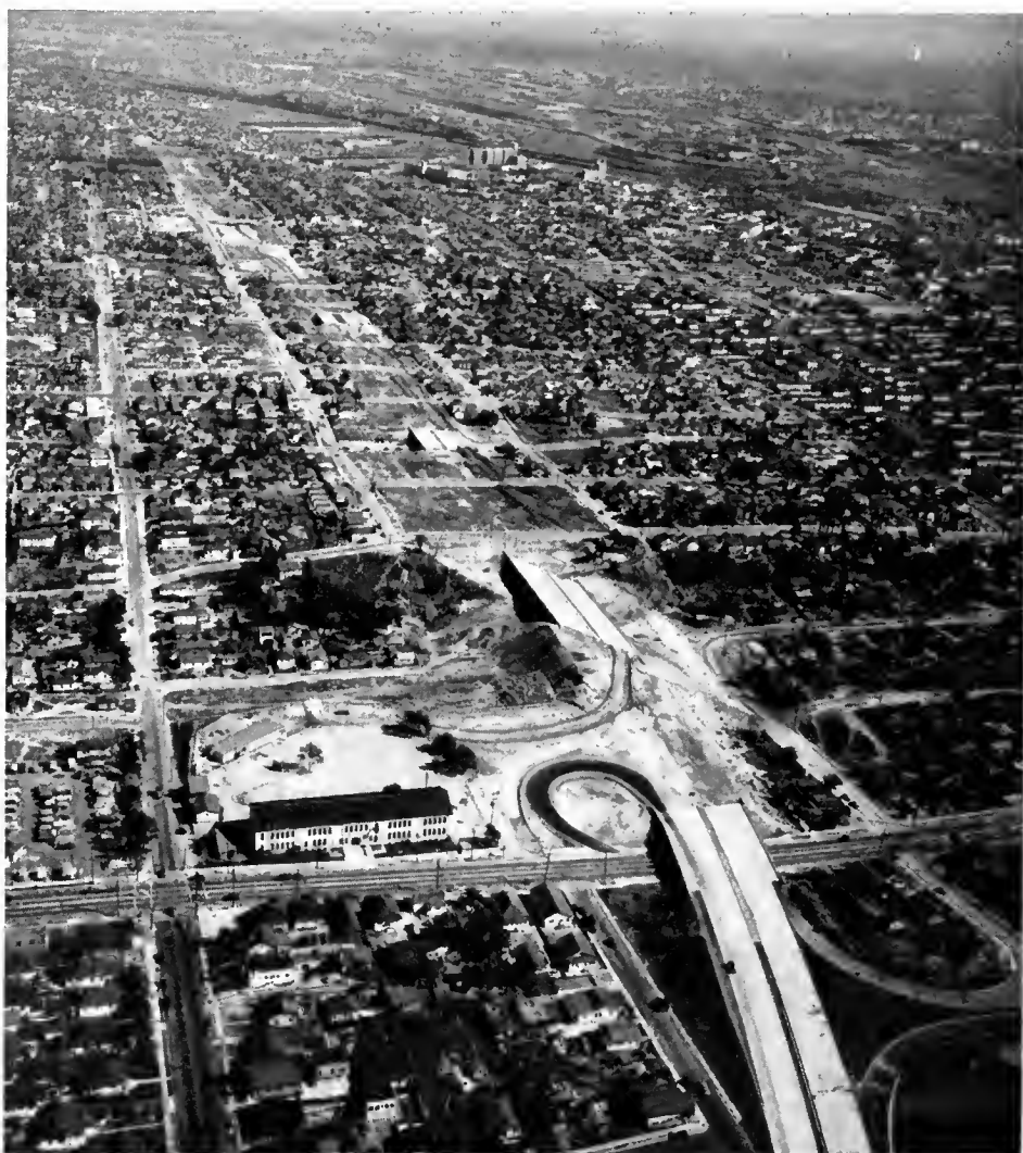
Aerial photograph looking easterly from completed section on Santa Ana Freeway at Soto Street to a point easterly at Eastern Avenue, showing completed freeway grade separation structures and right of way cleared ready for roadway construction. Approximately 90 percent of residential buildings in this area were moved to available vacant lots, rehabilitated, and are back in use housing families. Not a single tenant was evicted from a residential unit on the entire Santa Ana Freeway right of way clearance project from the Aliso Street viaduct at the northwesterly terminus of the completed section through the areas shown in this photograph.
