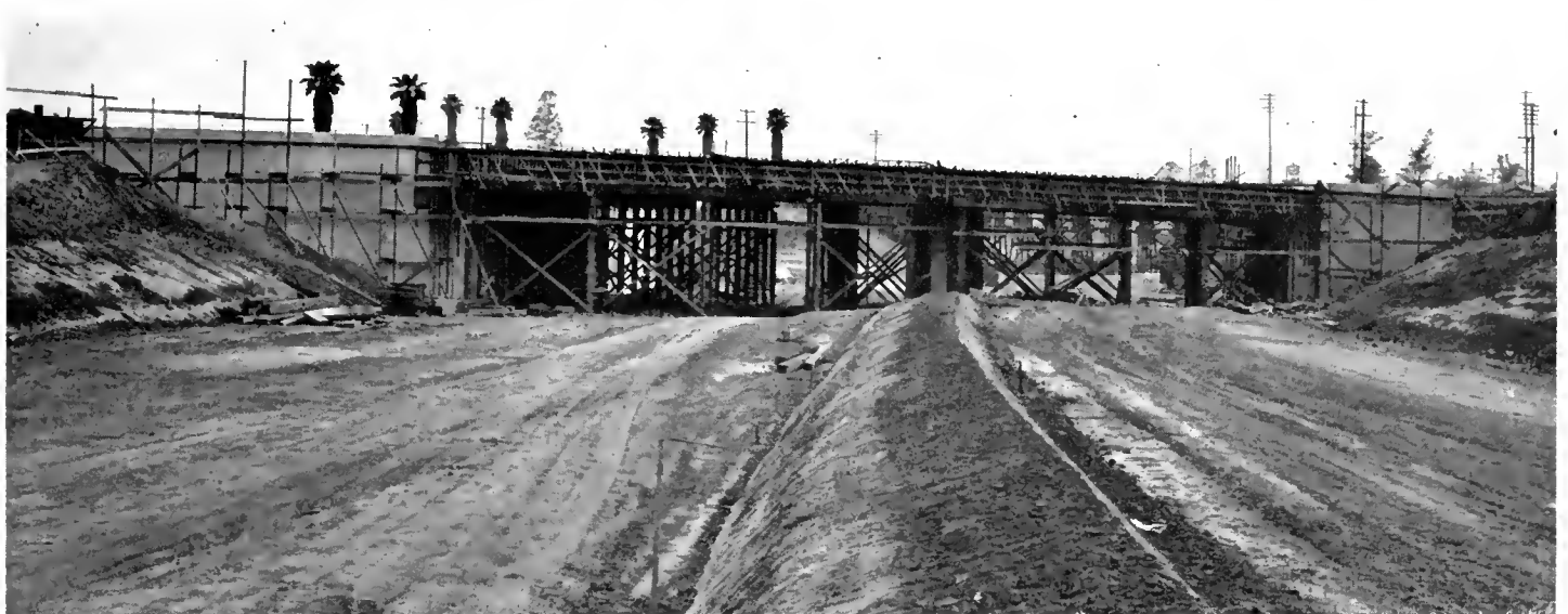
View looking southerly, showing construction in progress on Atlantic Boulevard grade separation bridge over Santa Ana Freeway
