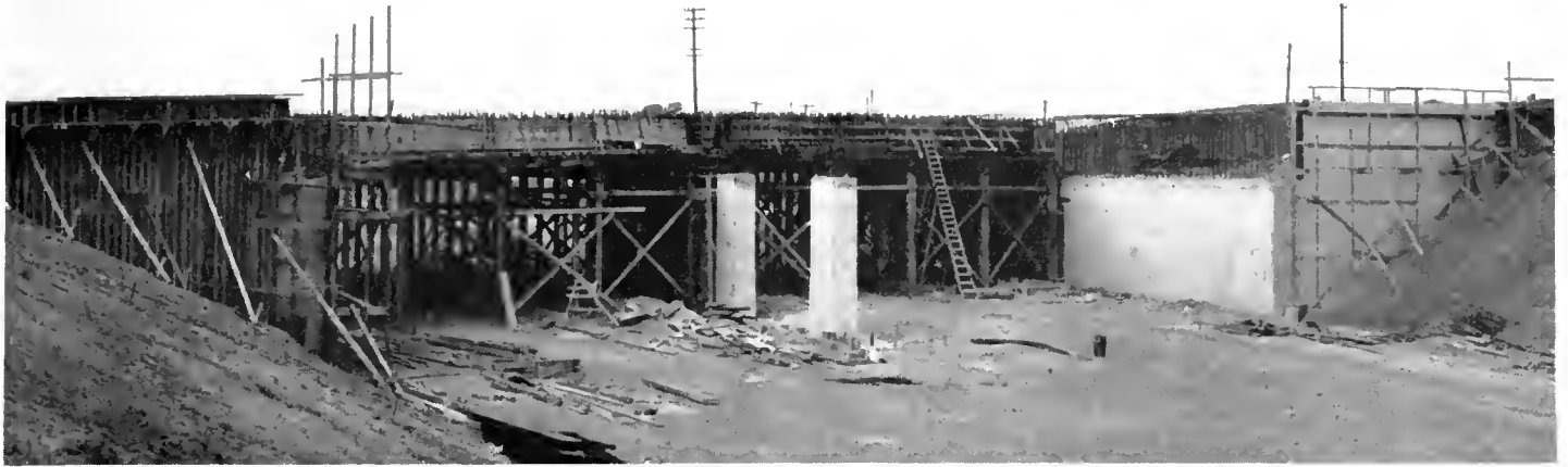
View westerly along Santa Ana Freeway showing construction in progress on the Atlantic Boulevard grade separation bridge
