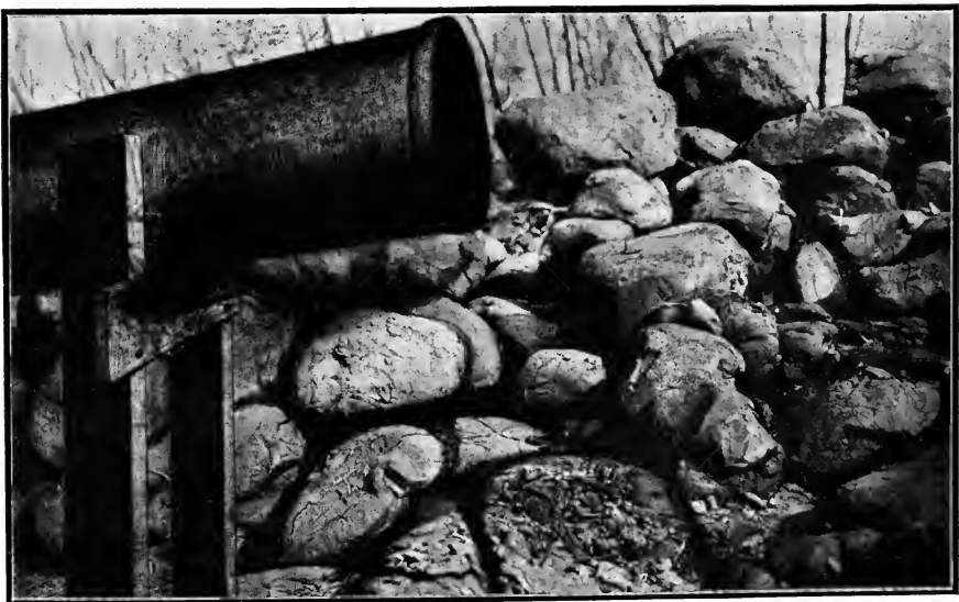
Lumps of clay at mouth of discharge pipe, sometimes weighing 300 pounds.
