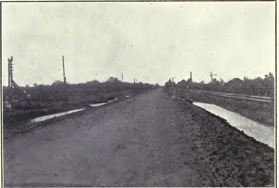
MARIPOSA ROAD AFTER IMPROVEMENT. THIS ROADWAY REMAINED PRACTICALLY UNINJURED AFTER THE FLOODS OF THE PAST WINTER.
