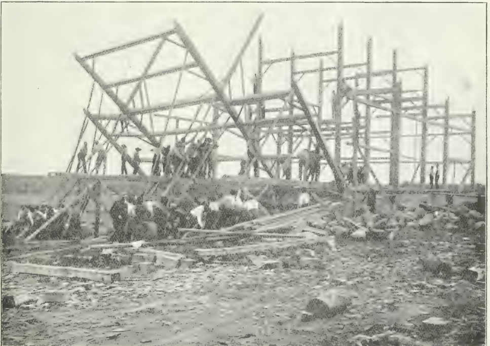
A RAINY RIVER BARN IN PROCESS OF GOING UP. TWO SIDES ARE CHOSEN, AND THERE IS ALWAYS A LIVELY RACE BETWEEN THEM TO SEE WHICH SIDE WILL GET ITS TIMBERS INTO PLACE FIRST
