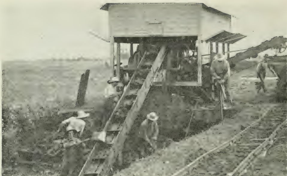
THE END ELEVATION OF A PEAT MACHINE. SHOWING THE ELEVATOR WHICH CARRIES THE PEAT OUT OF THE TRENCH, MEN AT WORK DIGGING THE PEAT AND THE TRACK ON WHICH THE CARS TRAVEL WHICH HAUL THE PEAT AWAY
