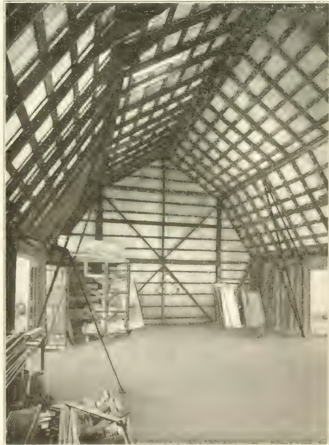
Interior view of the steel truss barn showing large amount of storage space. Note that there are no cross-timbers. Built by the Metal Shingle & Siding Co., Preston, Ont.
