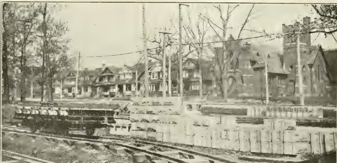
A car on which blocks are made and a quantity of granite-faced blocks. An idea of what a finished wall looks like may be had from the blocks piled up in the centre of the picture.
