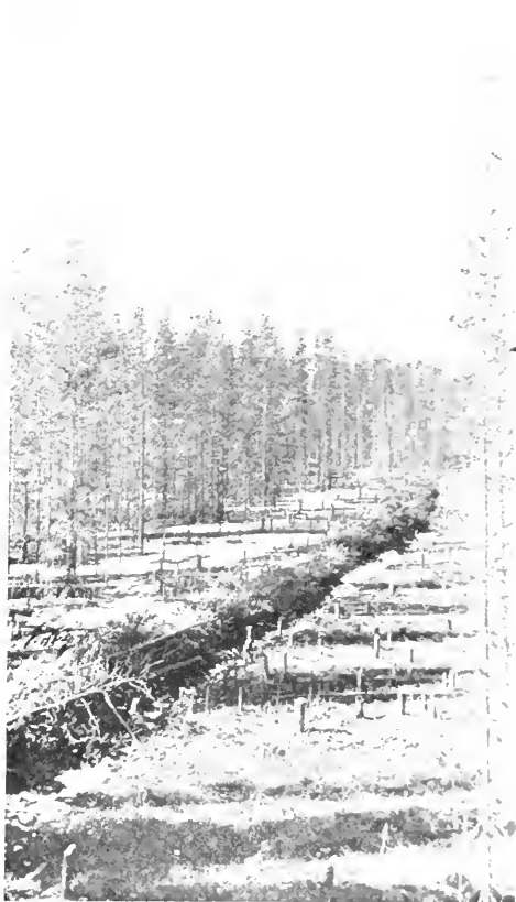
CUTTING A NEW ROAD IN BRITISH COLUMBIA Note how carefully the debris is piled for burning in the centre.
