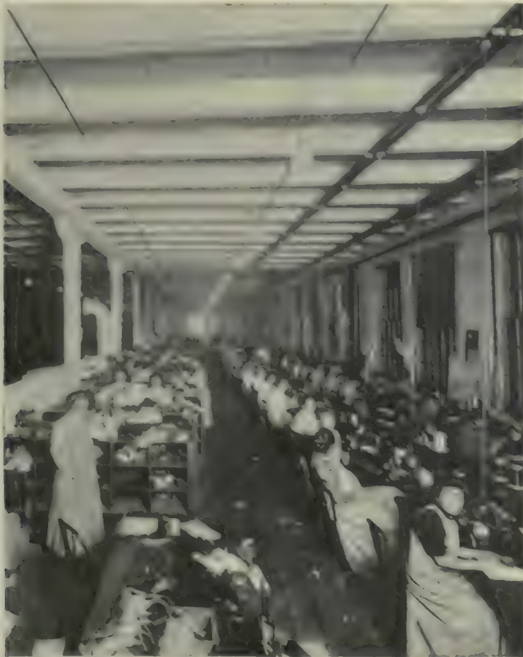
Fig. 3. General illumination of a factory obtained from a double row of one-hundred-watt tungsten lamps, provided with special distributing reflectors and hung on short drops from the ceiling, as illustrated. Special steel reflectors, each provided with an eight-candle-power carbon lamp, direct the light at the machines.
