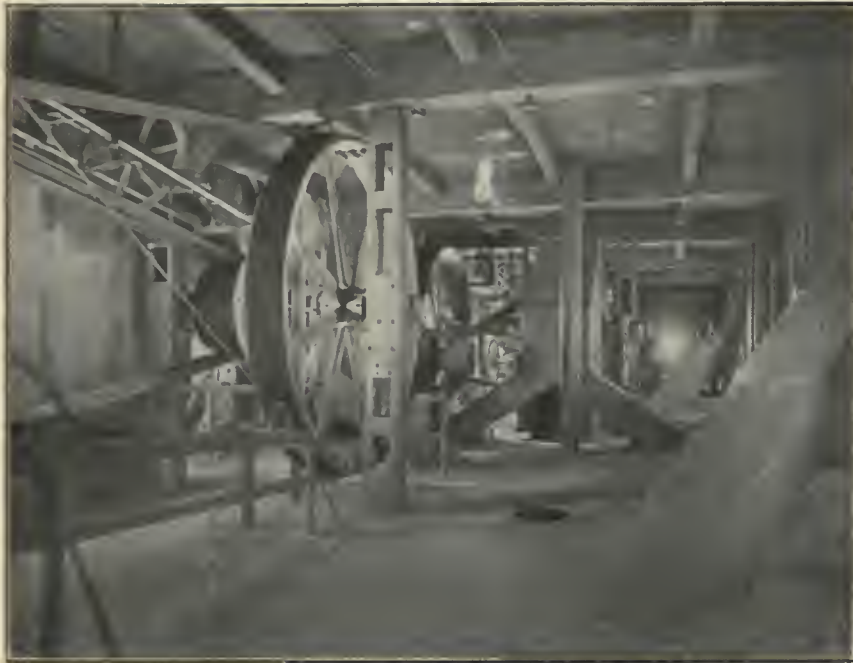
FIG. 10. TOP FLOOR. ELEVATOR HEADS AND DRIVES.
