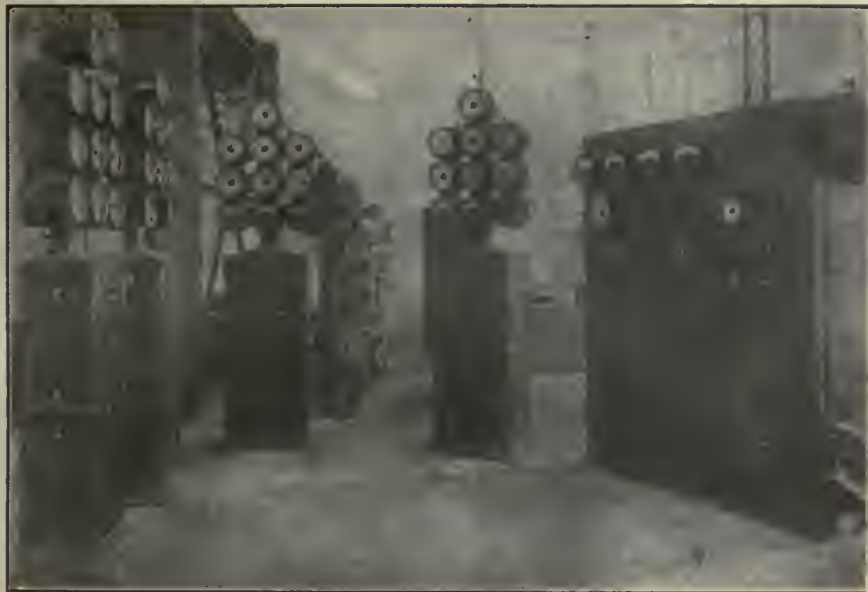
FIG. 24. SWITCH CONTROL PEDESTALS.
