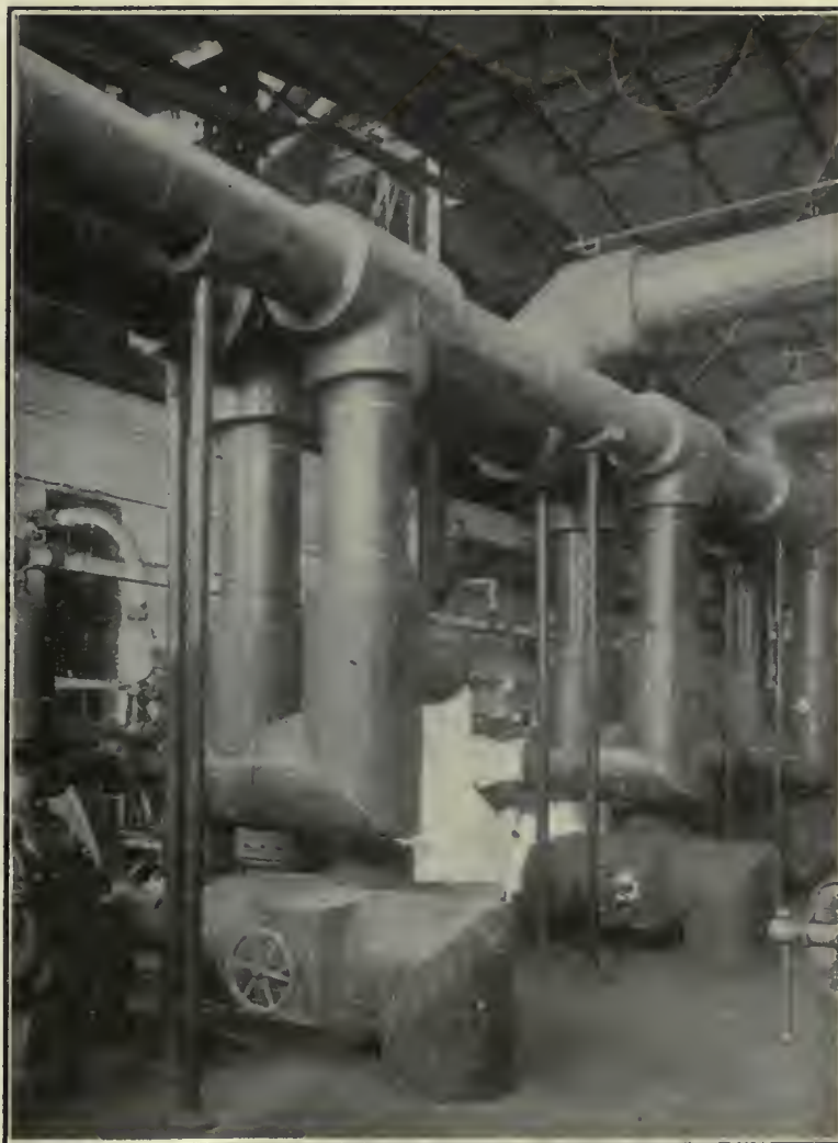
FIG. 1. CORK COVERING ON FLANGED BRINE PIPING AT STEEL CO. OF CANADA REFRIGERATING PLANT, HAMILTON, ONT. THE 8 IN. X 12 IN. SUCTION HEADERS ARE UNDER THE FLOOR.
