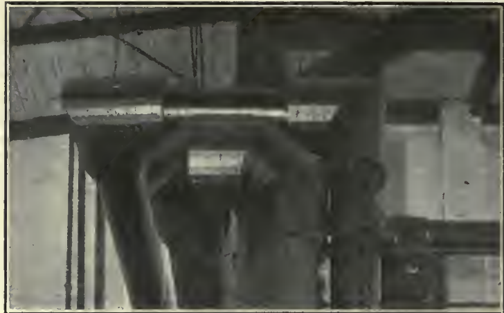
FIG. 3. A DIFFICULT PIECE OF PIPE COVERING. CORK COVERING ON 8 IN. X 12 IN. FLANGED BRINE PIPING.
