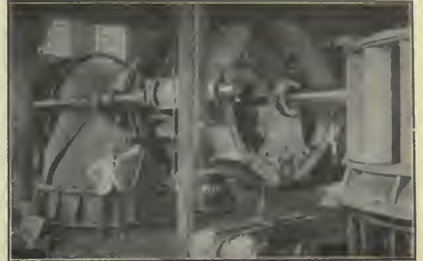
FIG. 11. VIEW OF TURBINE FROM ALTERNATOR END.
