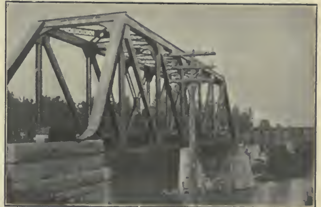
FIG. 7. THROUGH RIVETED LATTICE GIRDER SPAN AND THROUGH PLATE GIRDER SWING SPAN (IN THE DISTANCE), ERECTED OVER RIVER THAMES, AT CHATHAM, ONTARIO.
