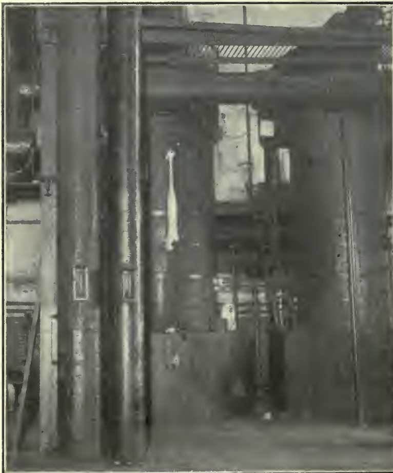
FIG. 2. VIEW SHOWING TWO VERTICAL BRINE COOLERS (SHELL TYPE), INSULATED WITH CORK LAGGING. TOP AND BOTTOM BOXED IN AND FILLED WITH GRANULATED CORK, ALSO SHOWING 8 IN. X 12 IN. BRINE RISERS.
