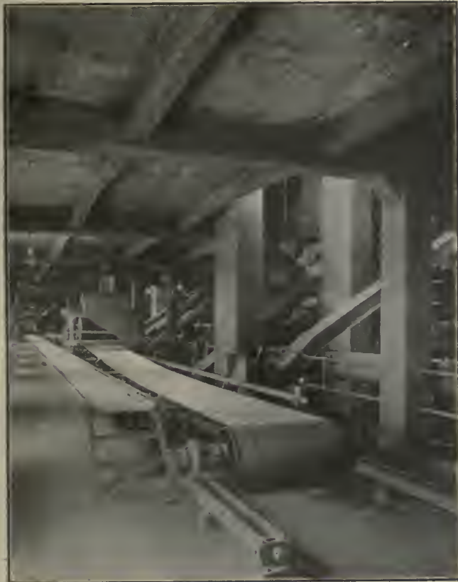
FIG. 6. BELT CONVEYORS IN SECOND STOREY OVER BINS.
