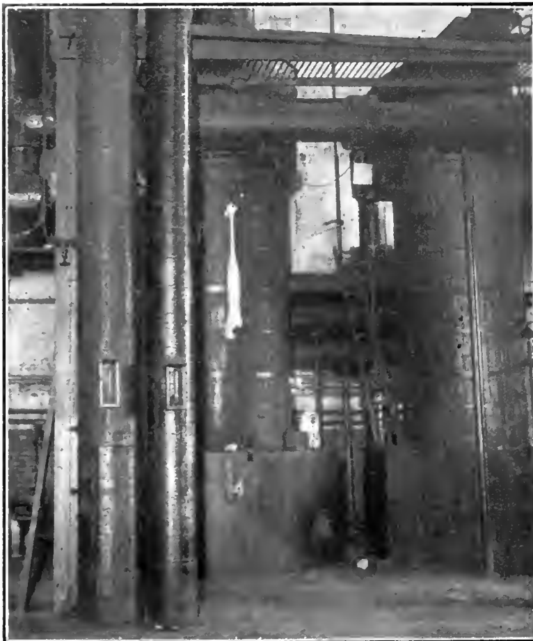
FIG. 2. VIEW SHOWING TWO VERTICAL BRINE COOLERS (SHELL TYPE), INSULATED WITH CORK LAGGING. TOP AND BOTTOM BOXED IN AND FILLED WITH GRANULATED CORK, ALSO SHOWING 8 IN. X 12 IN. BRINE RISERS.
