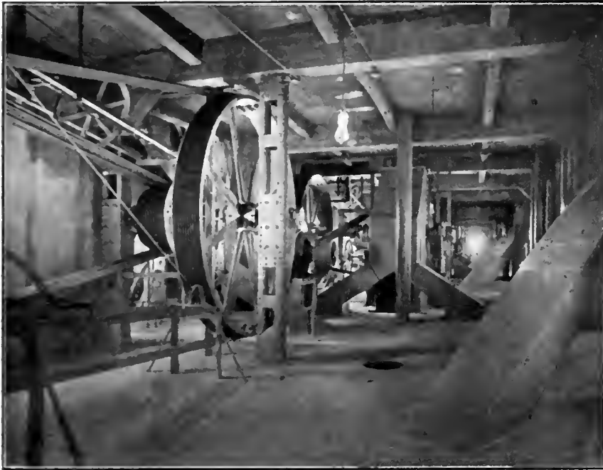
FIG. 10. TOP FLOOR. ELEVATOR HEADS AND DRIVES.
