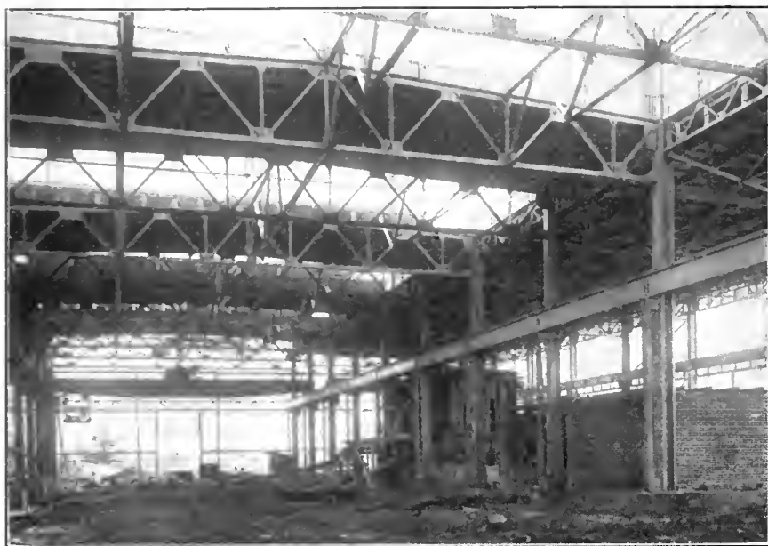
MAIN BAY OF FOUNDRY WITH DRYING OVENS AND NO. 1 OPEN HEARTH FURNACE UNDER CONSTRUCTION.
