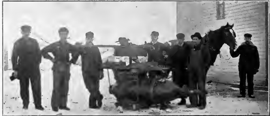
BORING 30 IN. SLUICE VALVE, CHUCKED TO EARTH AT TEMPERATURE 48 DEGREES BELOW ZERO.
