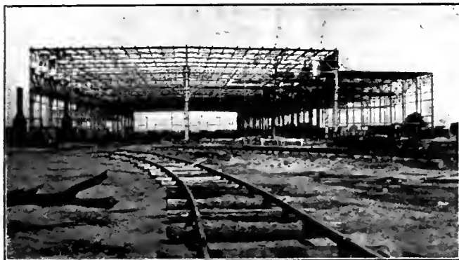
NATIONAL STEEL CAR CO. NEW PLANT. MAIN SHOP DURING COURSE OF ERECTION.
