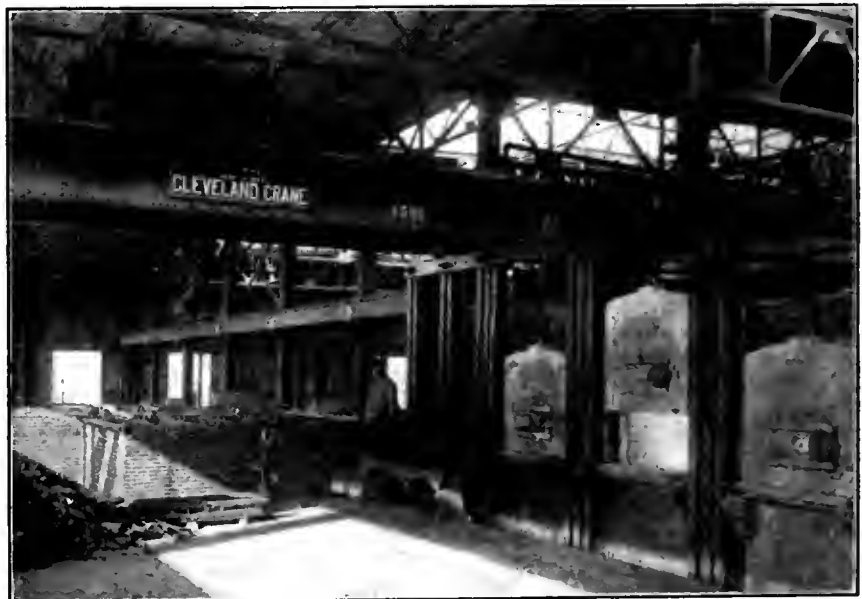
CHARGING PLATFORM, NO. 1 OPEN HEARTH FURNACE. IN THE BACKGROUND IS SEEN ONE OF THE DRYING OVENS UNDER CONSTRUCTION.
