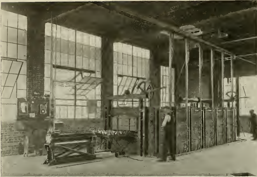
TYPICAL "ROCKWELL" 6-BURNER ANNEALING FURNACE INSTALLED, SHOWING PAN LOADED WITH CASES BEING FED INTO FURNACE BY AIR PUSHER. DUPLICATE PIPES AT SIDE ARE FOR FUEL OIL OR NATURAL GAS.
