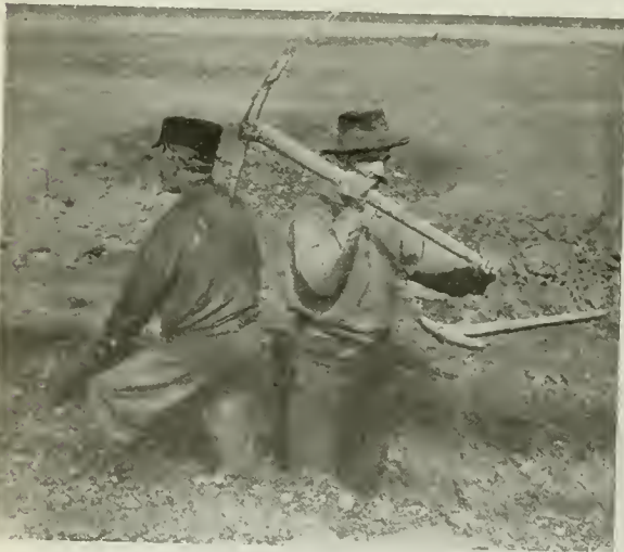
FIG. 27. EXCAVATION OR DITCHING, SHOWING LIABILITY TO SERIOUS ACCIDENT IF MEN WORK TOO CLOSE TOGETHER.
