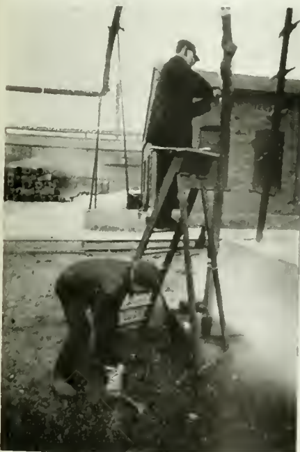
FIG. 33. WORKMAN PLACES WRENCH CARELESSLY ON LADDER PLATFORM
