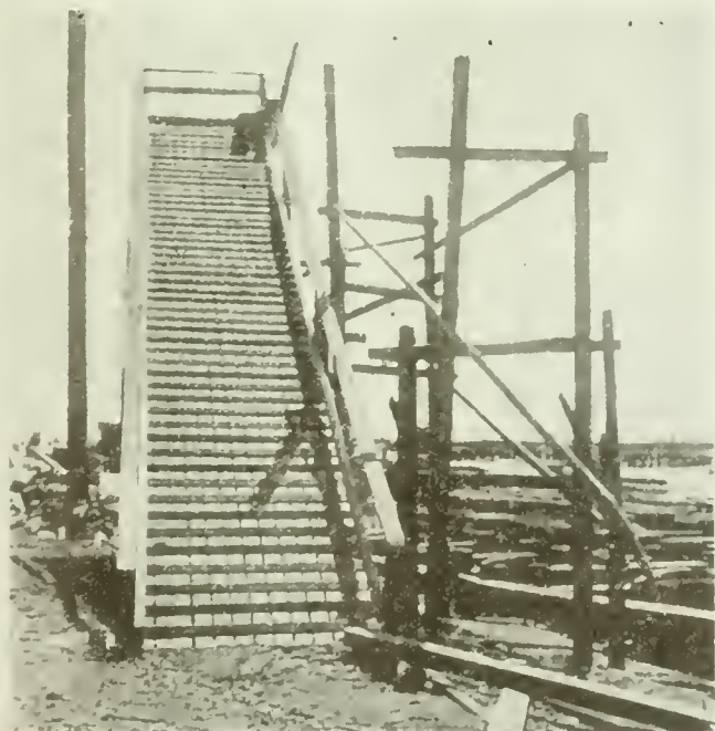
FIG. 6. WELL CONSTRUCTED MAIN APPROACH, WHICH IS A PERMANENT STRUCTURE, GIVING DIRECT ACCESS TO THE UPPER DECK OF A SHIP ON THE STOCKS.
