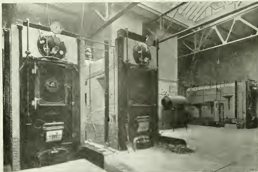
BOILER ROOM ONE 100 H.P. AND TWO 50 H.P. BARBOCK & WILCOX WATER TUBE BOILERS.
