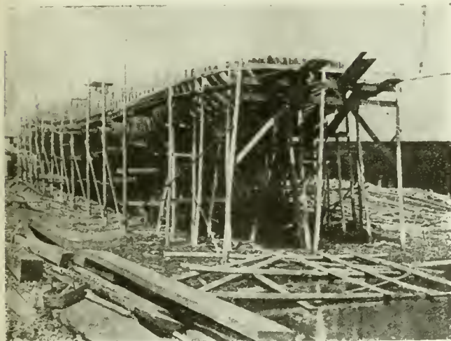
FIG. 1. A THREE-DECK STAGING. THE BOARDS ARE LAID LOOSELY AND NO GUARD RAILS ARE PROVIDED.
