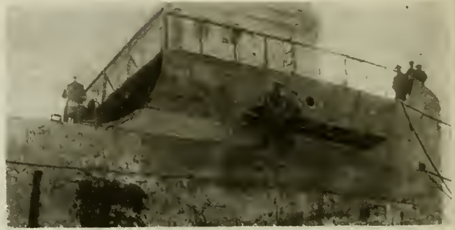
FIG. 5. RIVETERS WORKING FROM A SUSPENDED STAGING. THE RIVET HEATING FORGE AT THE LEFT IS TOO FAR FROM THE RIVETERS FOR SAFETY OR EFFICIENCY.
