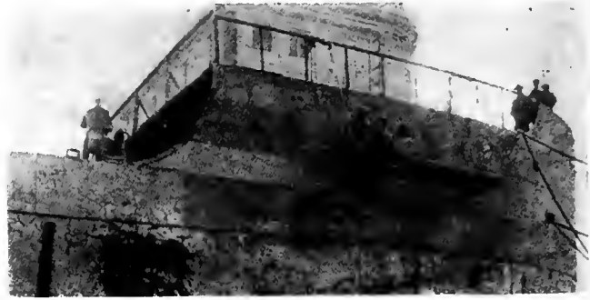
FIG. 5. RIVETERS WORKING FROM A SUSPENDED STAGING. THE RIVET HEATING FORGE AT THE LEFT IS TOO FAR FROM THE RIVETERS FOR SAFETY OR EFFICIENCY.
