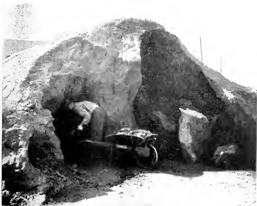
FIG 30—MAN CUTTING TOO FAR BENEATH BANK OF EARTH; A DANGEROUS PRACTICE
