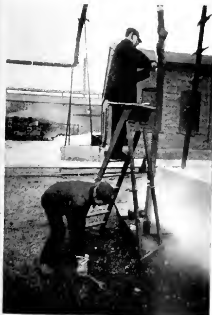
FIG. 33. WORKMAN PLACES WRENCH CARELESSLY ON LADDER PLATFORM
