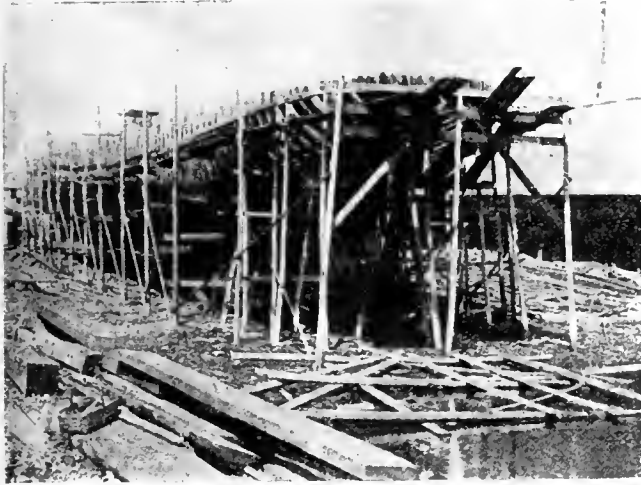
FIG. 1. A THREE-DECK STAGING. THE BOARDS ARE LAID LOOSELY AND NO GUARD RAILS ARE PROVIDED.
