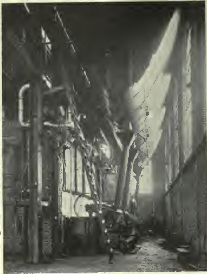
B. & W. BOILERS SUSPENDED BUNKER, AND CHAIN GRATE STOKER
