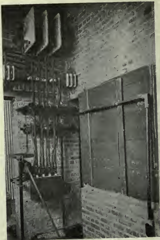
INCOMING LINE AND OIL SWITCH
