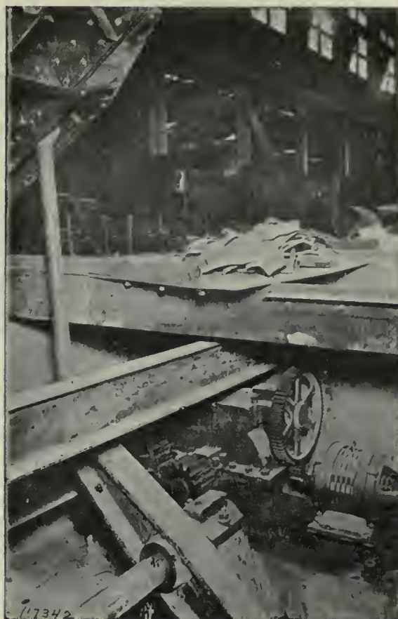
TILTING MECHANISM AND COUNTERWEIGHT SHAFT. WESTINGHOUSE MOTOR USED
