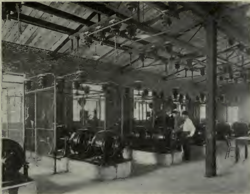
COTTRELL PRECIPITATION PLANT—SEVEN 25 KW. C.G.E. MOTOR GENERATOR SETS SUPPLY ALTERNATING CURRENT TO THE STEP-UP TRANSFORMERS
