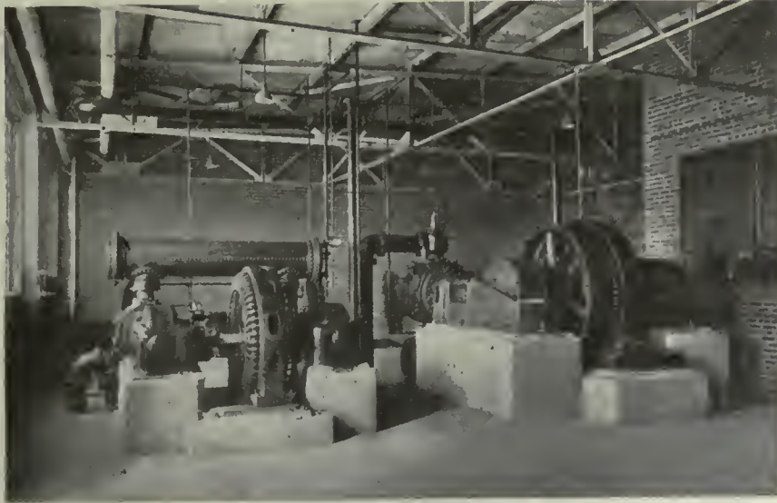
INTERIOR OF SUBSTATION, WESTINGHOUSE PLANT.
