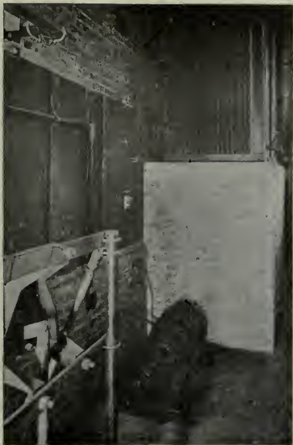
WESTINGHOUSE TRANSFORMER MOUNTED ON PEDESTAL TO SHORTEN LENGTH OF SECONDARY LEADS. BELOW: MOTOR GENERATOR SET FOR CONTROL MECHANISM
