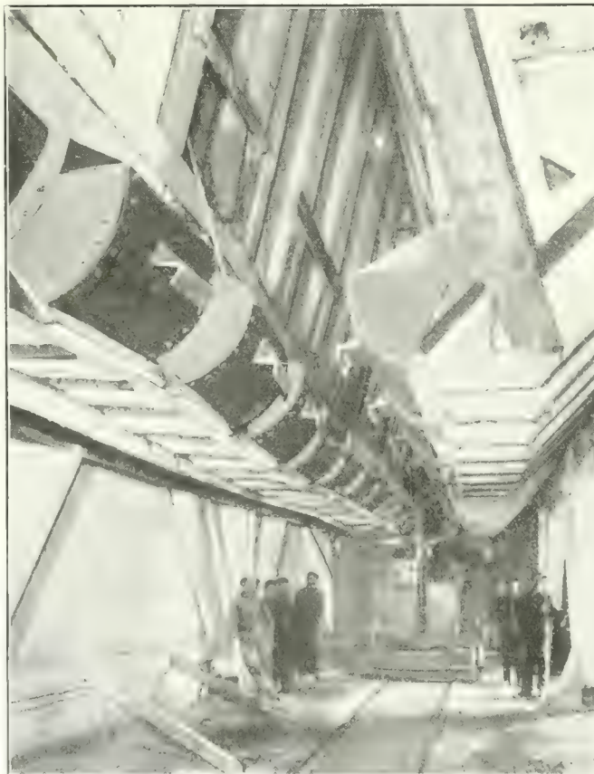
ELECTRICALLY DRIVEN CHARGING CAR WHICH WEIGHS THE ORE COKE, ETC. AS DELIVERED BY OVER-HEAD CHUTES FROM CHARGING BINS
