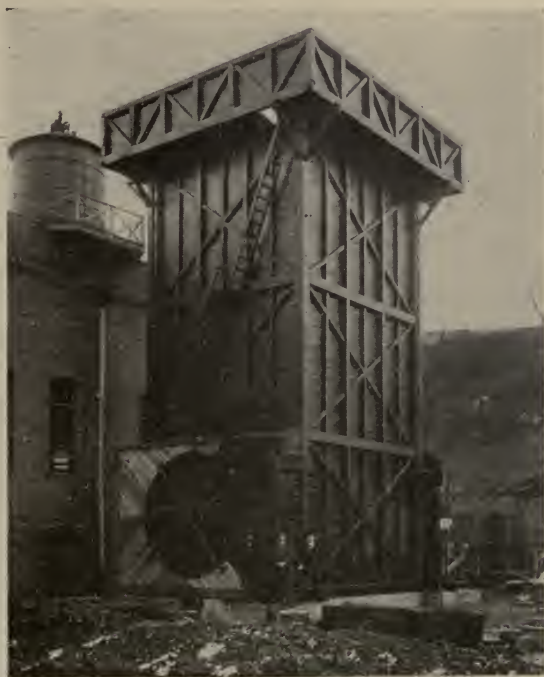
FIG. 76.—ANOTHER TYPE OF COOLING TOWER CONSTRUCTED ENTIRELY OF WOOD.
