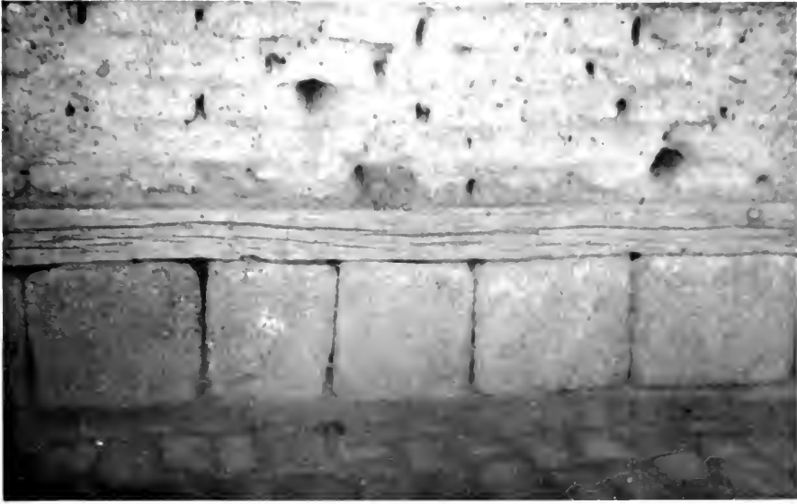
a. The lower part of a medieval mosque in the Citadel. As can be seen, the plaster is resting on the stones and transverse beams through the thickness of the masonry (cf. Islamic building methods , p. 108).
