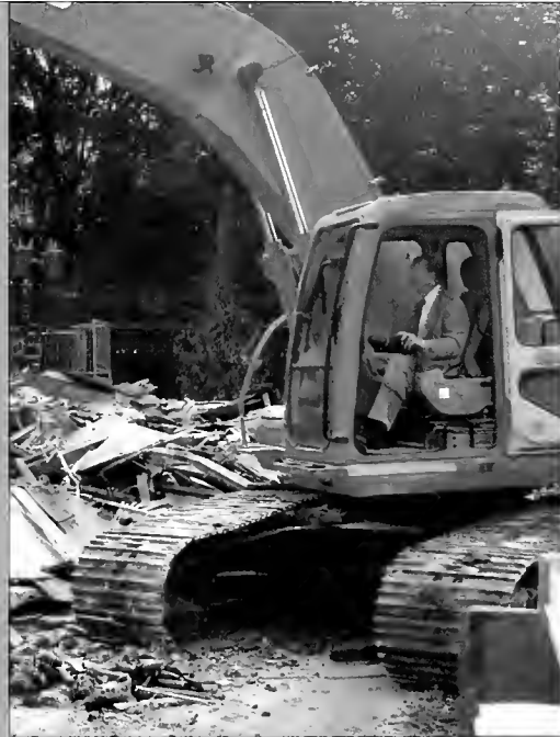
President Larry D. Large helps level former upper quad residence halls Dempsey and Trustee to make way for new student housing.
