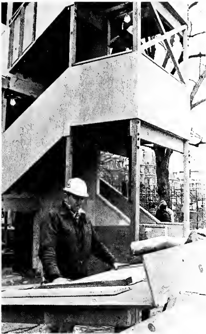
Tom "Dutch" Holland of Local 1145, job steward, looks over plans for the broadcasters' booths on Pennsylvania Avenue opposite the White House.
