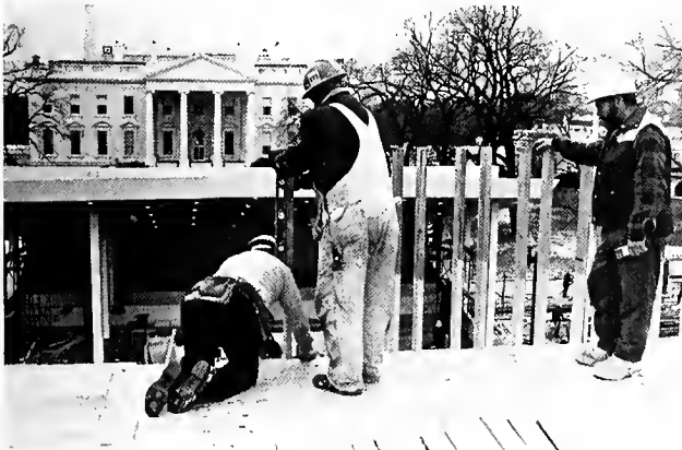
A foreman, Bruce Romesberg, left, works with Charles Kolband and Lewis Courtaney atop the broadcasters' stand on Pennsylvania Avenue. President Reagan's reviewing stand for the parade nears completion in the background. William Pritchett, D.C. business agent, covered the job for the district council.
