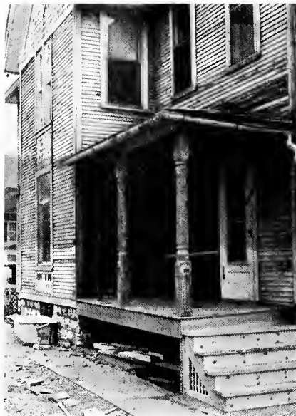
Volunteers knocked out a side wall around a contemporary bathroom to restore this side porch to the 1920's exterior; rain gutters were replaced.
