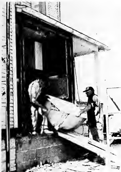
Local 790 volunteers Russell Glen of Dixon, left, and Si Witzlet remove a tub; the wall has been knocked out to restore the side porch.
