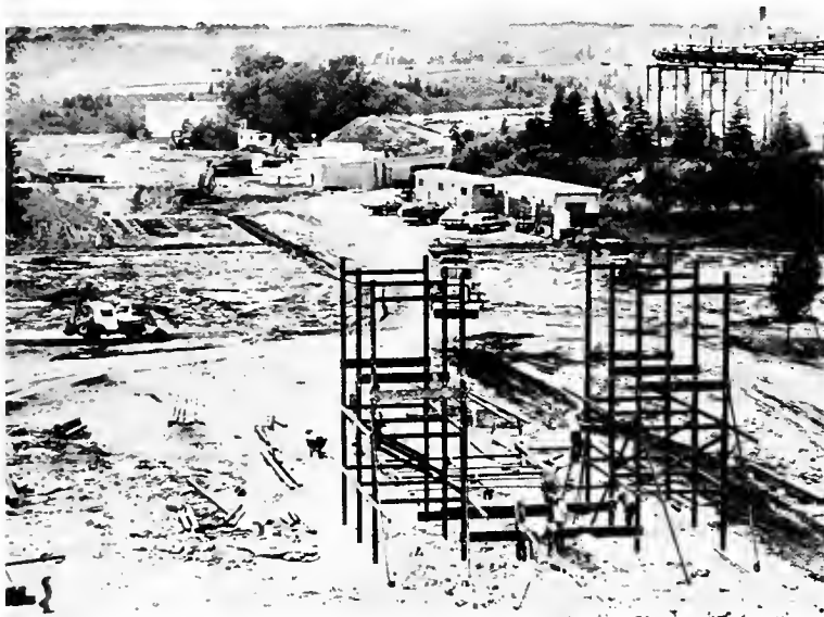
THE FIRST WOODEN BENT, or frame, was erected on July 20, 1980. Each section of a bent is six feet tall. Over 1,060,000 board feet of lumber, which has been chemically treated with a wood preservative, will be used to build the coaster. Carpenters are shown here as they began putting up the framework for the first giant hill guests will face when they ride The Eagle.
