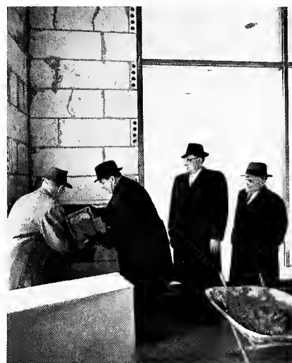
General President M. A. Hutcheson officiated at the placement of the cornerstone, becoming a trowel tradesman temporarily. In the copper cornerstone box went a number of items of historical significance, including copies of the Carpenter constitution and by-laws, union roster and other papers which indicated the healthy state of the Carpenters' Union in 1961.
