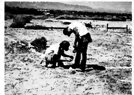
LAS VEGAS, NEV. — Two trainees lay out a building in the wide-open spaces surrounding this Western city. Las Vegas has hosted two International Carpentry Apprenticeship Contests.
