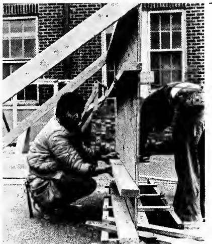
Two Seattle apprentices learn to build a concrete form under the PETS program.
