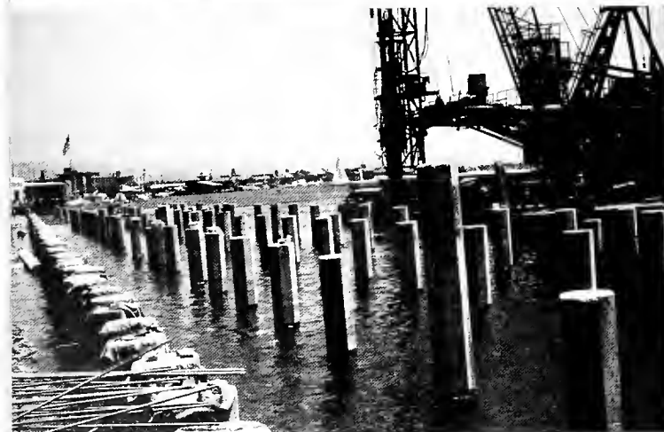
FROM THE TOP: UBC members work a pile driving rig atop the sandy soil of South Florida. They are employed by the Franki Co. In the middle picture, a California member measures the spacing of piles on a pier construction job. Lower picture, a big pier construction barge moves pile by pile, patiently completing its work in a California harbor.—All photographs by the UBC Apprenticeship and Training Department from the PETS audio-visual training materials.
