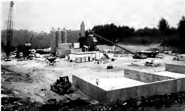
This automated batch plant for construction of the Clinch River Plant is now completed. It has icemaking equipment and boilers to control water temperatures. The plant will provide 350,000 cubic feet of concrete for the main buildings.
