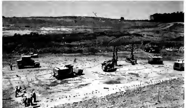
Blasting of rock continues almost daily at the site. This view of preparation includes percussion-drilling machines. Visible protrusions on the ground are plugs to keep holes open until explosives are placed.
