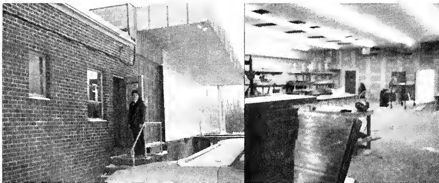
A 5,000-square-foot trucking terminal is the new site for Syracuse, N.Y., Local 12's apprenticeship and journeyman retraining center. Neil Daley, business agent and chairman of the joint apprentice committee, is overseeing the remodeling. When completed, the building will be used to instruct the PETS program, and to retrain journeymen in new skills and methods.
