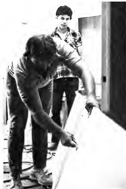
Washington, D.C., Apprentice Mark Classen cuts a sheet of drywall down to size while Apprentice Joseph Capitello stands in the background, ready to help with the installation.
