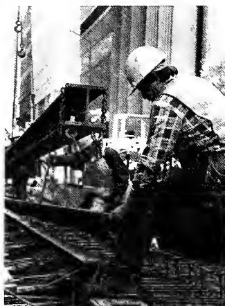
Several unions were involved with the various phases of the project. The ironworkers installed the slot rail on California Street.
