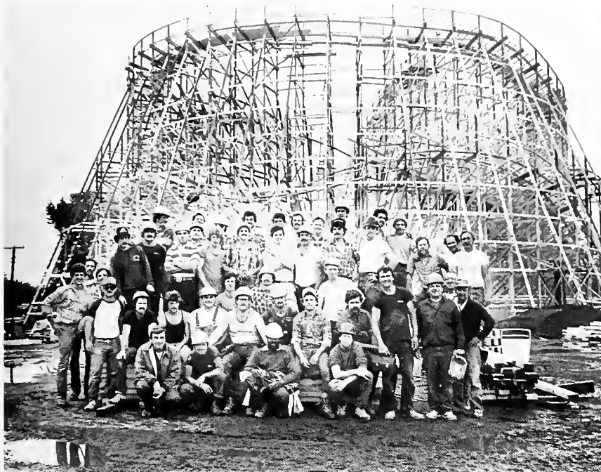
Union carpenters, mostly members of Local 108, Springfield, Mass., pose in front of the recently completed "Cyclone," one of the largest roller coasters in the world.
