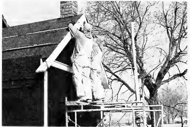
Bob Simpson and Local 61 Retiree Joe Dorman of the Kansas City District Council reinforce the roof at the rear of the house.
