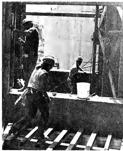
Joseph Carano, left, Catherine Barber, center, and Morris Fayer Weather, all members of Local 94, Providence, R.I., work on the Capitol Center Project in historic downtown Providence, where almost four fifths of the buildings were constructed between 1860 and 1940.
