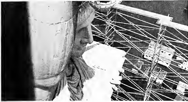
There were about 20 men working on the project for four months. Members of Timbermens Local 1536 also worked with UBC members.
