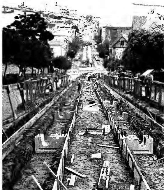
Hyde Street was one of 69 blocks cut open to place new underground structures. Here the U-shaped channelways are being installed.
