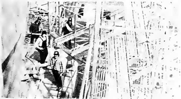
Standing near Miss Liberty's base, the monumental task of erecting 120 tons of scaffolding seems much less harrowing to these workers.
