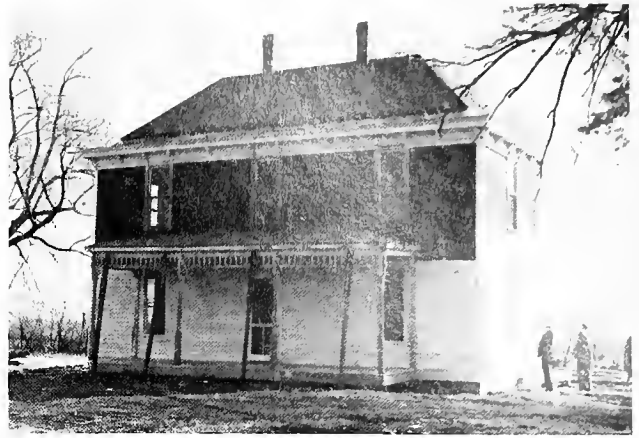
The front view of the Truman Farm Home as restoration work began. Old siding was ripped away and the porch roof was shored up.
