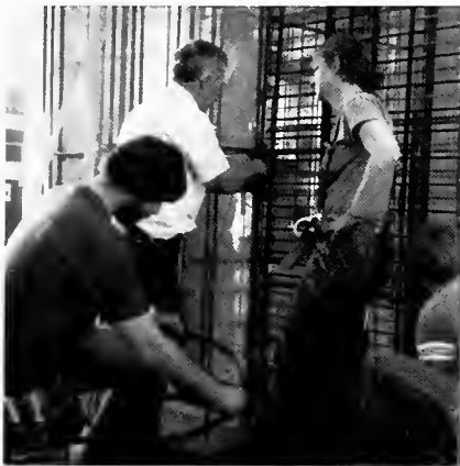
Instructor Wayne Botorff, center, gives lathing pointers to Apprentice Michael Fantazzi, left, and Kathy Ferrell, right.
