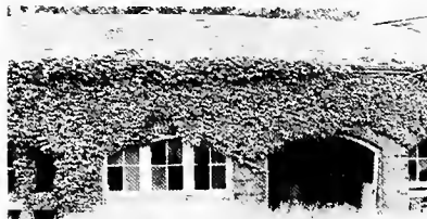
The overgrown vines and broken windows of the carpentry shed show the condition most buildings on Ellis Island were in prior to the restoration.
