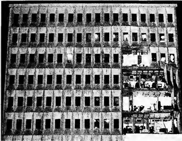
The Parkview Tower office building in Nashville, Tenn., recently suffered damage. An outer wall gave way during a rainstorm, injuring none but leaving the occupants thunderstruck and exposed to the weather. The building, we are told, was built non-union.—Nashville Banner Photograph.
