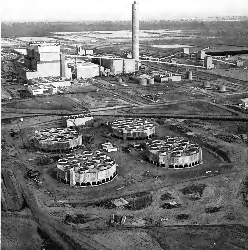
The Intermountain Power Project as it stood one year ago. The cooling towers are in the foreground; the coal handling area is at upper right; and the waste disposal areas are in the background.
