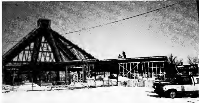
A wood-and-steel-framed St. Ann's church building is under construction in Cape Breton, Sydney, N.S.
