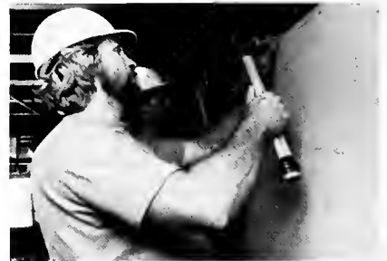
Apprentices Dean Scott, Local 906, Glendale, Ariz., rear, and Vernon New, Local 1089, Phoenix, Ariz., at work on the homeless shelter in Phoenix, Ariz.
