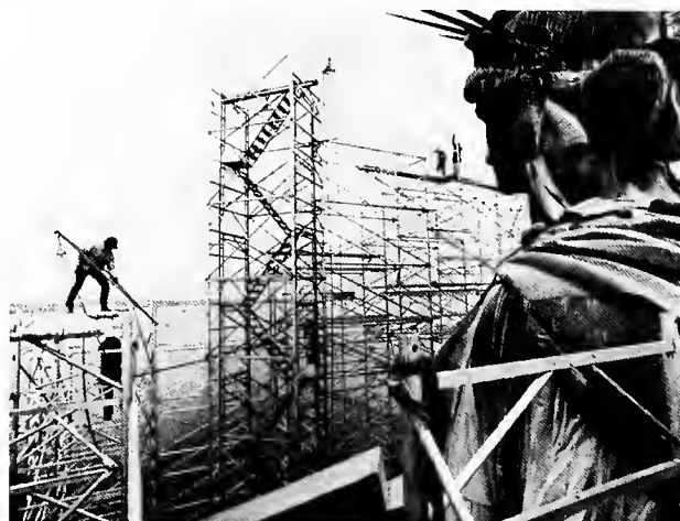
The 300-ton scaffolding was in place for a year and a half while crews worked to complete their work on schedule. Photo © Dan Cornish/ESTO.
