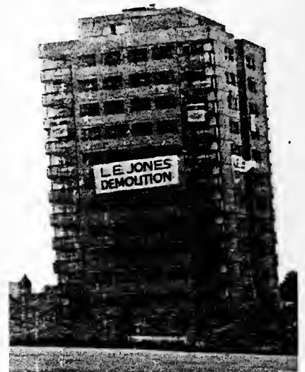
The top 12 floors of the East London apartment building, leaning like the Tower of Pisa but still intact.
