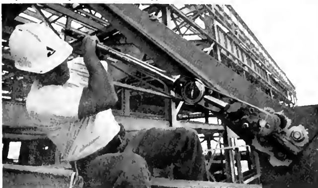
Sitting astride a steel beam, John Dorough, a civil section inspector, torques a bolt to verify the tension.
