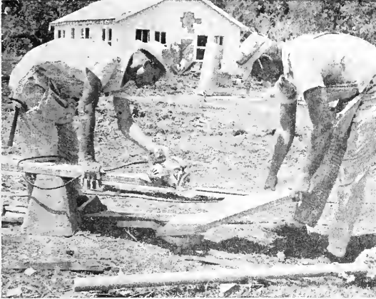
H. R. Jamison (left) and T. T. Wilson, carpenters from Shreveport, work on boards for the steps of the new home for Mrs. Clarise D. Broussard, 64-year-old widow, whose home was destroyed by Hurricane Audrey.
