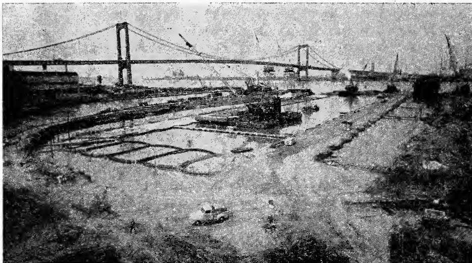
Filled with trap rock and sandy material, the cells make sturdy walls.
