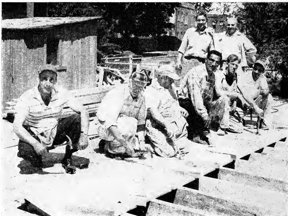
Members of Local 385 are shown working on the community-sponsored "Dream House" for the Bronx's blind Petraglia triplets. More than 100 different men from Local 385, as well as many from Local 1888, donated their Saturdays to work on the home.
