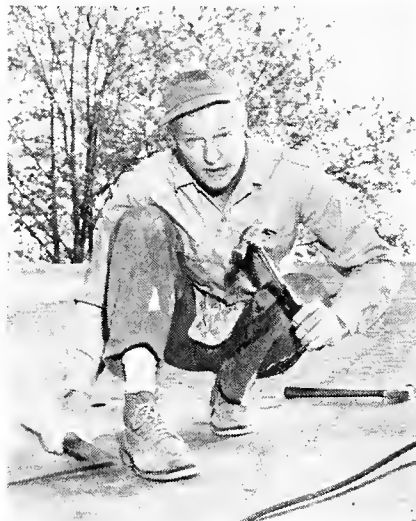
Placing roof sheathing on the Lansing workshop is Andrew Vanderbilt of Local Union No. 101.
