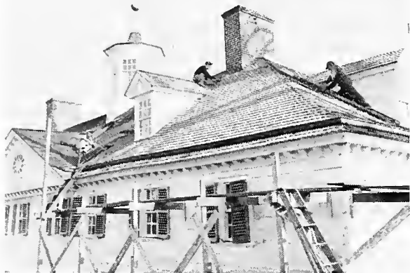
Reshingling was completed in 1953. It was done in small sections. There was no interruption to visitor flow as scaffolding was kept to minimum.
