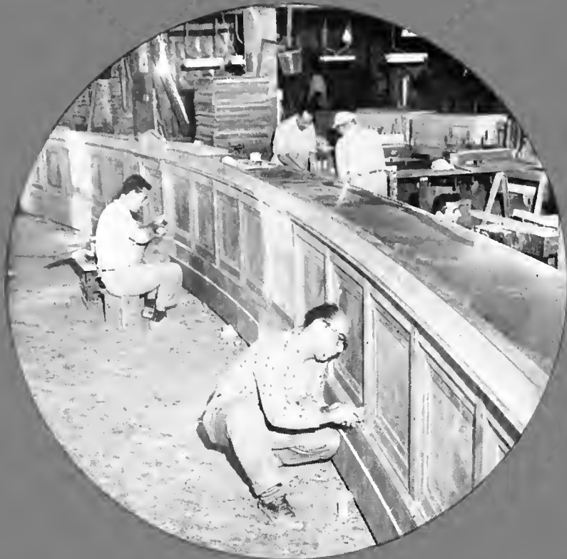
Members of Locals 1050, 1073 and 359 put finishing touches on a committee room rostrum at George Weiss Company in Philadelphia, where all millwork for the Rayburn House Office Building was done. Working surfaces of the rostrums are plastic laminates with the faces sawed walnut veneer over particleboard corestock.
