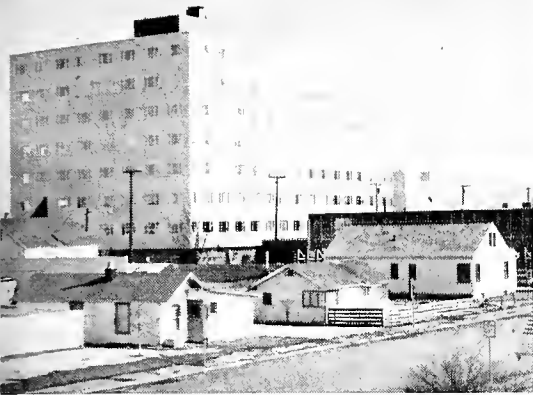
Severe structural damage. Building may have to come down.
