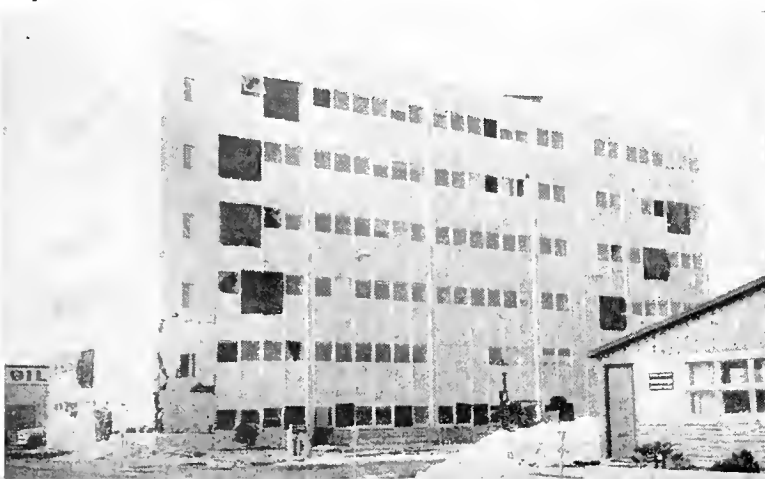
Structural steel and metal curtain wall. Severe structural damage. Building may have to come down.
