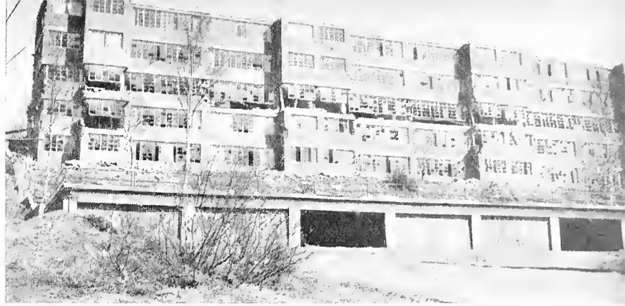
Concrete block. Just couldn't take it. Total loss.
