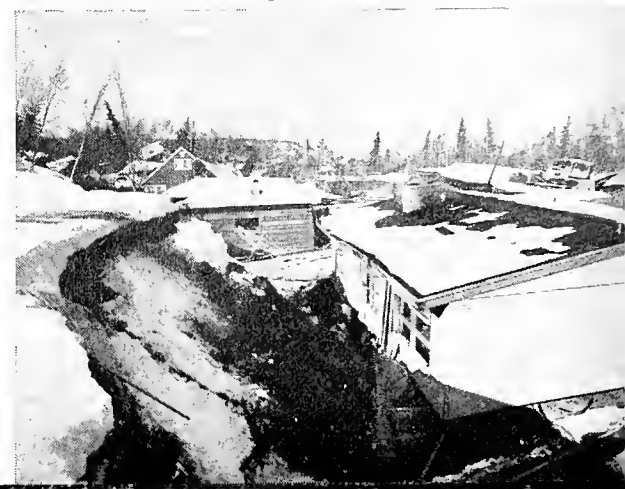
BELOW: These frame homes need new lots, new foundations, and some repairs.
