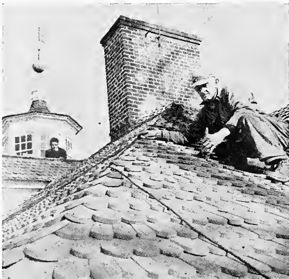
Carpenter puts finishing touches on new cypress shingles atop famous old mansion. The building underwent thorough restoration in 1952 and 1953.
