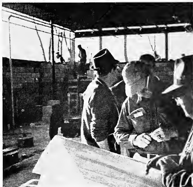
SEVERAL CARPENTERS STUDY blueprints in the $300,000 rehabilitation center that more than 8,000 building tradesmen are constructing in Gary, Ind. All construction time once again is being donated.
