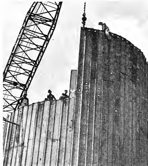
Above: Members of the United Brotherhood working on sheet steel piling for cofferdam cells during construction of TVA's largest dam, Kentucky Dam, southeast of Paducah, Kentucky.
