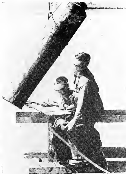
TOPPING OFF —With the precision of a trained team, two Navy Seabees saw off the excess of one of the big piles.
