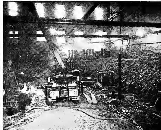
A view of the gutted interior of the theater as foundation work got under way.
