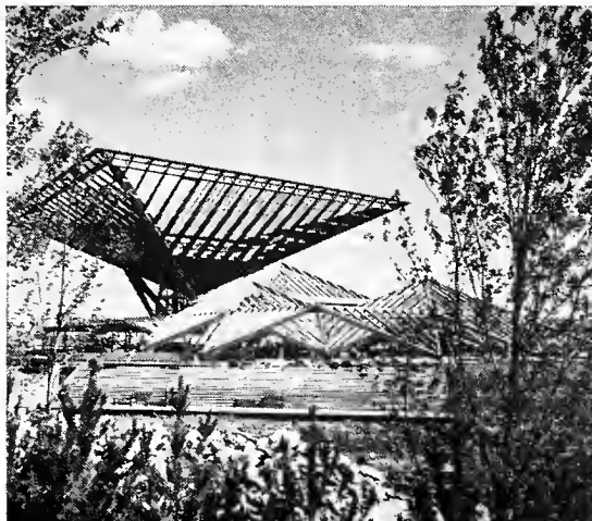
Built-up girders of laminated wood and plywood form the pine-tree-shaped Theme Building. Near photo is a view from the 65-acre park on Ile Notre Dame, a rest area on the site of Expo 67. Inverted pyramid in the center of near photo is one of Canada's exhibition buildings called Katimavik (Eskimo for "the gathering place"). Canada has earmarked $21 million for the construction of its exhibit.
