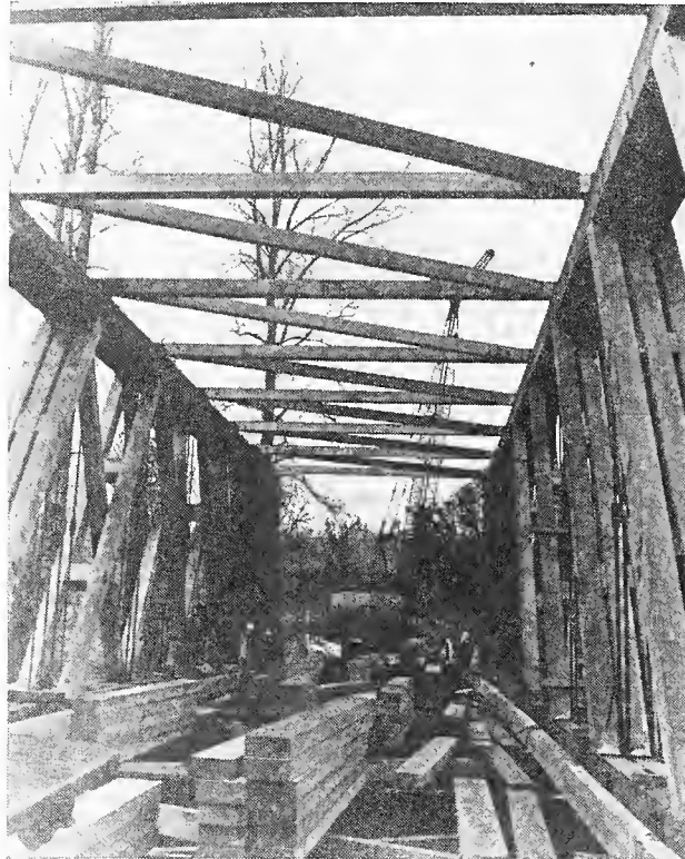
A worker's view down the center of the new bridge, showing the size of the timbers used in the restoration project at Shimanek.
