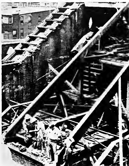
Carpenters help to rebuild the old roof. Original beams were about all that was strong enough to be retained.
