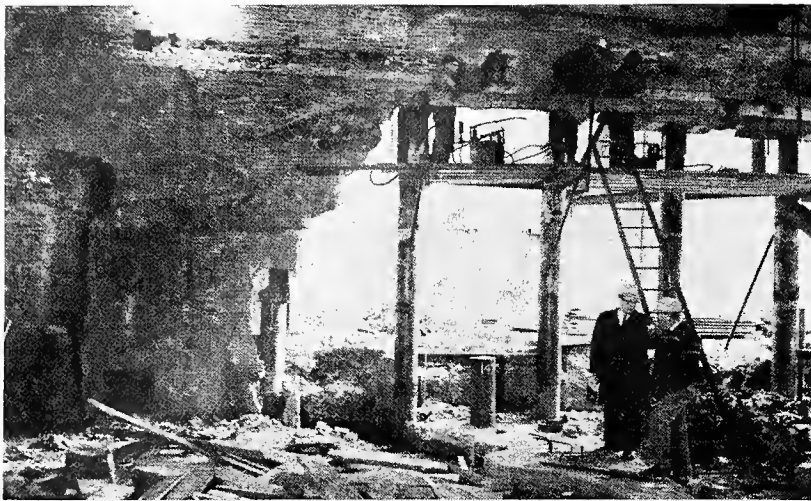
The weak foundation of the South Wall, adjacent to the restored Star Saloon, was shored with piles. Photo by Abbie Rowe, National Park Service.
