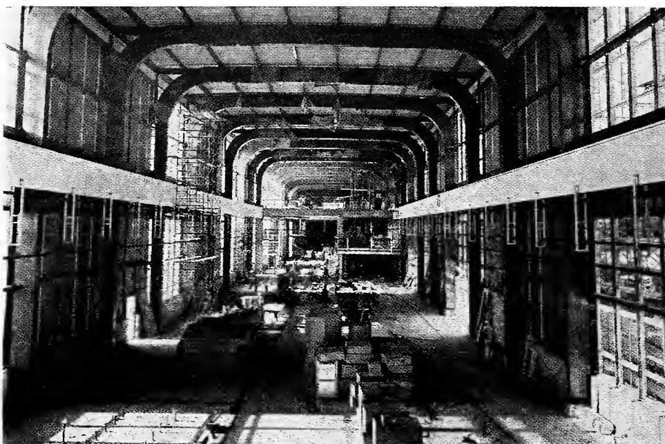
Hard Wisconsin winter did not stop members of Local 314 as they work from scaffolding (top photo) to install connecting beams between legs of 50-foot high laminated wood arch. Closed-in room of pilot plant (bottom photo) offers unobstructed work space for research.
