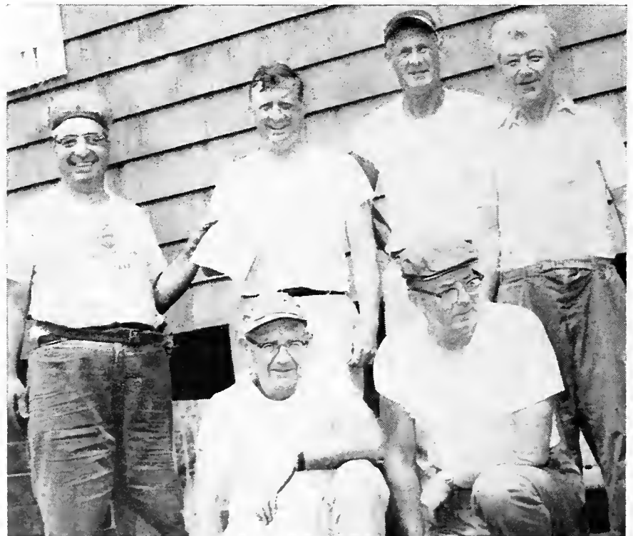
JERSEY CITY, N. J.—Carpenters from Hudson County, New Jersey, volunteered their services on a recent Saturday to help the Hudson Council of Boy Scouts dismantle a house which had been donated to the Scouts by the Harrison High School Vocational Department. The purpose of the dismantling was so that the house could be shipped to the Rock Hill Scout Reservation in Pennsylvania. Some of the Hudson County carpenters who assisted are pictured, left to right, kneeling: Morton Press, Local 383; Hugh Cuthbert, Local 482; standing: Dom Pinella, Boy Scout representative; Al Beck Jr., business representative for the Hudson County District Council of Carpenters; George Haas, Local 299; and Ted Kosiakowski, Local 486.
