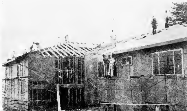
Construction progresses on group home, with members of Carpenters Local 22 contributing hundreds of man-hours.
