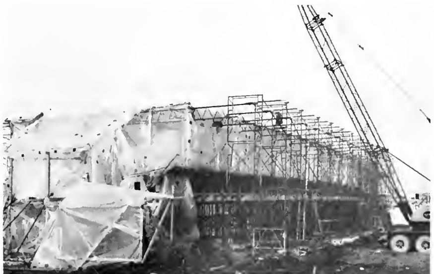
Enclosures such as this, as well as warm air-filled "balloon" structures, are being employed in many parts of the world to permit "near routine" construction to continue year round. Increased wage incentives, tax incentives to builders and price incentives to buyers are offered in some countries to accelerate construction in winter months.
