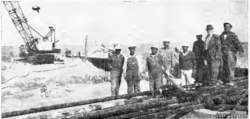
Piledrivers of Local 396 constructed a dock facility on the James River to handle equipment arriving by barge. Second from right is Business Representative and Financial Secretary John Chandler. Foreman of the job was C. Hughes, extreme right.
