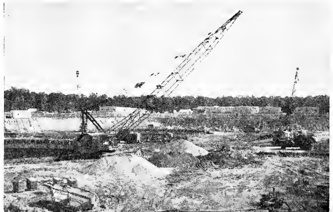
A view of the main excavation area. This excavation alone required the removal of 442,000 cubic yards of earth.
