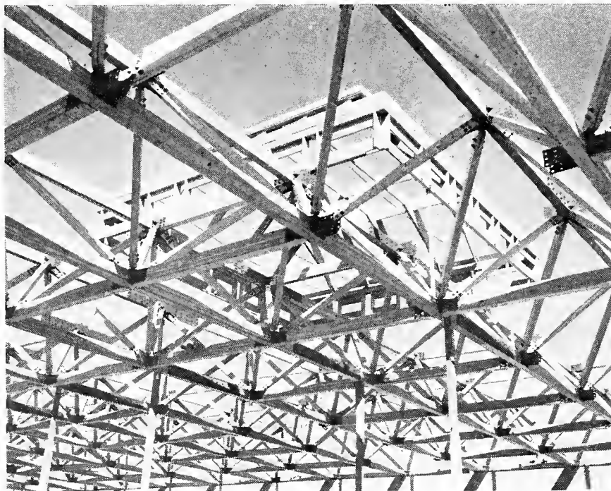
Chords are all 7 x 10½ inches, and diagonals 5¼ x 6 inches net in Lane space-frame truss system. Three large buildings required 4,272 glu-lam wood members, 1,688 gusset plate assemblies. Most web plates are 5/16 inch thick; bolts 1½ and ¾ inches in diameter.
