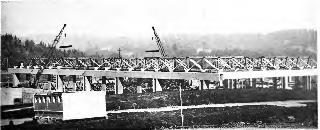
One of three large buildings chosen for wood space-frame truss roofs on $16,000,000 campus in Eugene, Oregon is shown here under construction. Extremely rigid despite 120-foot span, roof will support 5-ton moving crane as well as usual loads. Truss depth is only 8 feet.
