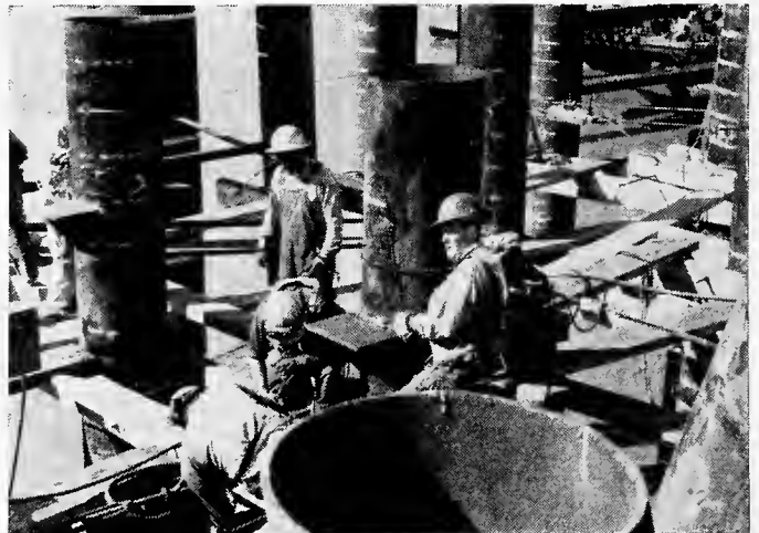
Right: Piles were aligned with hand winches, and "clips" were welded to the piles to support deck forms. The under-pinnings were of three different diameters.
