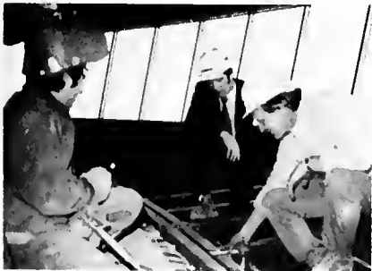
Al Carbone, left, and Bill Westbrook at work on installation of revolving restaurant deck. Keith Bonning, center, supervised the rotating deck installation.
