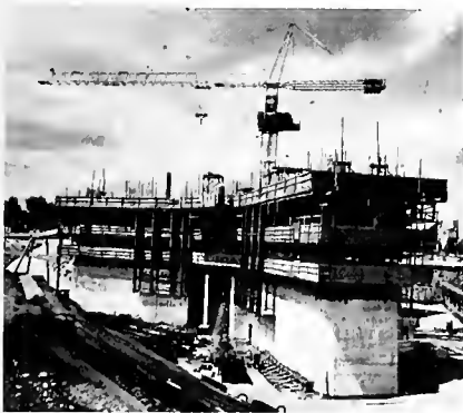
The tower at approximately 200-foot level, showing the three-story steel form, which is approximately 35 feet high on the outside.
