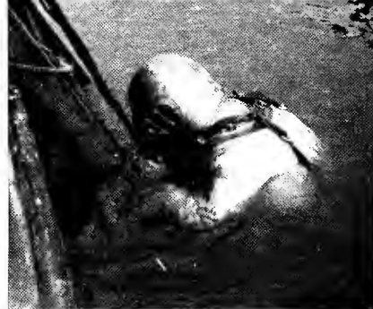
A diver wearing hard-hat gear goes down to do some repair work in the harbor at Portland, Ore.
