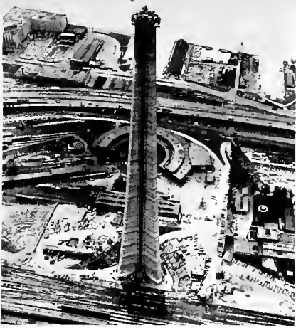
CN Tower approaches the 1,100-foot height. Four elevators in glass-faced shafts were installed in grooves of tower.
