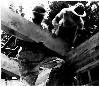
Robert Scott and Dave West, members of Local 266, Stockton, setting the large timbers for the roof.
