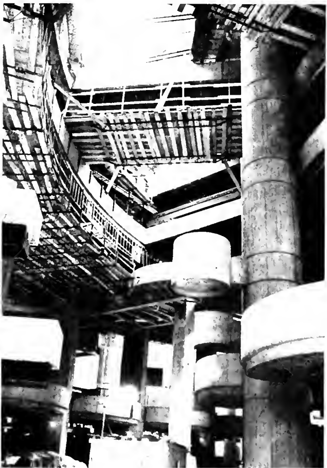
Big concrete pods and tall columns add a touch of the future to the interior of the center. An 8-story atrium will feature a half-acre lake, sculptures, trees and hanging gardens. The Detroit Plaza will feature a Coffee Garden, Cafe Express, Cocktail Pods, a Sky Lobby, and other facilities. According to reports, the hotel has already booked more than 120 conventions through 1981 and close to 400,000 room nights.
