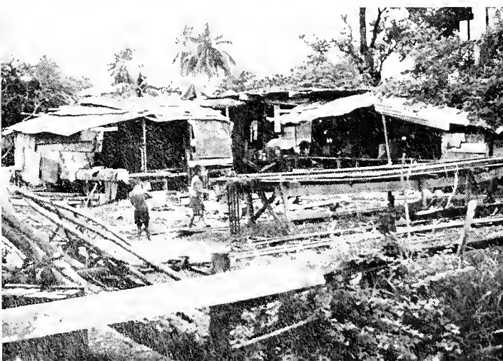
The construction site for a new hotel in Bangkok, Thailand. The shanties house the families of the superintendent and his work crew.
