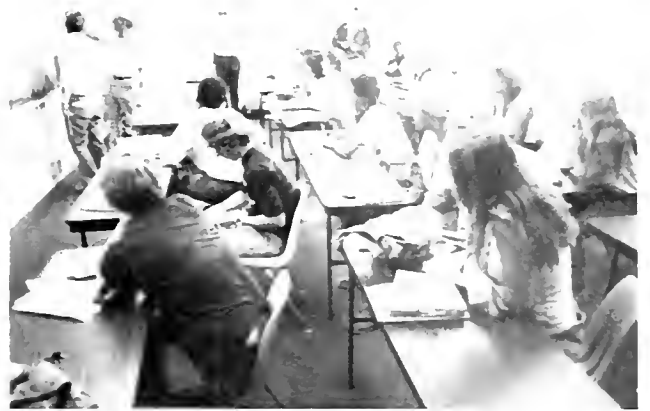
Women trainees in pre-apprenticeship build structures for community use under the supervision of Bobby Ballard, instructor/coordinator at the JATC Center, Las Vegas, Nev.
