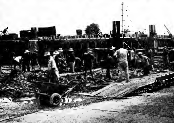
Chinese men and women work side by side on this construction job in Hong Kong. The form work shows the European influence.
