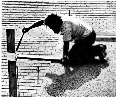
Inventor Robert Campbell positions the collar assembly on a wood support member.
