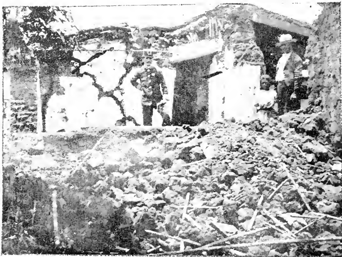
At Cartago the old adobe houses and stone walls fell or cracked.
