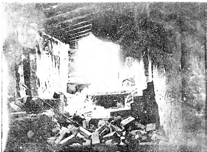
In Cartago the roofs caved in making a total wreckage.
