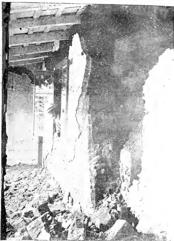
The plaster, ceilings and tiles from the roofs of buildings in San José fell all about the city, causing considerable damage.
