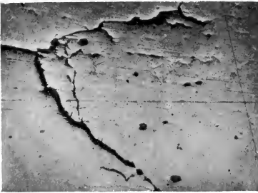
NO. 41. SHOWING SLAG CRACKS.
