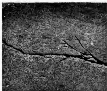
NO. 51. SLAG CRACK NEAR EDGE OF SHELLED-OUT SPOT.
