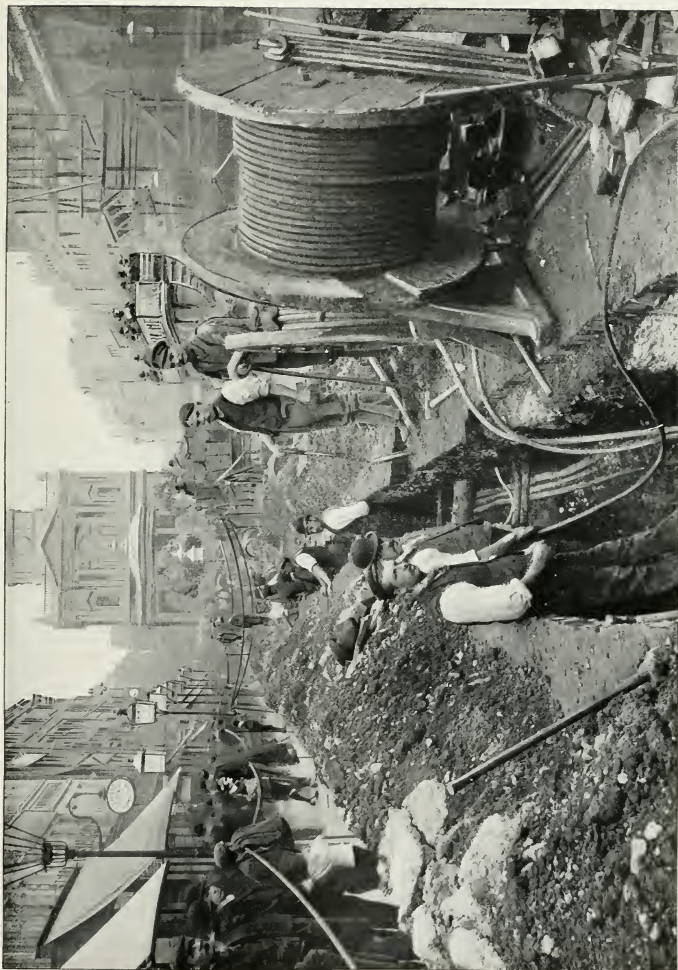
Photo supplied by Messrs. Callender and Co., Hamilton House, Thames Embankment.
