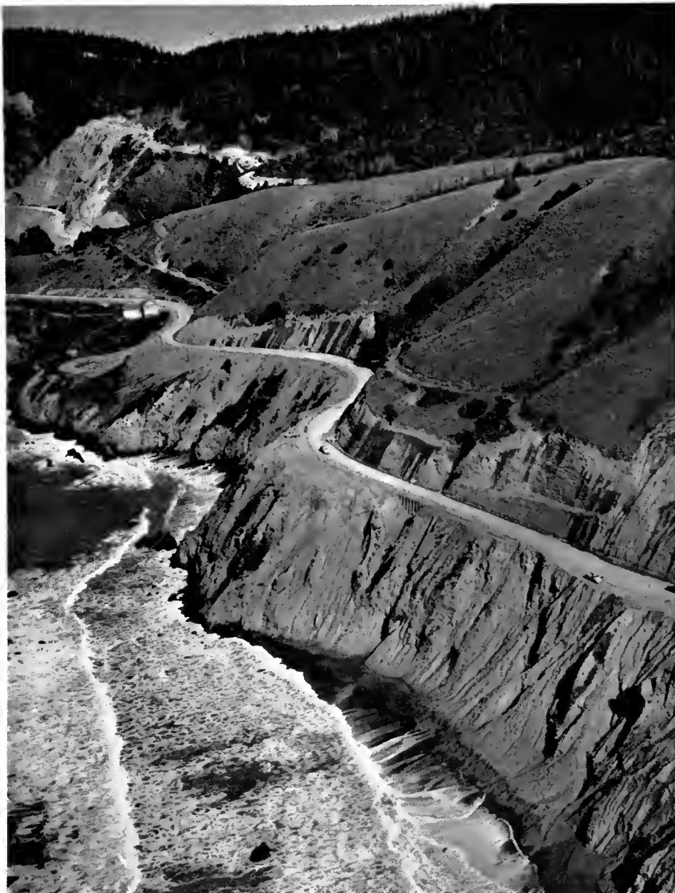
This view looks north along the reconstructed portion of State Sign Route 1 between Westport and Leggett Valley in Mendocino County. The Juan Creek Bluffs are in the left background.
