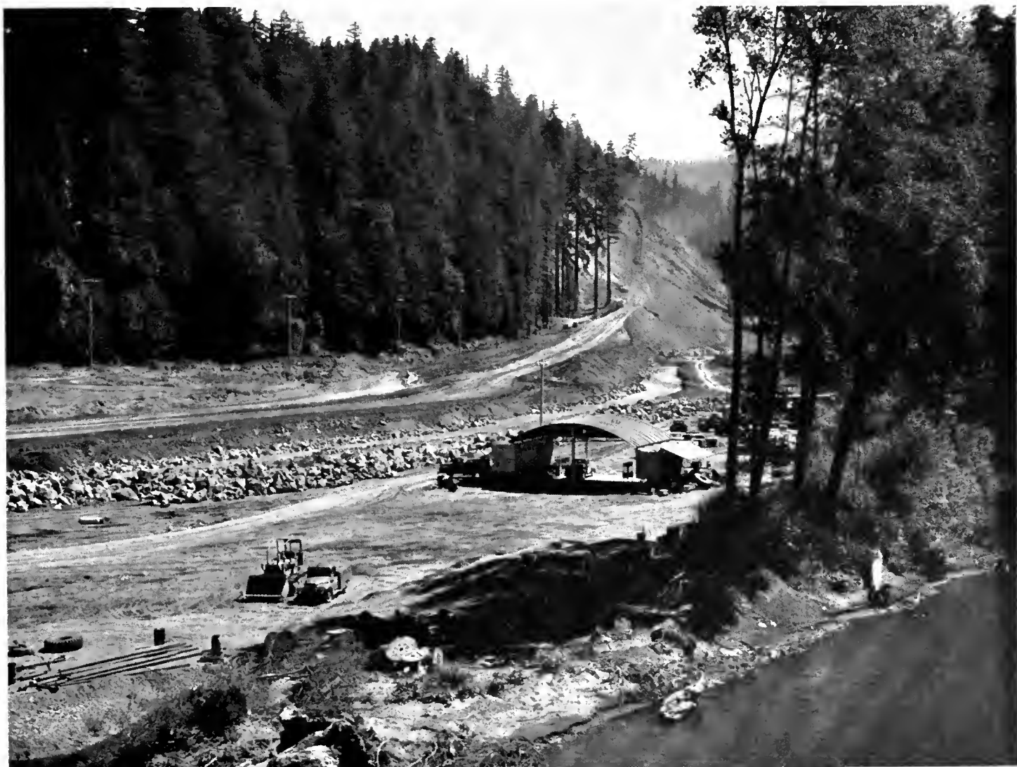
The South Fork of the Eel River shows none of the fury it unleashed in December, 1955, when it rose from elevation 110 feet to about 168 feet, overtopping existing US 101 in the right-hand portion of this picture. The projected cut failed to "catch" short of the top at elevation 650 feet.
