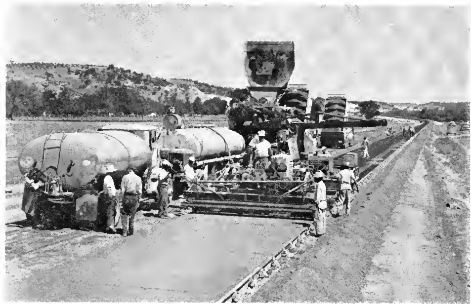
A contractor's paving train at work on a freeway section of US Highway 101 now nearing completion in the vicinity of Paso Robles
