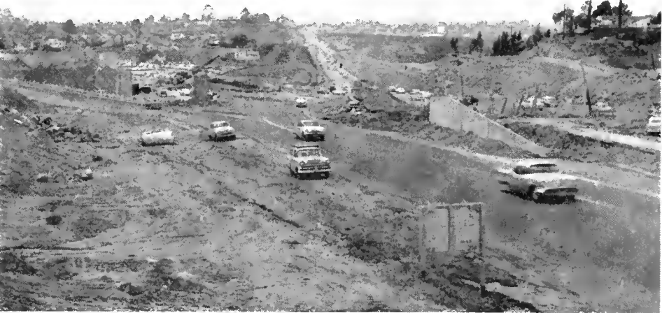
UPPER—View looking east on US 80 with Baltimore Driving Overcrossing in foreground and City of La Mesa beyond. CENTER—Looking east on US 80 showing Lake Murray Boulevard Overcrossing during construction.—LOWER—Looking west on US 80 showing construction of US 80—State Sign Route 67 interchange in the foreground.
