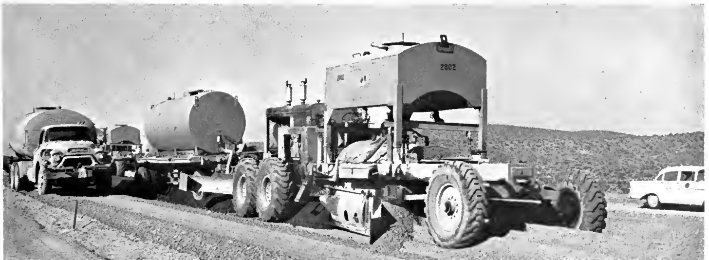
A self-propelled mixer lays cement-treated base along the Victorville-Barstow freeway. A second unit is visible in the rear.
