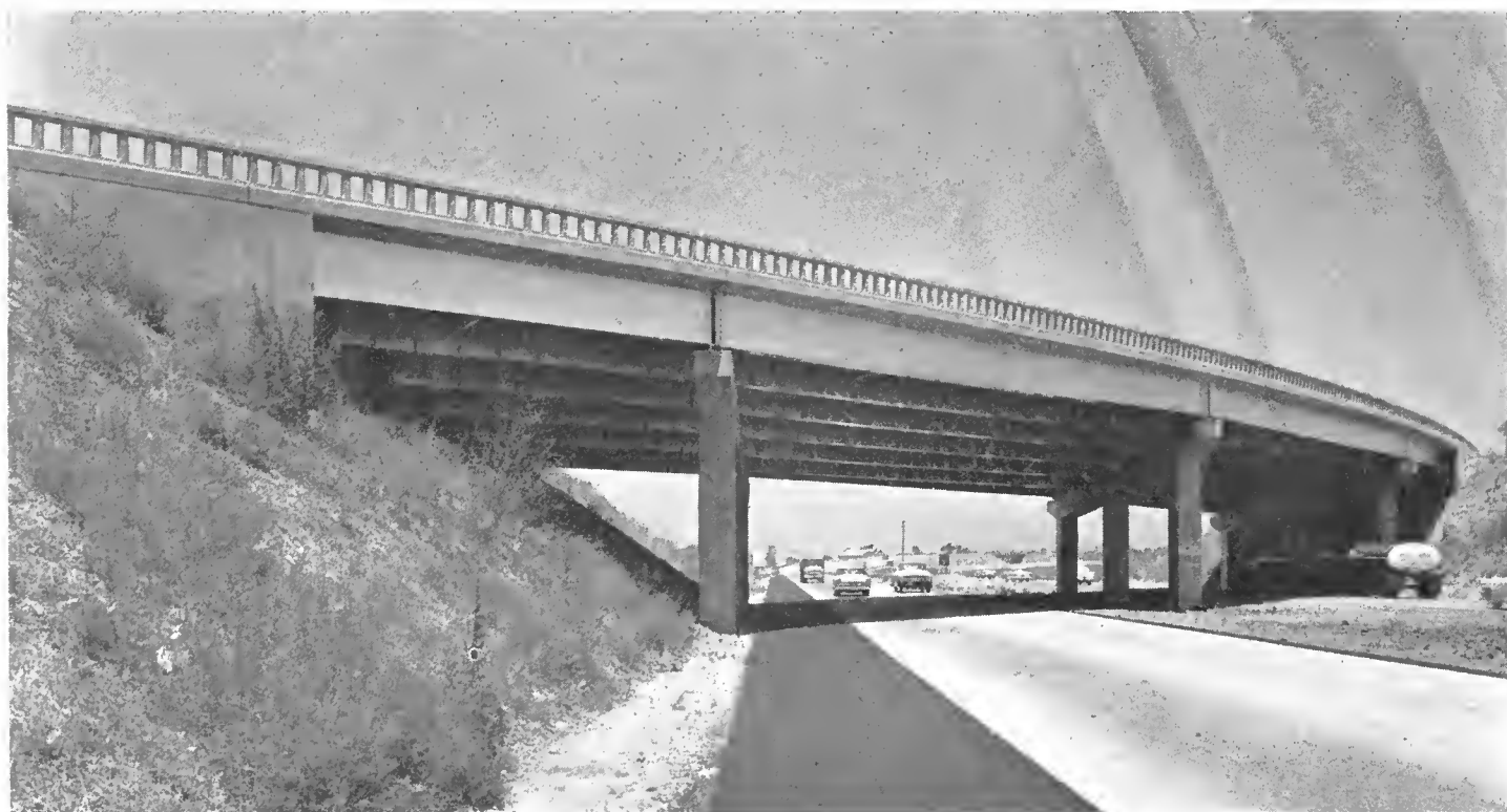
The Laguna Canyon Road separation bridge as seen from the new section of freeway. The view is northward.
