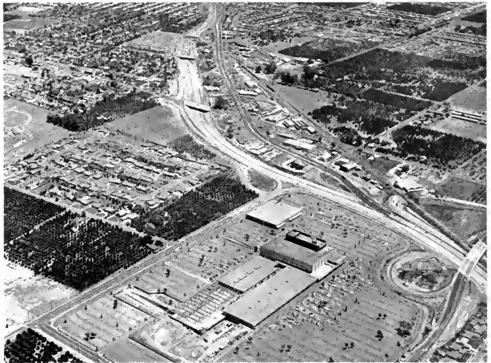
Looking southeast along construction of Santa Ana Freeway through City of Anaheim. In foreground, Braadway-Anaheim shopping center.
