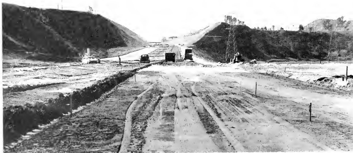
UPPER Work is progressing on the south end of the "Missing Link" section of the Riverside Freeway near the City of Riverside. The interchange in the distance will connect US 91 and 395. LOWER—The Grand Terrace Cut on the "Missing Link" section of the Riverside Freeway.
