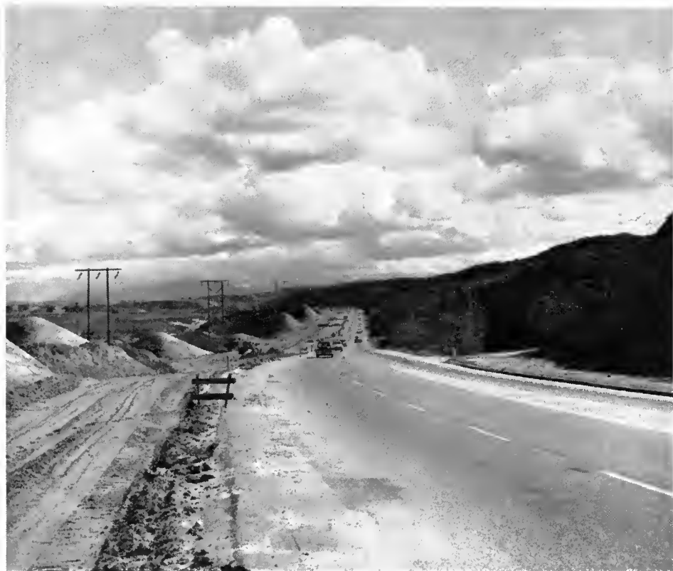
Construction now under way through the "Badlands" west of Beaumont is converting a section of US 60 to multilane, divided expressway.
