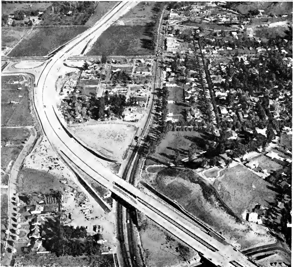
UPPER—Looking east along Ventura Freeway construction near Calabasas showing Mulholland Drive Bridge in foreground. LOWER—Looking east along Ventura Freeway construction in the Woodland Hills area.
