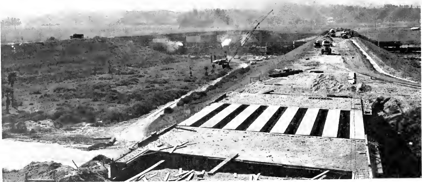
UPPER—This construction scene is on the Corona Freeway near Pine Avenue south of Chino. LOWER—A view of construction near the north end of the "Missing Link" section of the Riverside Freeway showing the Colton-Loma Linda Yard Overhead structures just south of the interchange with the San Bernardino Freeway.
