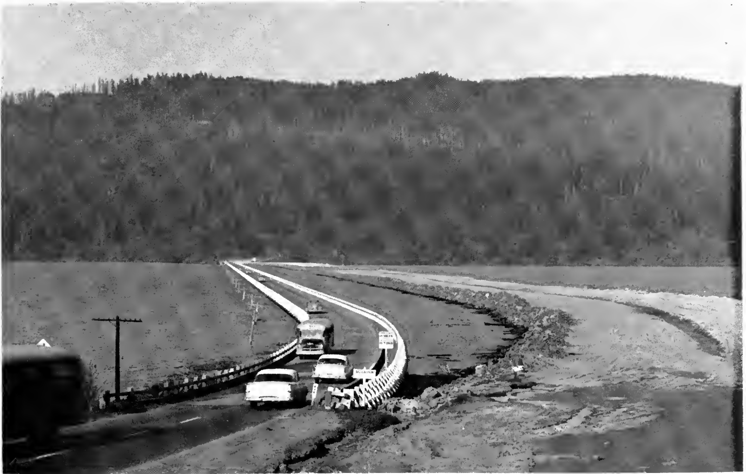
A four-lane fill between Potricks Point Pork and the north shore of Big Lagoon will replace the 4,000-foot timber trestle (left)
