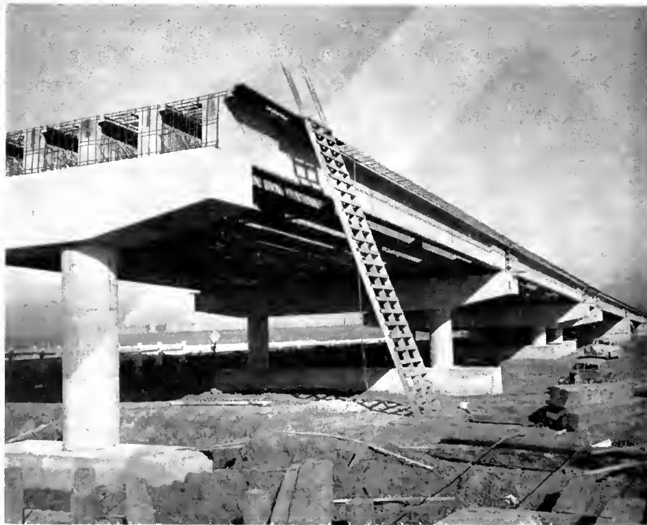
This photo of the new construction shows 80-foot, precast, prestressed girders in place on the west approach to the new bridge
