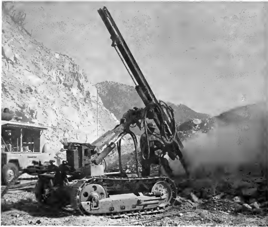
One of the late model drills being used on the Crystal Lake Road construction.
