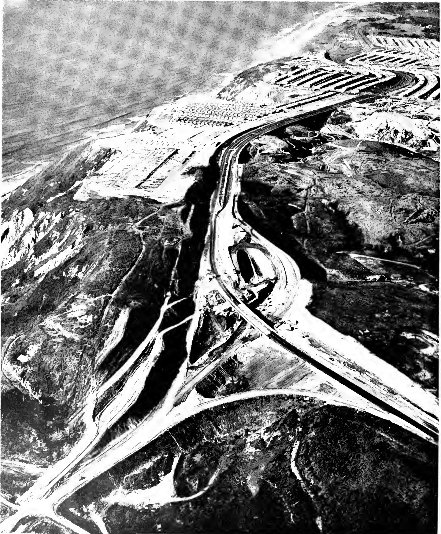
This aerial view shows the interchange under construction connecting the new freeway with Skyline Boulevard (State Sign Route 5)
