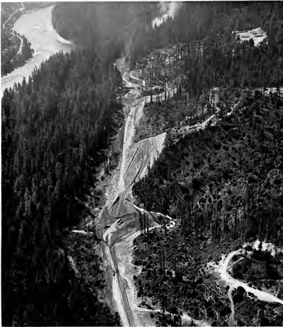
Heavy grading operations on the first unit of the Redwood Freeway. This aerial view southward was taken over High Rock Hill. The river in the upper left is the Eel.
