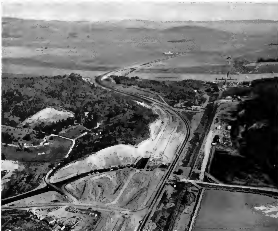
Expressway construction on the Black Point Cutoff (Sign Route 37) with the new bridge across Petaluma Creek in the upper center and the Atherton Avenue interchange in the foreground.
