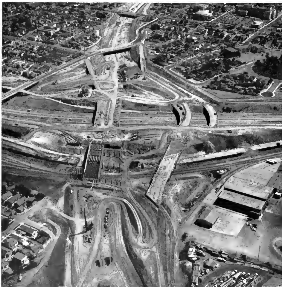
A southward view along the Golden State Freeway construction and the future interchange with the San Bernardino Freeway.
