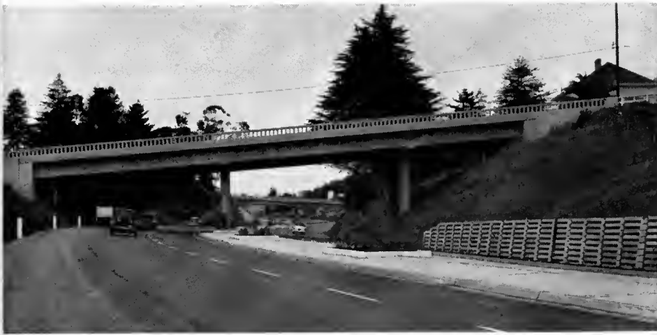
US 101 in Arcata was reconstructed on a new routing east of the central business area. This view northward shows the Ninth and 14th Street overcrossings.
