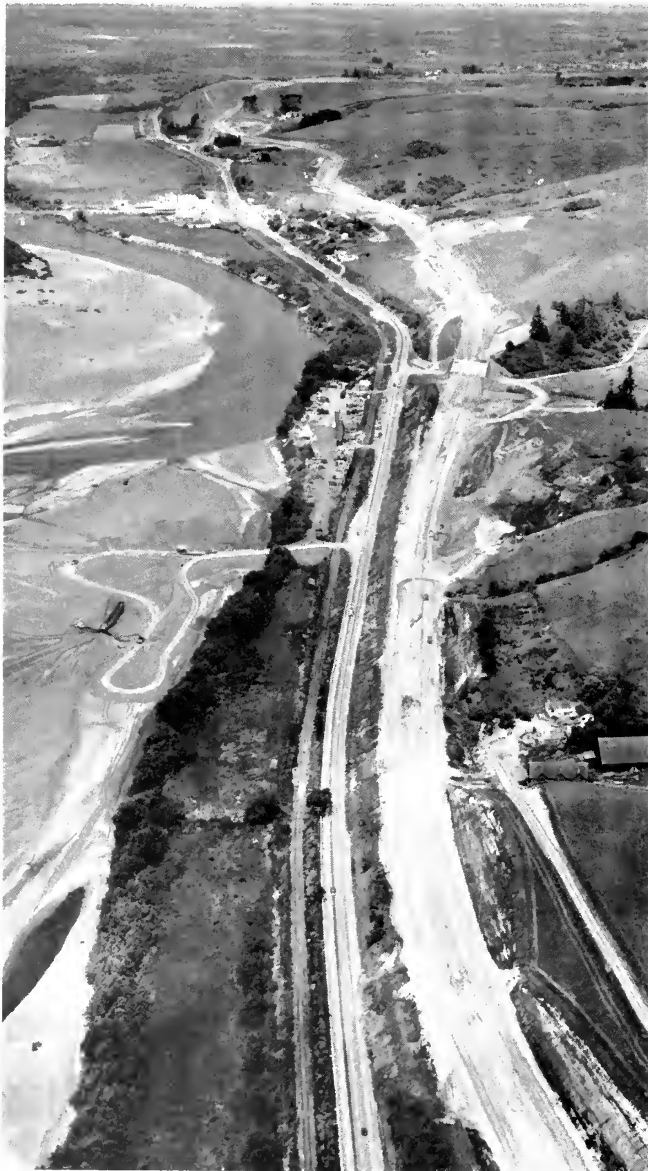
Looking north along the construction of the freeway on US 101 between Fortuna and one mile north of Fernbridge in Humboldt County.
