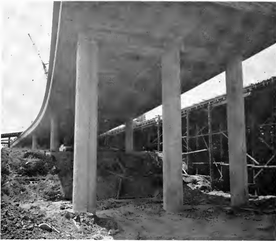
A view of the completed portion of the third level of the separation structure with falsework supporting the uncompleted portion (right).
