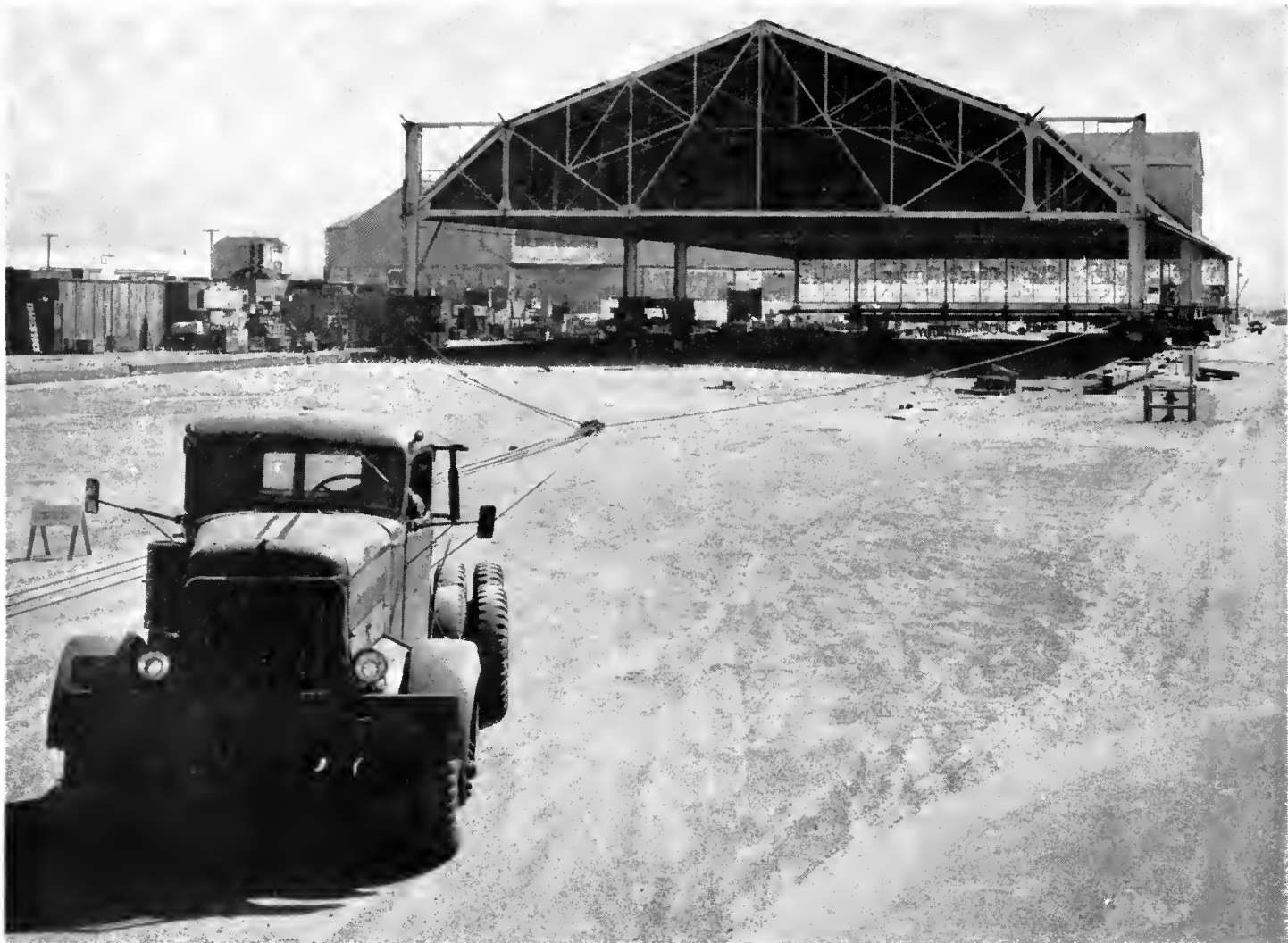
Hangar being moved. Nate black and tackle method. Projecting ends of H columns for bin frameworks may be seen beneath building.
