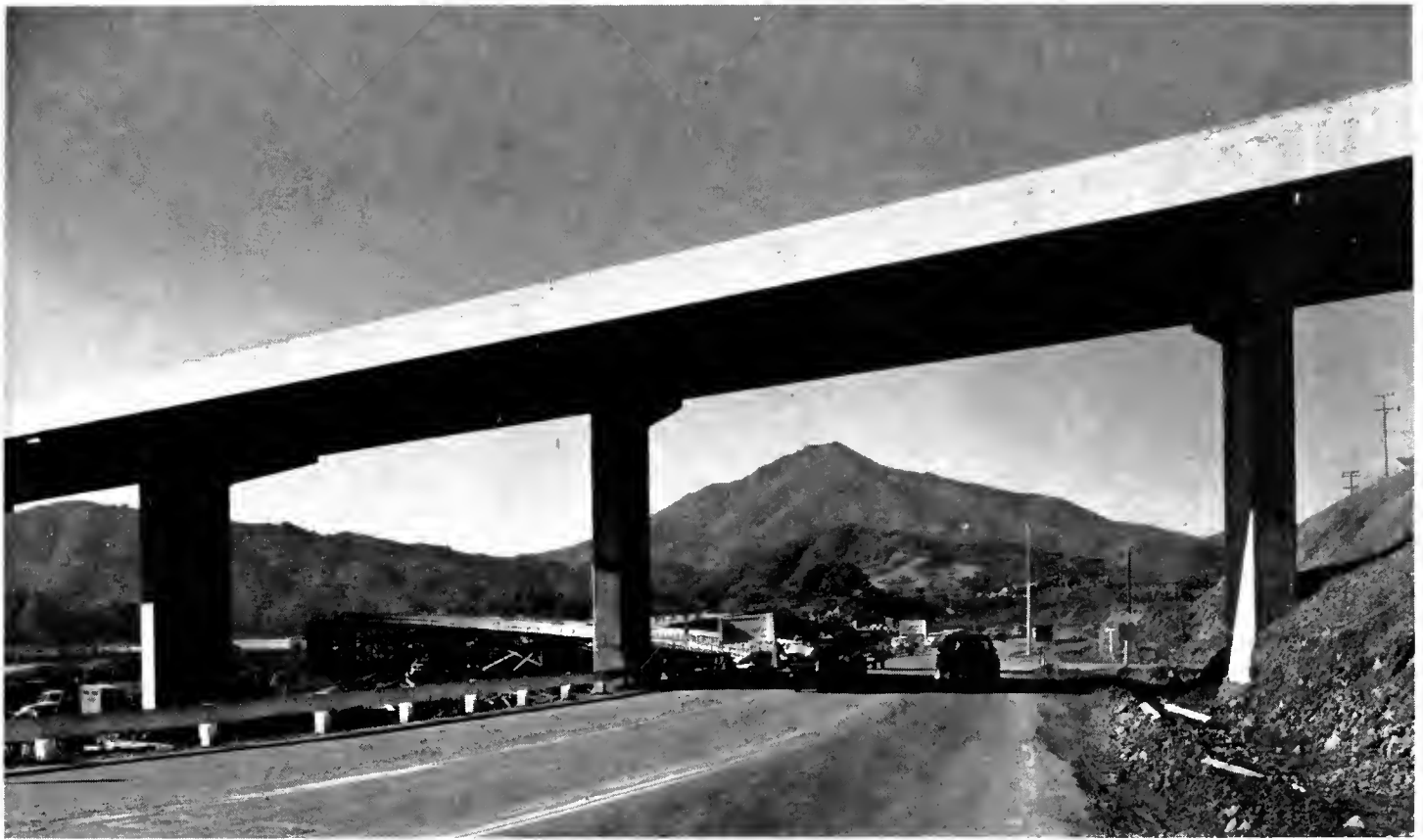
One of the bridges under construction at Corte Madero Creek on U. S. 101 in Marin County. The old bridge and lift span will be replaced by a new high level structure.
