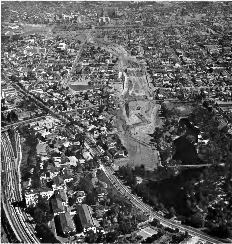
Construction on the Golden State Freeway is under way in the Boyle Heights area of East Los Angeles. Hollenbeck Park is in the right foreground; Los Angeles County General Hospital in the background.
