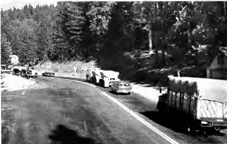
Reconstructed county road at Monte Vista provides detour around construction in this area.
