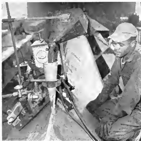
One of the heavy box section compression members being welded by the submerged arc process at one of the American Bridge fabricating plants.
