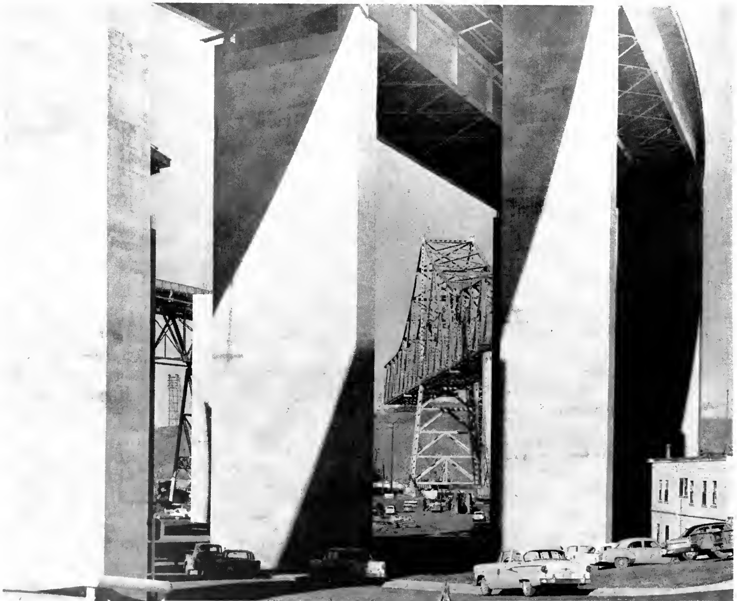
Construction is progressing on the parallel Carquinez Bridge which will connect with freeway sections now being built on US Highway 40 northeast of Oakland and through Vallejo. The bridge is one of several major projects which are under construction or budgeted on this interstate route between Oakland and the Nevada State Line. In view (center) between the giant piers which support approach roadways is a portion of the superstructure of the new bridge.
