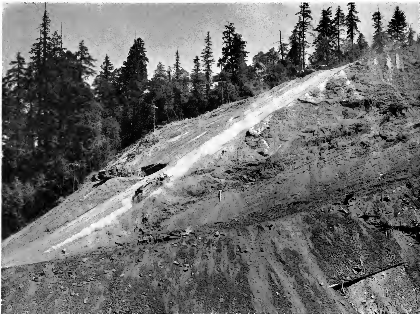
Equipment at work on the Big Cut. Steepness of the slope made it necessary to draw equipment to the top by the use of steel cable and winches.
