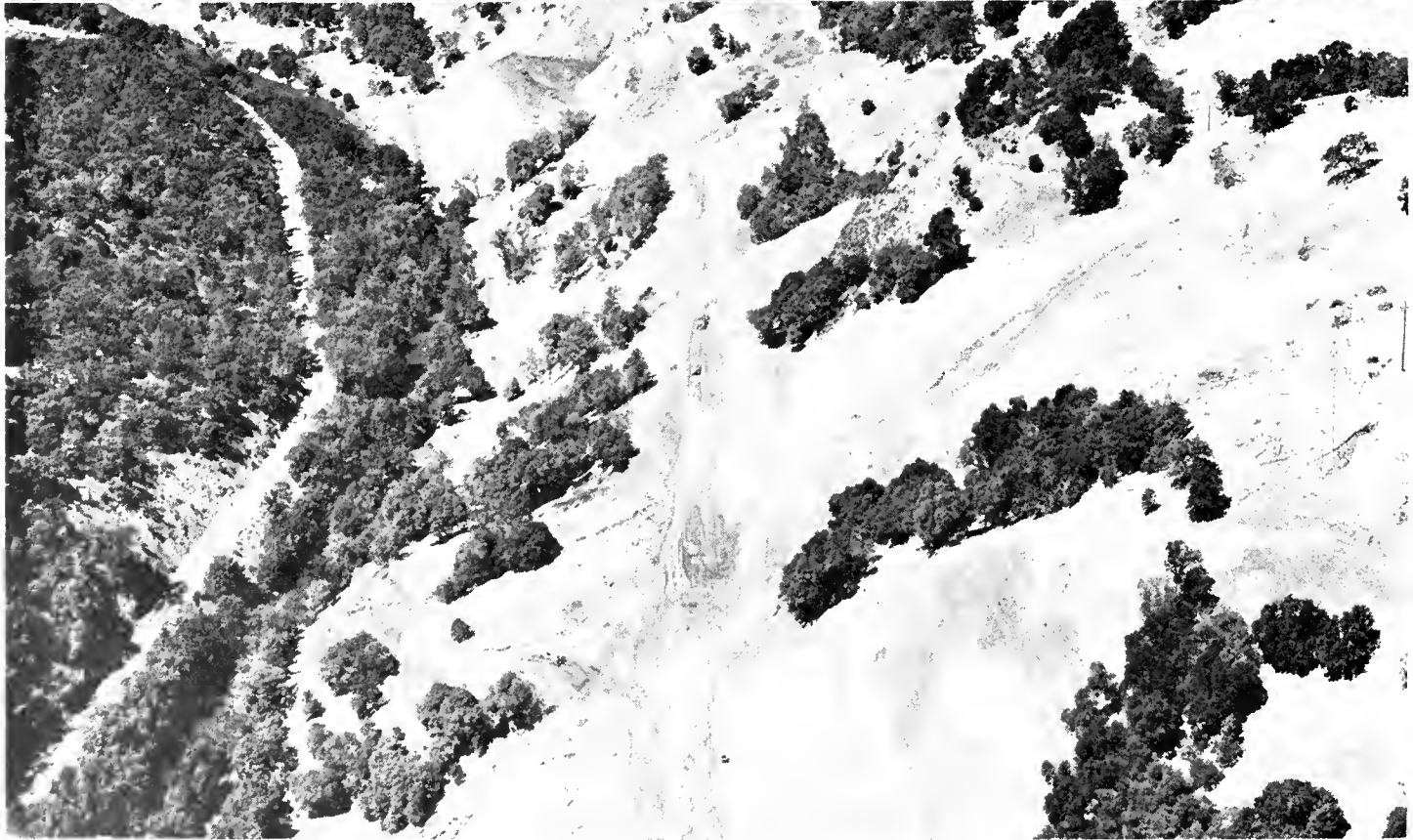
UPPER In Lake County, Sign Route 53 is being constructed as a modern two-lane freeway. This aerial is looking southward toward Clearlake Highlands and Clear Lake (right background). LOWER Heavy sidehill construction in the canyon of the East Branch of the Russian River in Mendocino County featured the relocation of Sign Route 20 between Colpella and Potter Valley Road.
