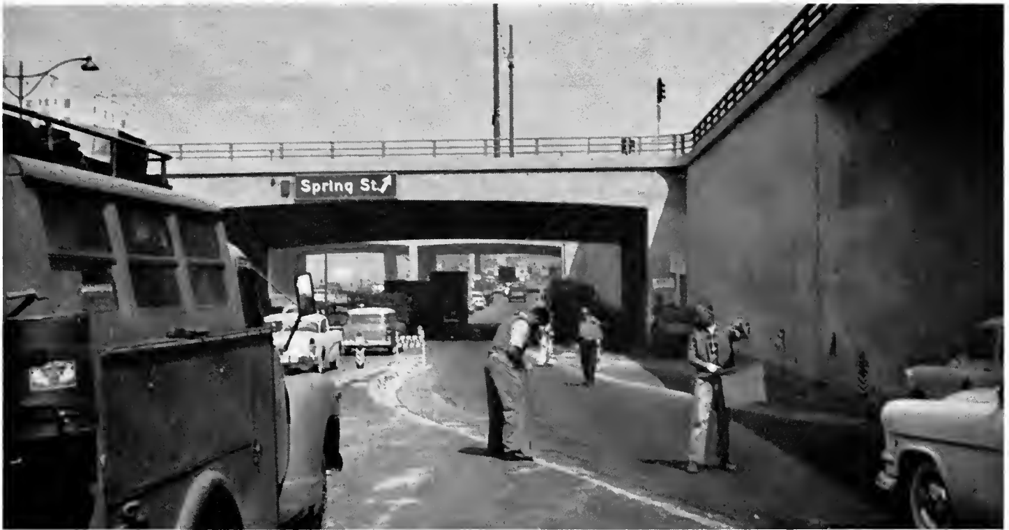
Traffic on a freeway inlet is temporarily stopped while surveying operations are in progress.
