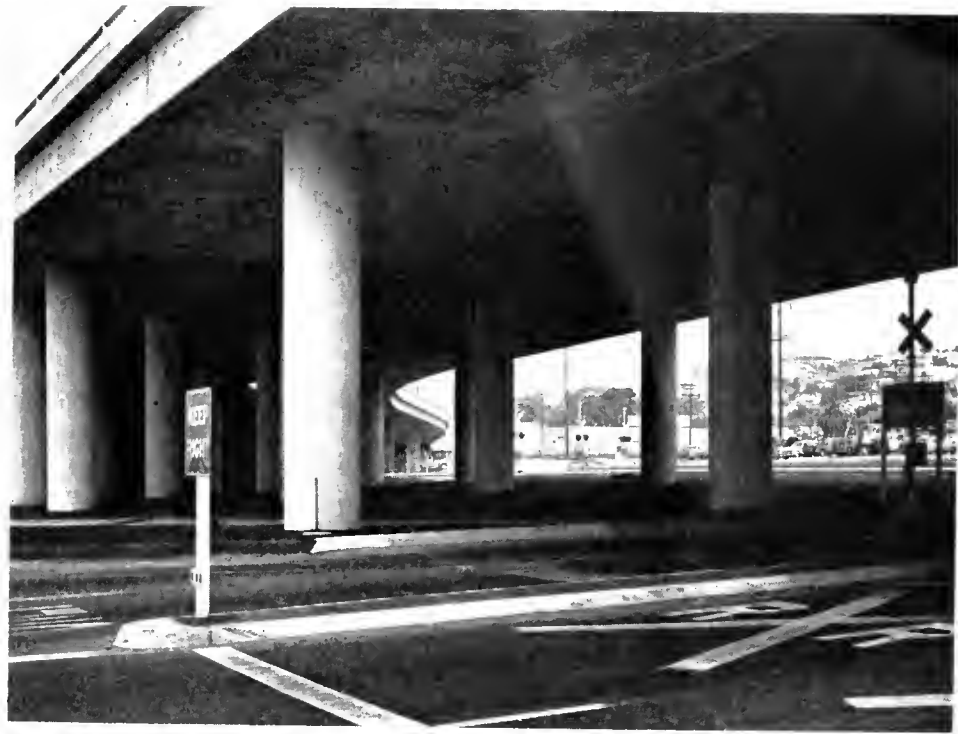
This picture was taken under the Washington Street interchange on US 101 in San Diego. The columns have been arranged to provide for a railroad wye as well as the highway.
