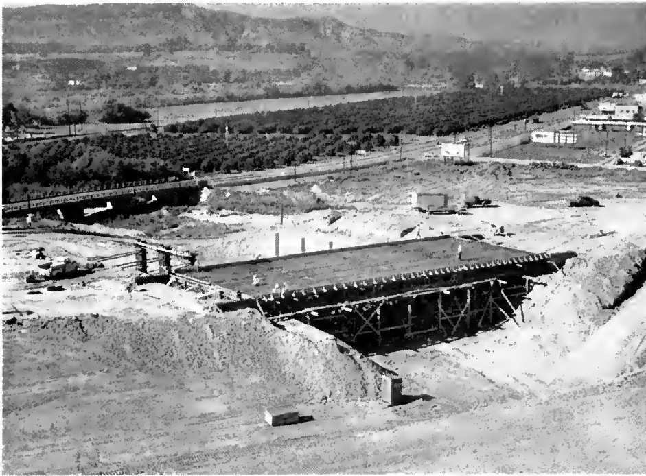
Overcrossing on the San Diego Freeway. This section of the freeway passes through San Juan Copistrano. It is 4.1 miles long and will be completed sometime during the fall of 1958 at a cost of $4,223,000.
