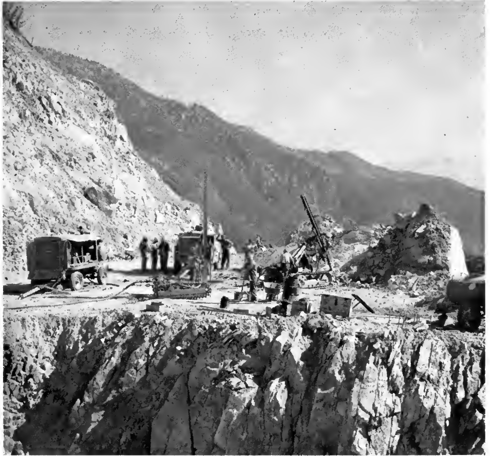
This photo of drilling operations on a section of Crystal Lake Road gives an idea of the ruggedness of the terrain.
