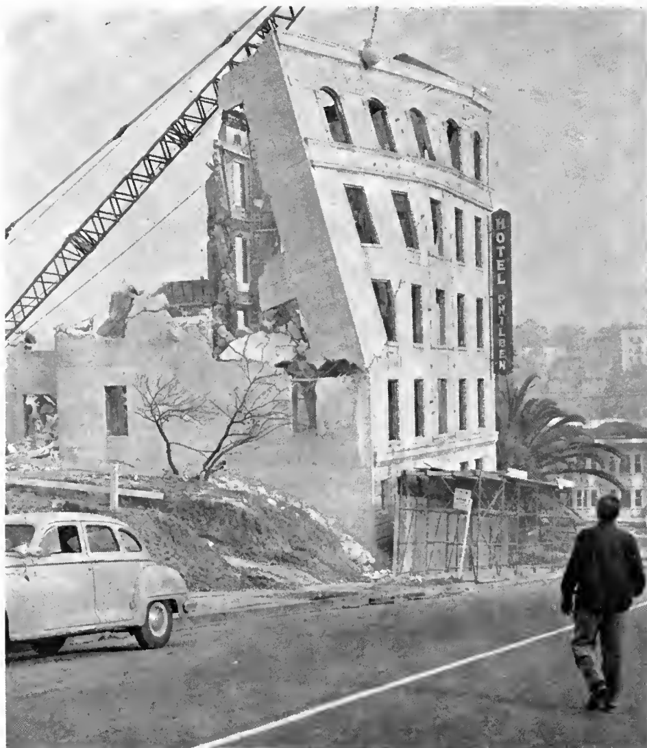
A 3,700-pound weight on the end of a long crane boom demolishes a concrete building to make way for a new freeway through downtown Los Angeles
