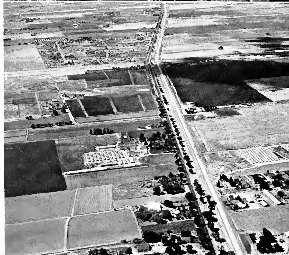
UPPER—This section of Sign Route 88 in Amador County near Jackson is being improved. The Town of Martell is in the distance. LOWER—An aerial showing the newly constructed southbound lanes to the right of a US 50 in San Joaquin County.
