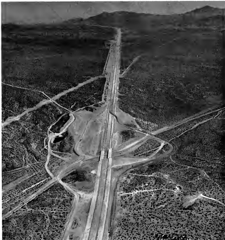
California highway construction is performed under contracts awarded on the basis of competitive bidding. The longest freeway ever built in California under one contract was opened in December, 1958. A portion of this 29-mile stretch of freeway on US Highway 91-66 between Victorville and Barstow is shown above during construction.
