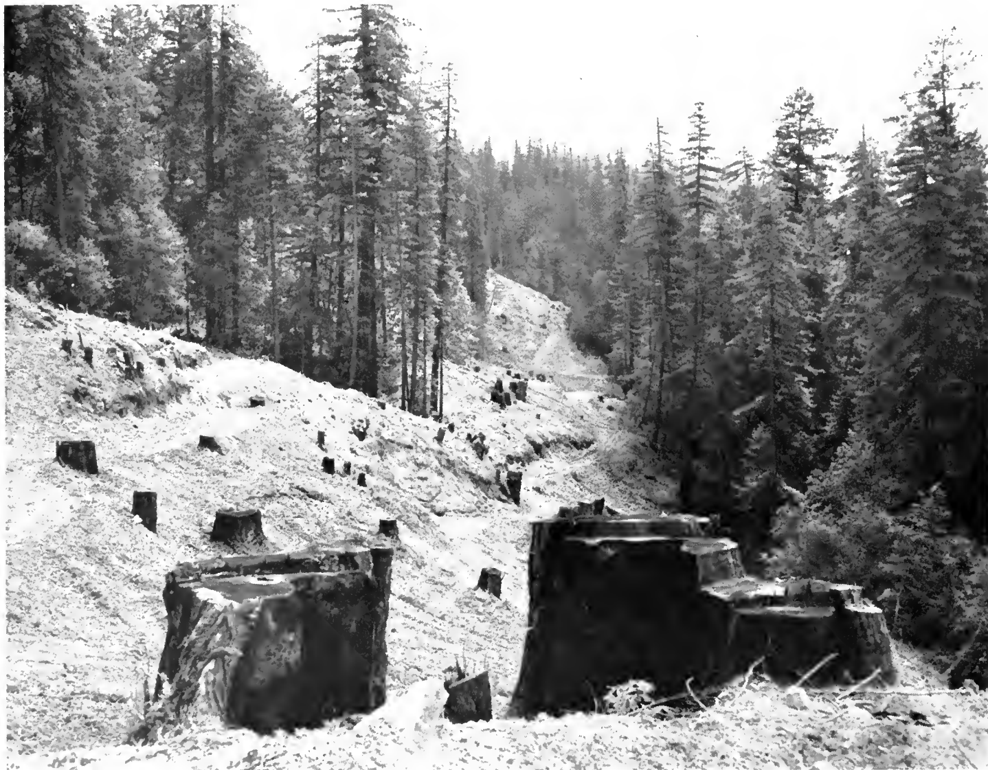
A cleared area prior to grading operations on the second unit of the Redwood Parks Freeway (US 101) between Myers and Dyerville in Humboldt County.
