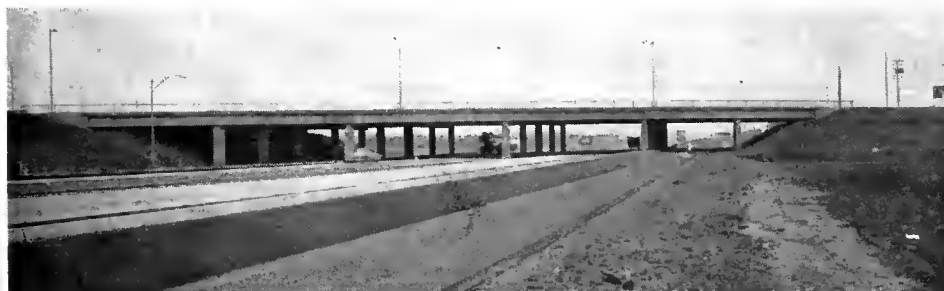
Separation structures such as this on the Eastshore Freeway are typical of the State's freeway construction program
