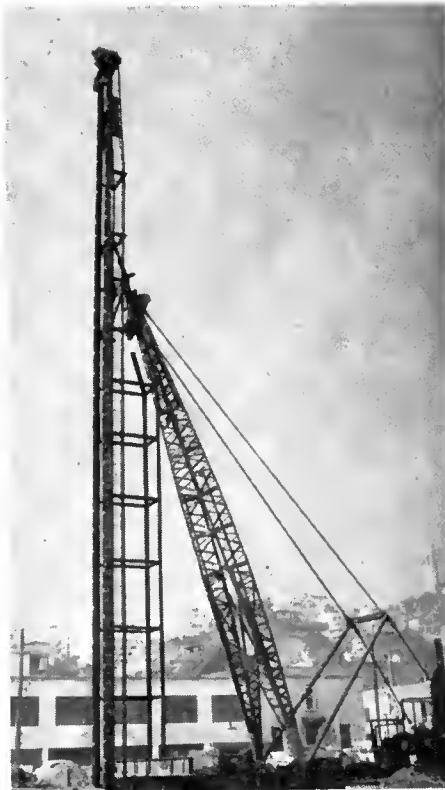
Quiet Myrt, one of the piledrivers used on the job, as it was being assembled.
