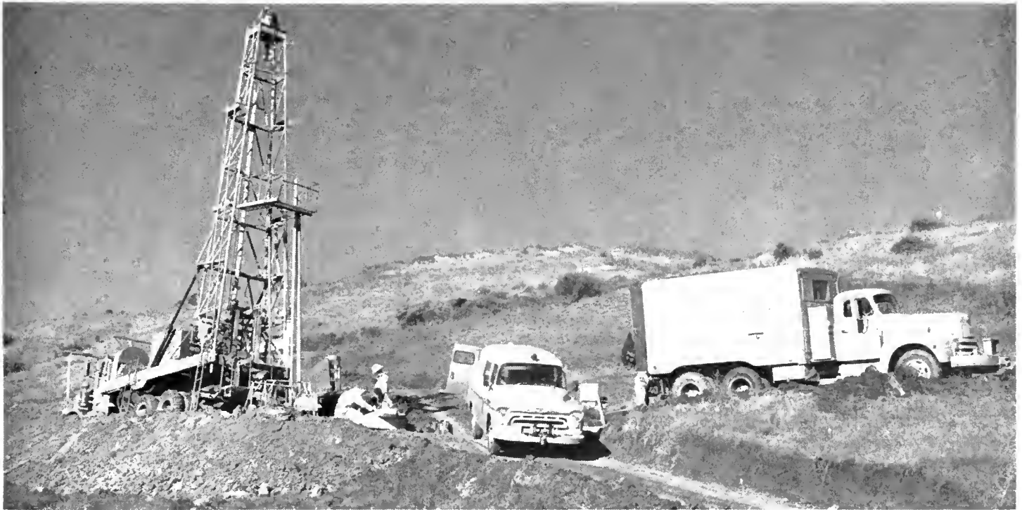
Large drill rig in position for making deep borings in a landslide area. Undisturbed samples can be obtained with this equipment with a drive-type sampler or a rotary type core barrel. Cores have been taken with this machine from depths in excess of 300 feet.
