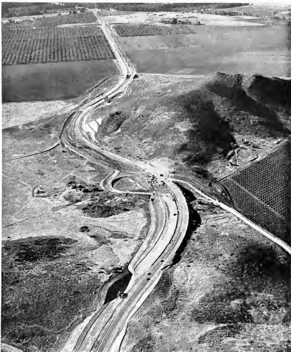
Looking west along Ventura Freeway construction showing Conejo Grade in the foreground
