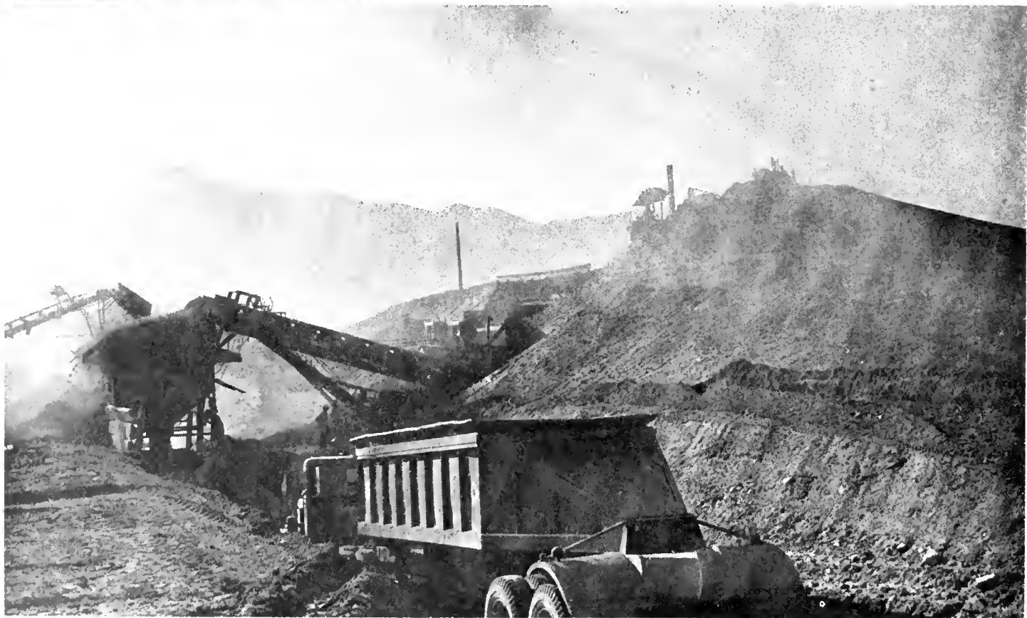
UPPER - Trucks wait in line on the Victorville-Barstow job and then (LOWER) they are loaded at the Wild Wash base material plant
