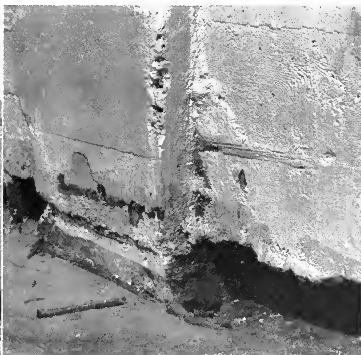
Floor actually sank beneath foundation footings in places. Pile cap is almost exposed at this point.
