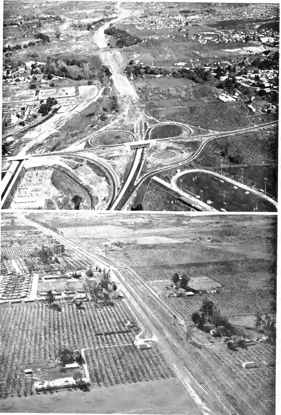
UPPER—The new freeway under construction between San Jose and Las Gatos (Sign Route 17). Saratoga Avenue Interchange in Las Gatos is in the foreground. LOWER—Sign Route 29 north of Napa. Construction of an additional two lanes converted this section into a four-lane expressway between Union Station and Orchard Avenue.
