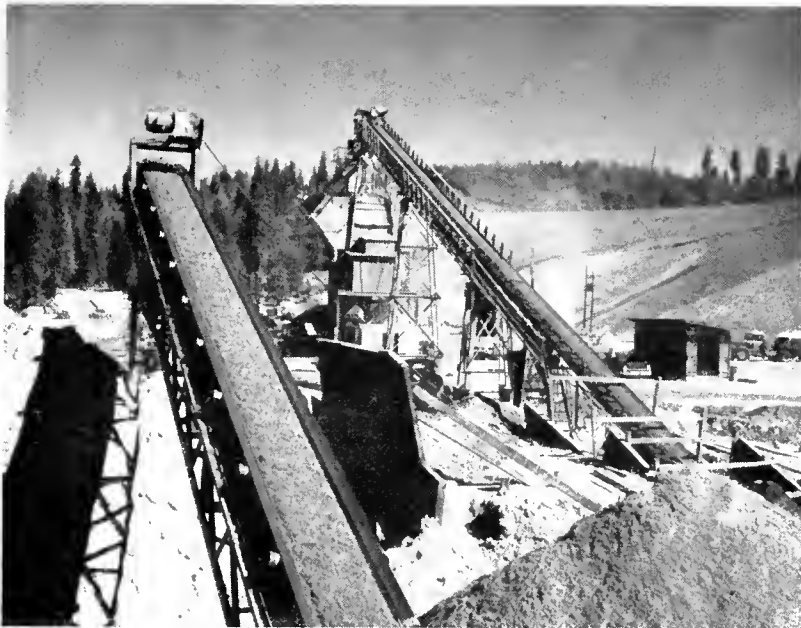
Batch plant in operation near Baxter. This is site for new Whitmore Maintenance Station. Old highway extreme left, new route on fill upper right.
