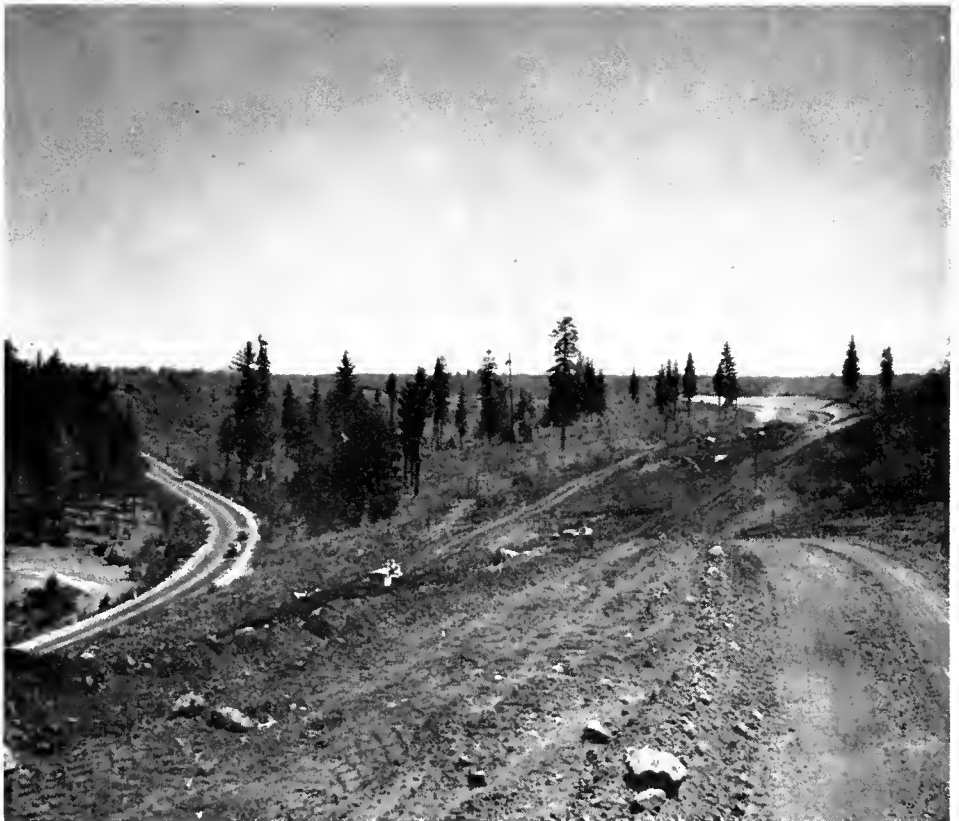
UPPER—Work progresses on the new Yuba River Bridge at the south city limits of Marysville on U. S. Highway 99E. LOWER—A view of freeway construction looking eastward from near the foot of Airpart Hill in Placer County. Present US 40 (left) will serve as the westbound lane of the new freeway. The eastbound lane is under construction (right).
