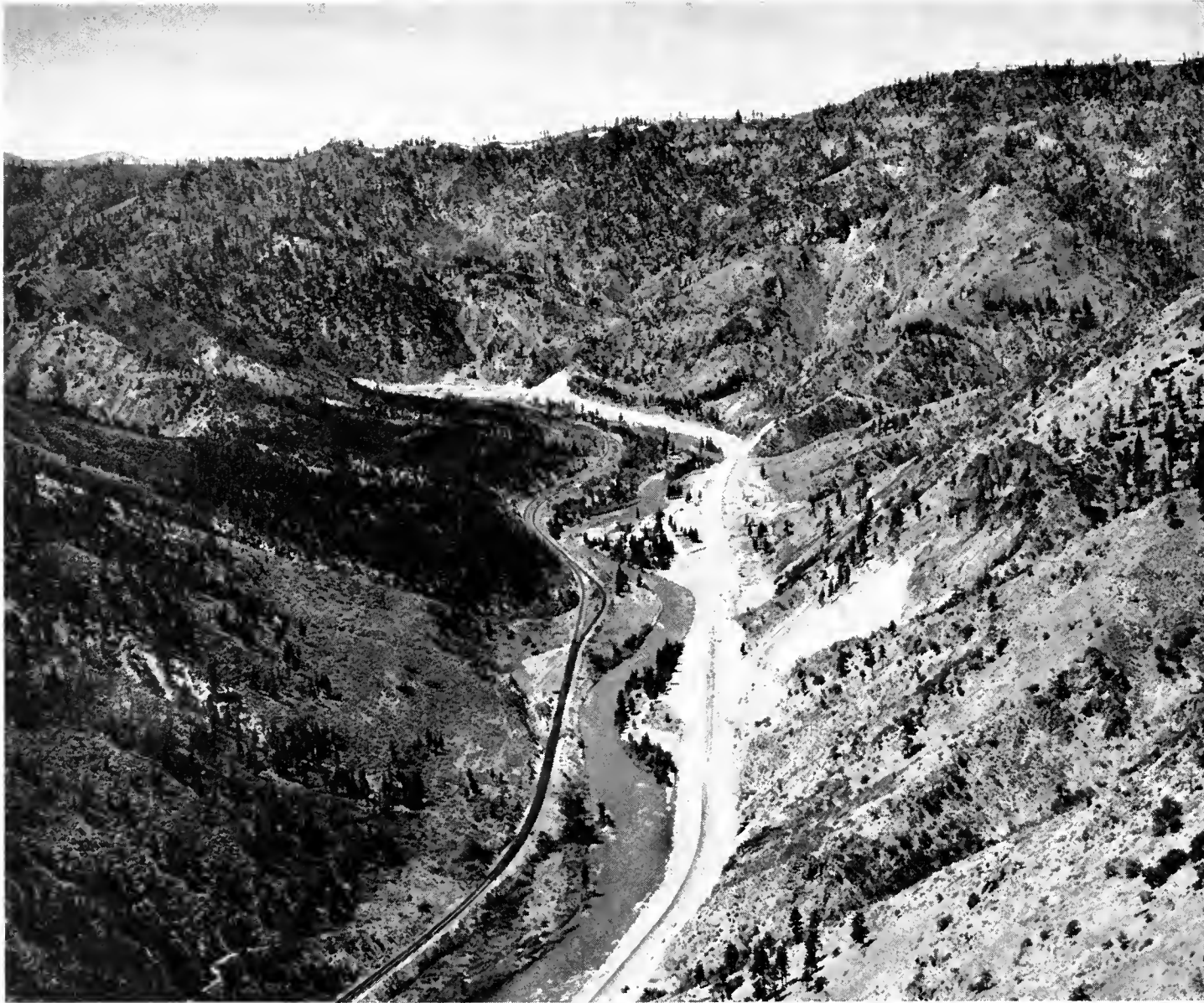
This photo shows paving operations in progress on the US 40 freeway in the Truckee River Canyon between Floriston and the Nevada state line. It is scheduled for completion this summer.
