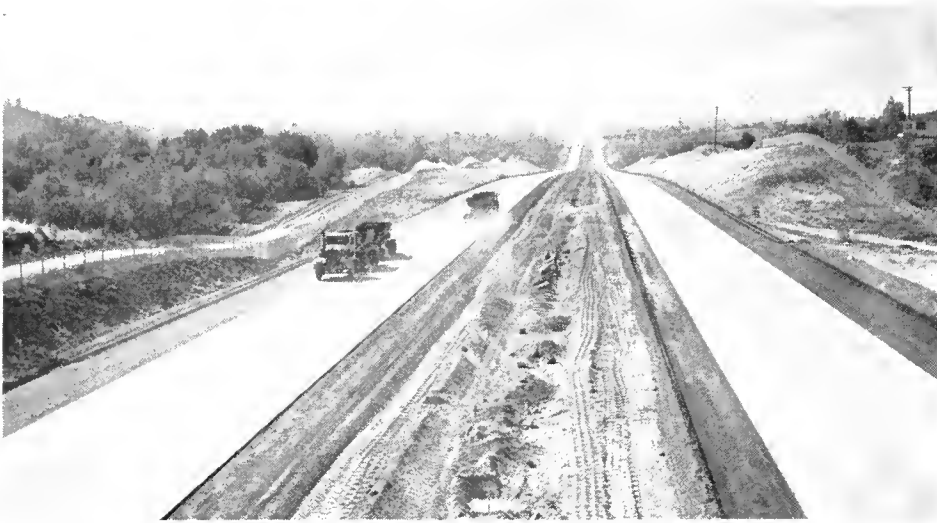
Looking west on US 40 a few miles above Roseville on the new section between that city and Newcastle.
