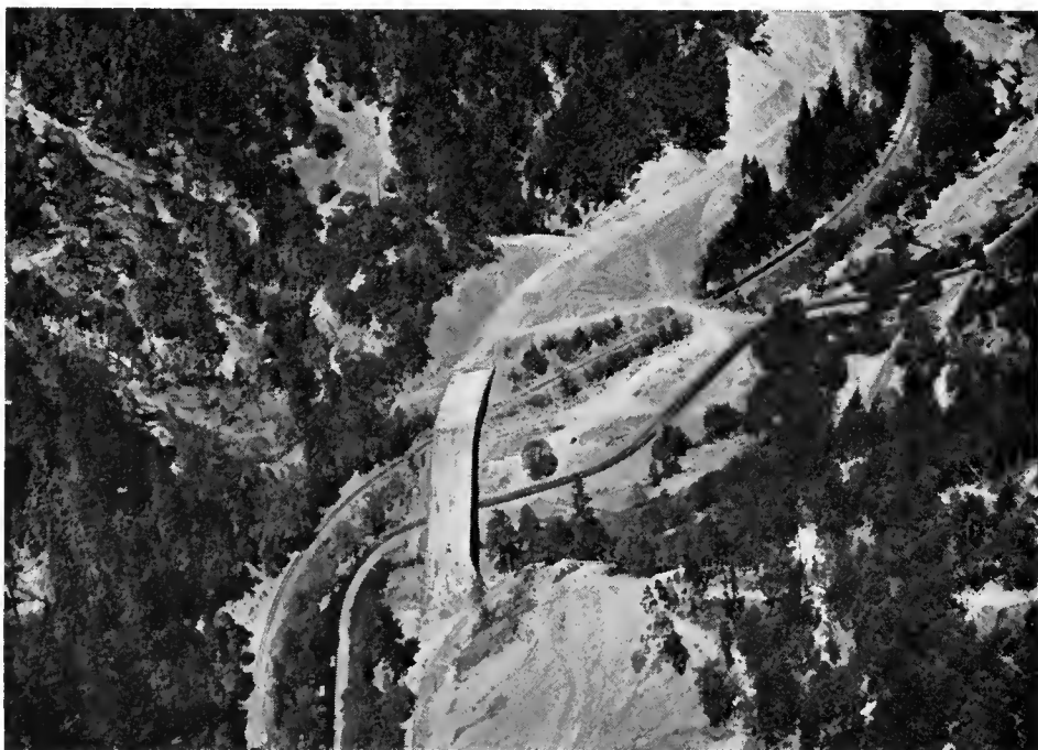
This four-lane structure over Outlet Creek and the Northwestern Pacific Railroad is part of the US 101 freeway construction north of Willits.
