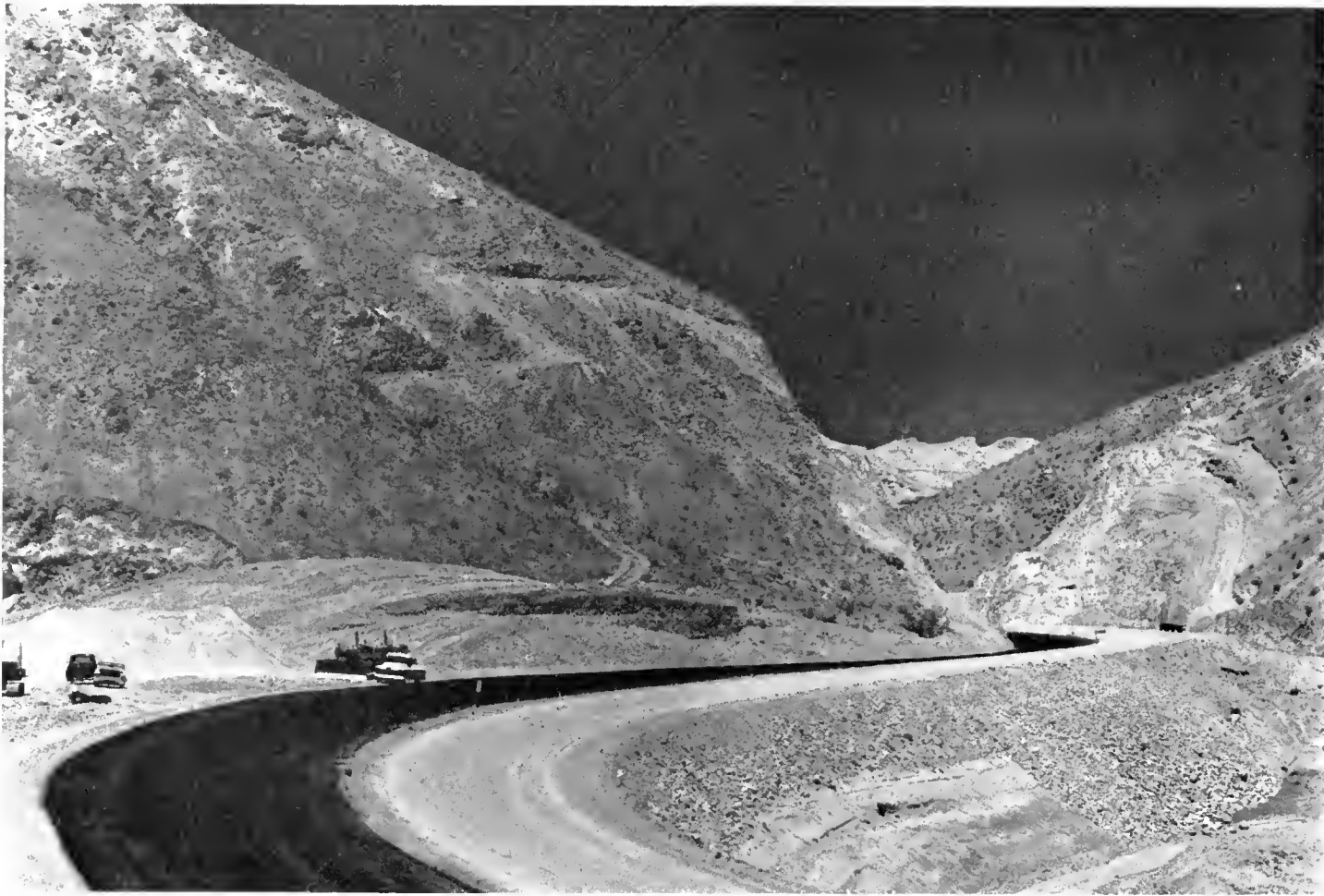
New four-lane expressway construction in Red Rock Canyon north of Mojave on US 6. The high rock cut and channel excavation on the right were necessary to make room for the highway and flood channel in the canyon.
