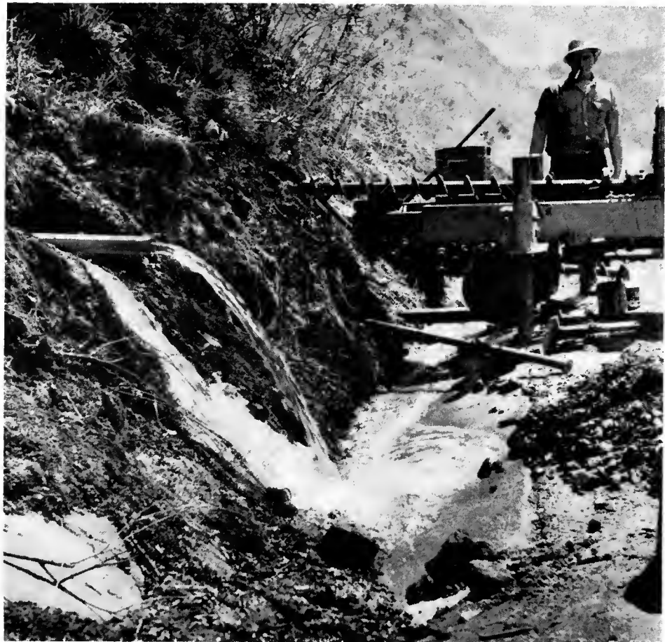
Completed horizontal drain in foreground and boring being made for another drain on a recently completed horizontal drain installation in San Luis Obispo County
