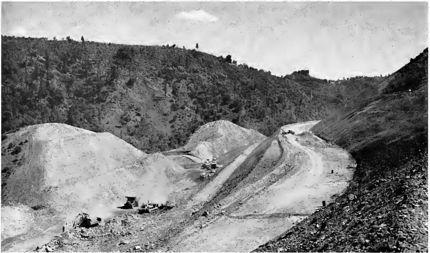
This photo taken two miles east of Cherokee in Butte County shows some of the heavy grading work involved in the construction of US 40 Alternate.
