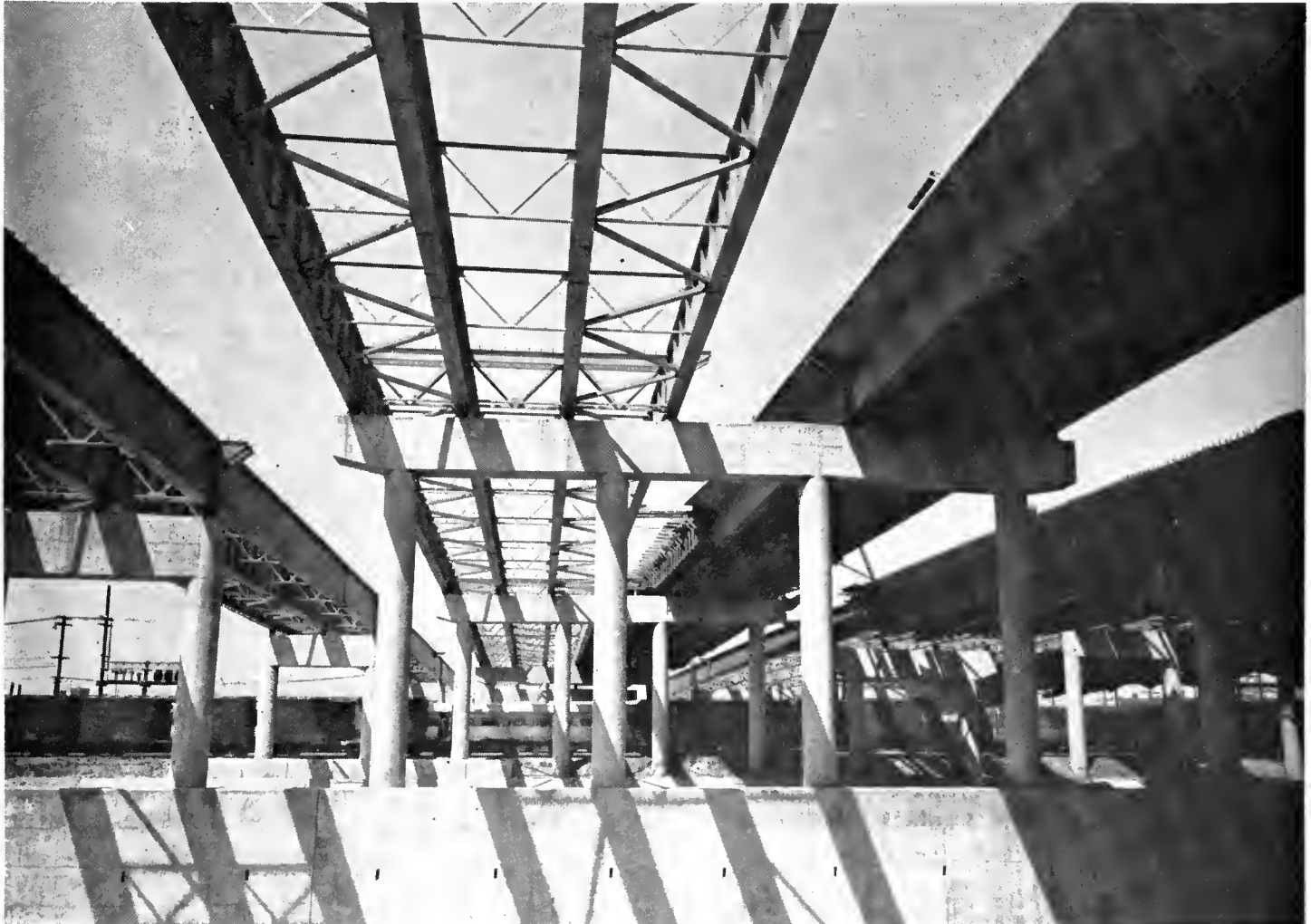
This view westward of the bridge construction was taken under the main eastbound roadways. There will be a total of six parallel structures with a combined width of 14 traffic lanes.
