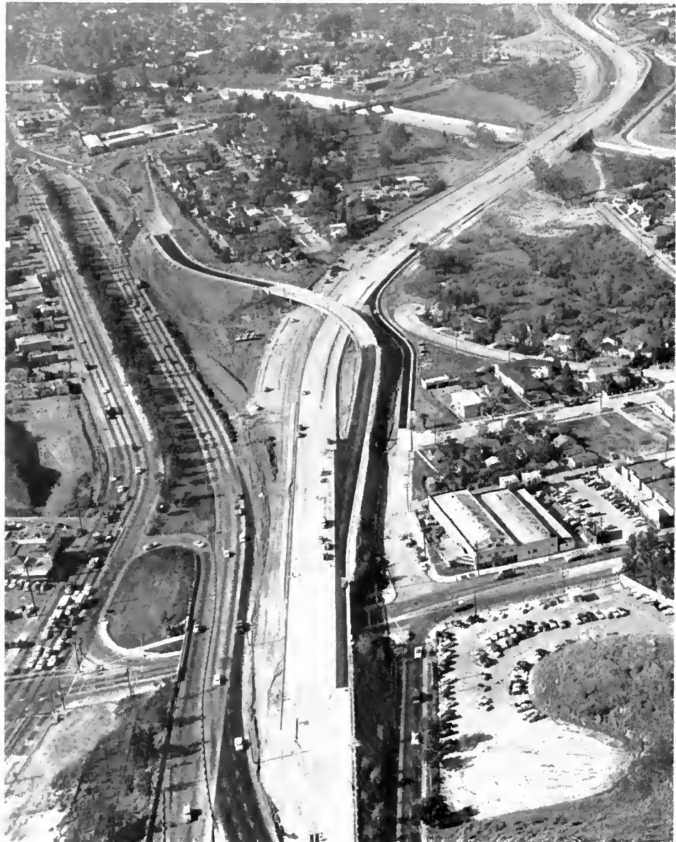
Looking northwest along Hollywood Freeway Extension. Lankershim Boulevard is in foreground. During construction traffic uses inbound lanes of Hollywood Freeway and Venturo Boulevard to left.
