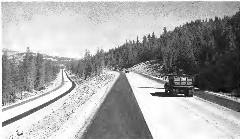
Hampshire Racks to Soda Springs portion just before completion while crews were completing asphalt shoulders.
