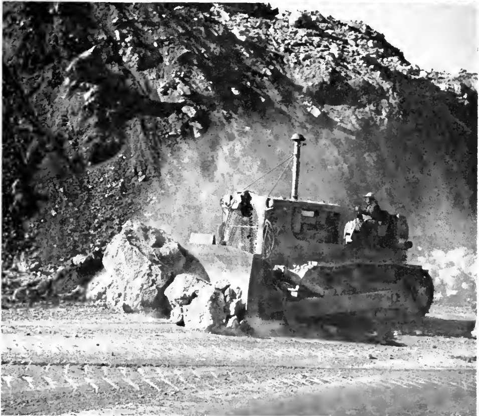
UPPER—Section of a cut taken just after a blast. The larger boulders will have to undergo secondary blasting operations before they can be hauled away. LOWER—A tractor clears boulders from the roadway shortly after a blast.
