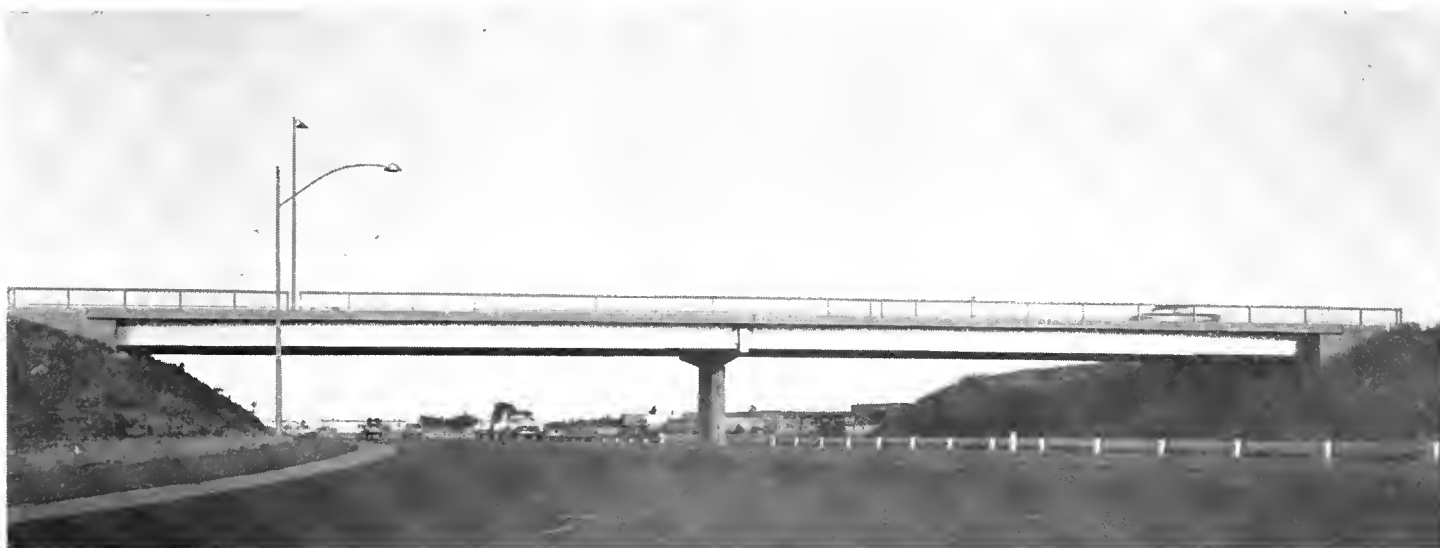
Honorable mention winner in the Class III Division for Bridges with spans less than 400 feet long and costing less than $500,000 was the Marsh Road Overcrossing south of Redwood City on the Bayshore Freeway.
