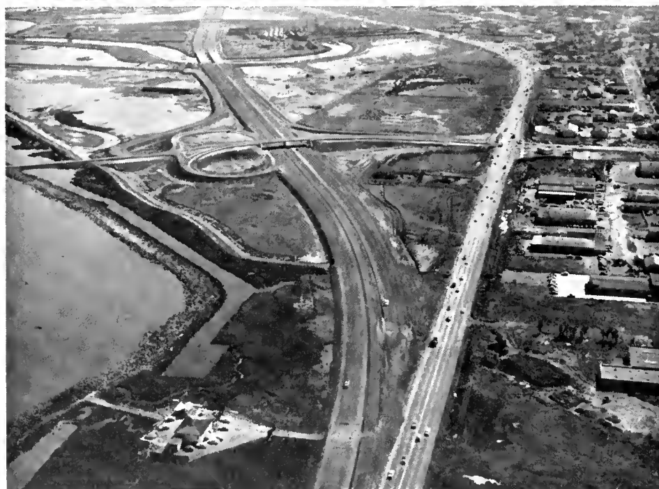
UPPER—Freeway construction on the Boyshore Freeway looking north from the Son Moteo-Santa Clara County line. LOWER—Construction on the Bayshore Freeway in Redwood City. The present highway is on the right. The Whipple Avenue Interchange is on the new freeway to the left.
