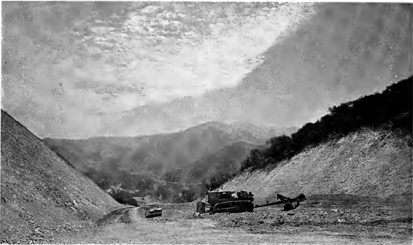
Relocation of Sign Route 166 because of the construction of Twitchell Dam and eventual flooding of the present highway by the reservoir has required several large cuts and fills through rugged mountain terrain
