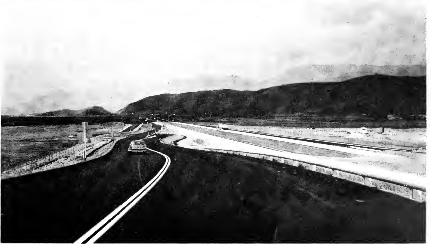
Two photos of recent construction of the San Bernardino Freeway show (upper) the new freeway looking south from the San Bernardino city limits and (lower) looking north from the vicinity of Highland Avenue.
