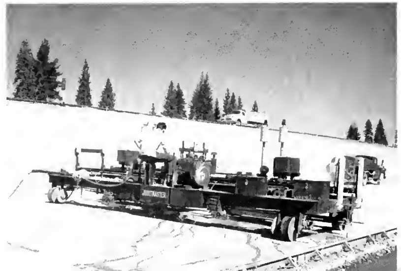
Concrete saw cutting joints in new pavement near Soda Springs. Old highway is on level above.
