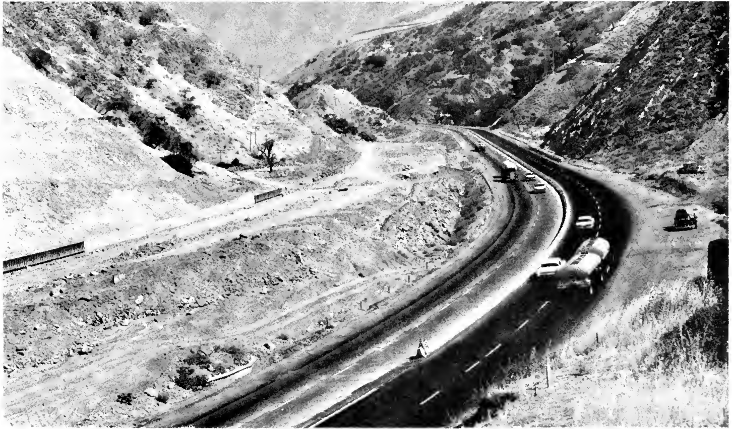
UPPER—Shoulder construction on the US 99 resurfacing project in Madera County. LOWER—A view southward of freeway construction in the Grapevine Grade (US 99).
