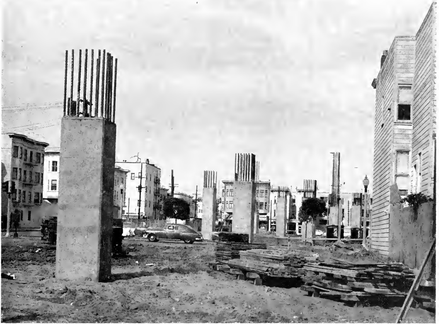
Construction on the Central Freeway (U. S. 101) in San Francisco. The piers will support a double-deck traffic structure. Right-of-way needed is reduced to a minimum by double-deck design.
