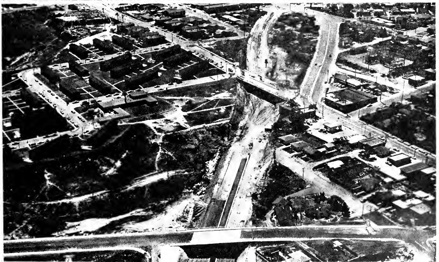
UPPER- This aerial, looking westward, shows the US 395 Clairmont Mesa Interchange in San Diego County. LOWER An aerial showing construction along Nimitz Boulevard in San Diego. The view is south.
