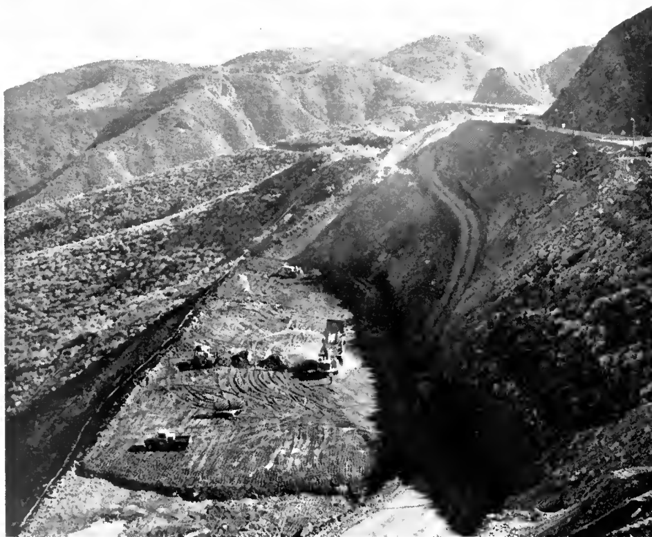
UPPER—Heavy equipment moves blasted material from a cut. LOWER—Grading operations in progress near the summit. The embankment under construction in the foreground will contain a total of half a million cubic yards of material when completed.
