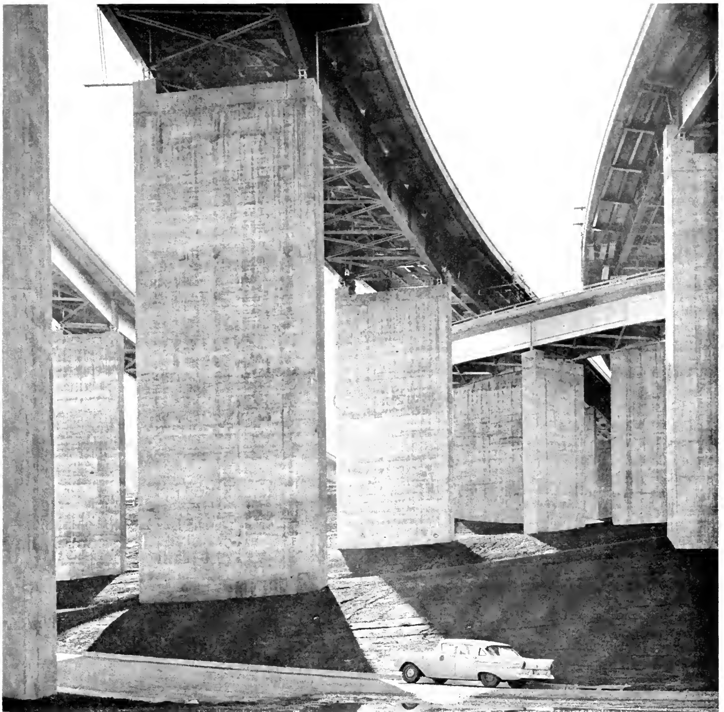
The interchange structure as seen from the streets of Crockett. Each of these pier shafts took only one week to construct. Slip-forms and modern bridge construction techniques made this speed possible.
