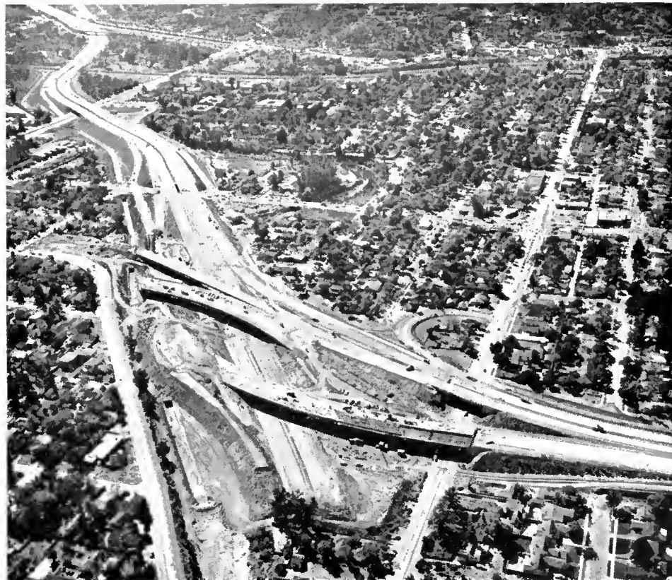
UPPER—An aerial view eastward showing the Ortego Highway interchange crossing over the San Diego Freeway (right). The buildings in the middle ground are the San Juan Capistrano Mission. LOWER—Construction is now under way on the Ventura Freeway-Hollywood Freeway interchange. This view southward shows the northern end of the Hollywood Freeway.
