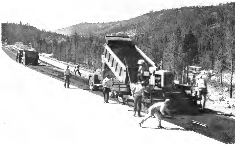
Contractor's crews finishing asphalt shoulder on Hampshire Racks to Soda Springs section.
