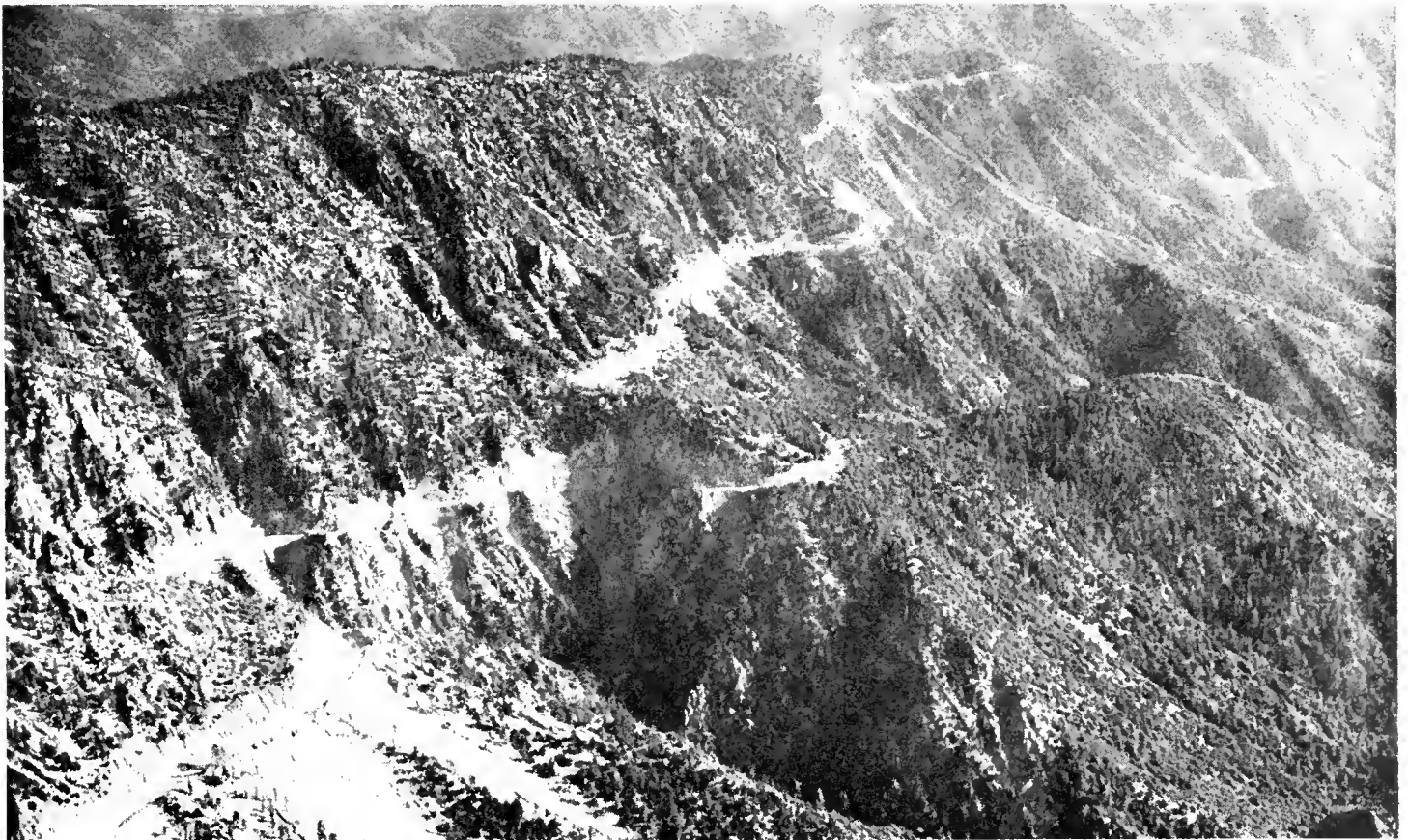
UPPER—Another view of the rugged terrain through which the road is being constructed. LOWER—An aerial showing the alignment of the road. Note the dust cloud in the background where the construction is going on.
