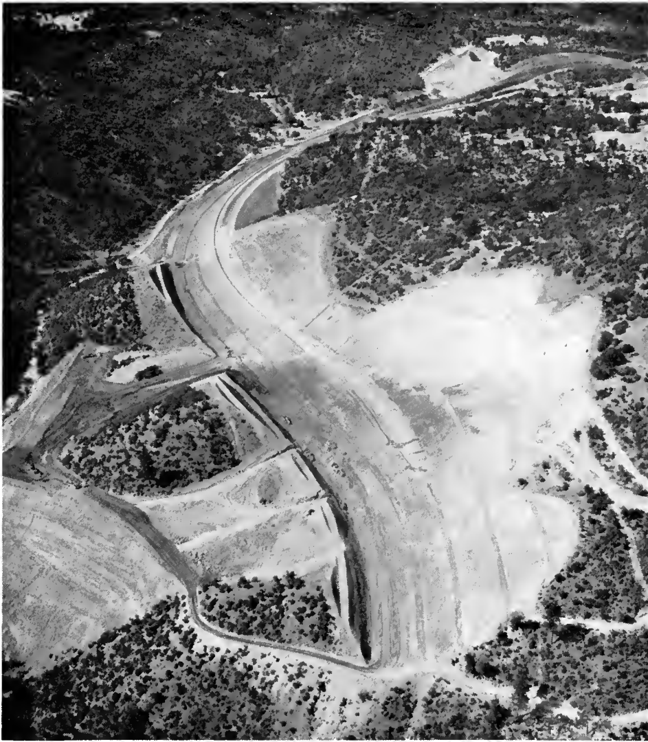
This large benched cut on US 40 Alternate in Butte County is located just south of the future location of the new West Branch Bridge.
