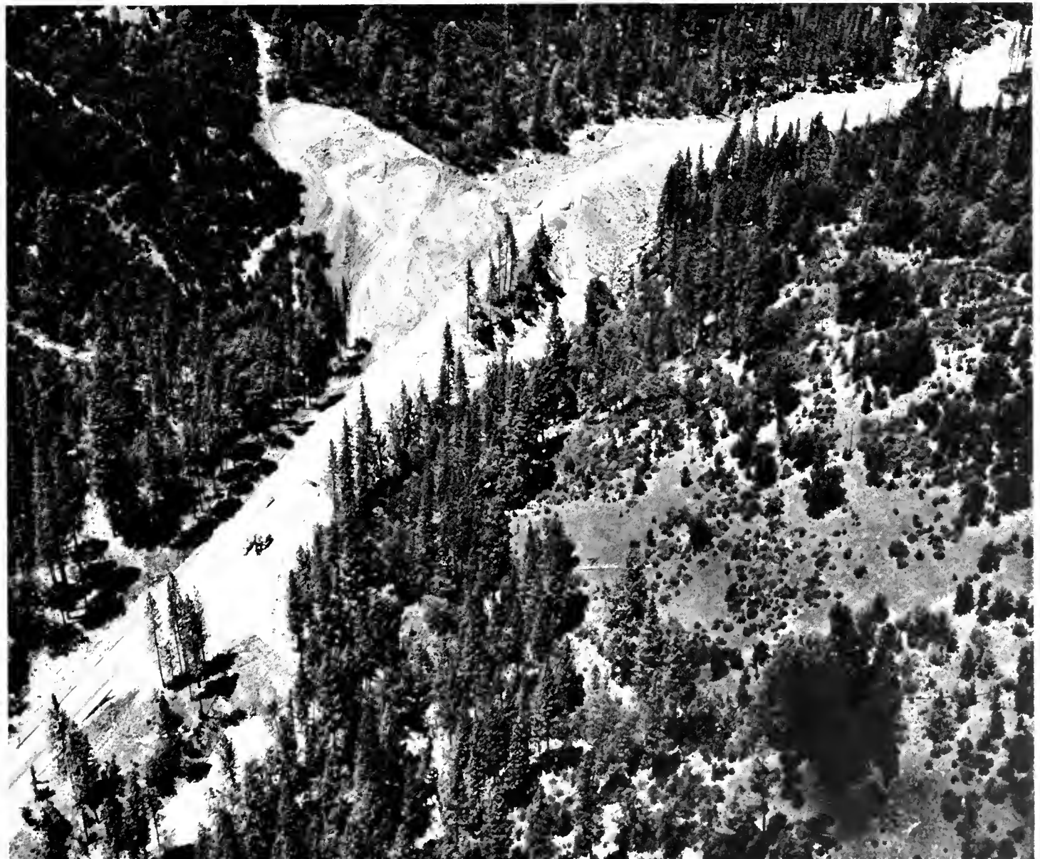
Construction on the Yosemite All-year Highway (Sign Route 140) eight miles north of Mariposa is improving this important recreation route
