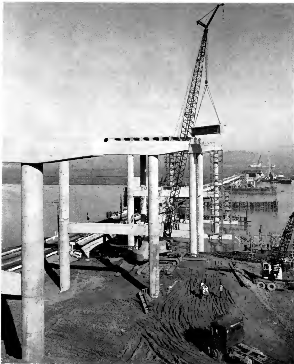
This view, taken from the west abutment fill, shows a crane with a 120-foot boom setting one of the 12-ton, 25-foot-long girders in place
