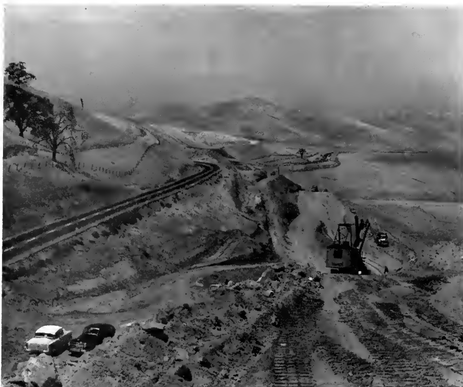
Shown here are some of the US 466 relocation operations now going on east of Bakersfield. The present highway is to the left.
