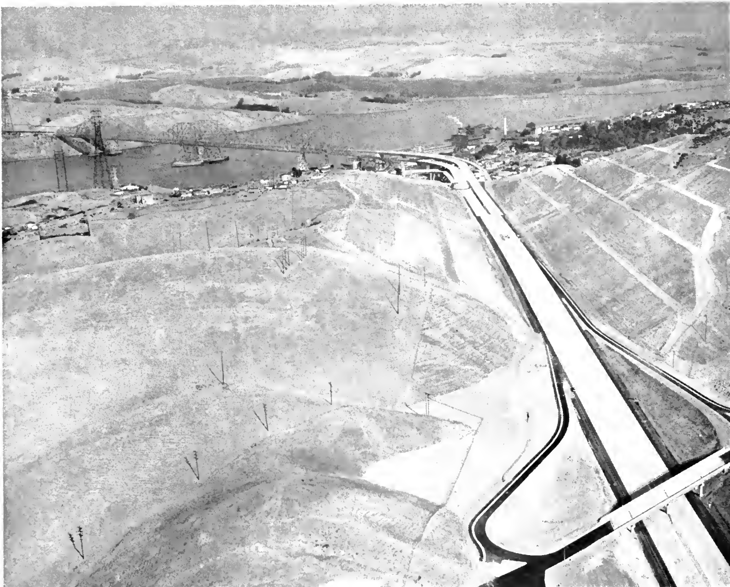
Picture showing the "Big Cut" completed with the Corcuinez Bridge in the background. To the right can be seen the 30-foot benches spaced every 60 feet in elevation going up the side of the cut. Slope of cut between benches is 2:1; that is one foot up for every two feet horizontal.
