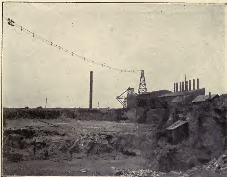
FIG. 75.—Cableway in cement-rock quarry.
