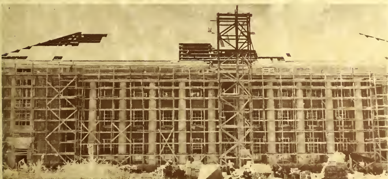
The Science Building, shown underway in 1949, was the first major post-war project. It now bears the name Mickle Hall.
