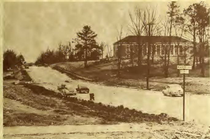
With the construction of Mickle Hall, the campus turned its face toward Woodlawn Avenue and began to take on an entirely new aspect.
