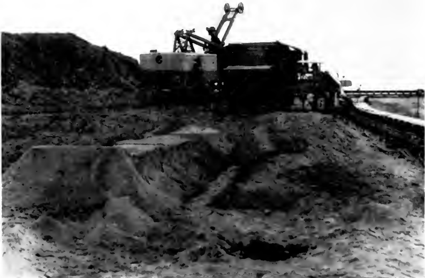
Two of the highly mechanized iron-ore mining operations are dredging (top) and movement of the ore on a conveyor belt (bottom). (Fig. 6)
