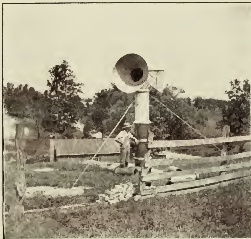
Eighteen-inch cowl to sub-earth duct at B. B. Herriek's factory, Wellington, O. The duct runs down a hill and the factory is seen at the foot of the hill.
