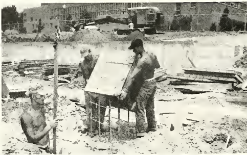
Workmen broiled in the hot sun as work got under way on constructing a new stand for the football stadium.
