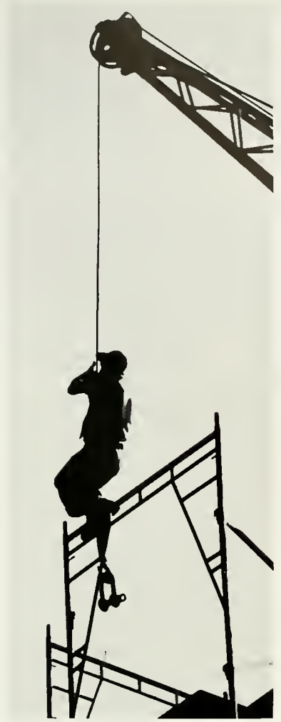
Work is in progress for the completion of Lake and Olsen men's dorms, opening in the fall.
