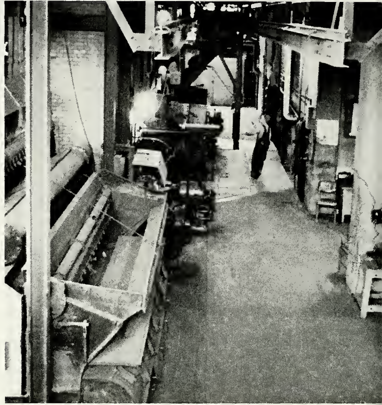
A camera's-eye view of a part of the vast machinery housed in the heating plant.
