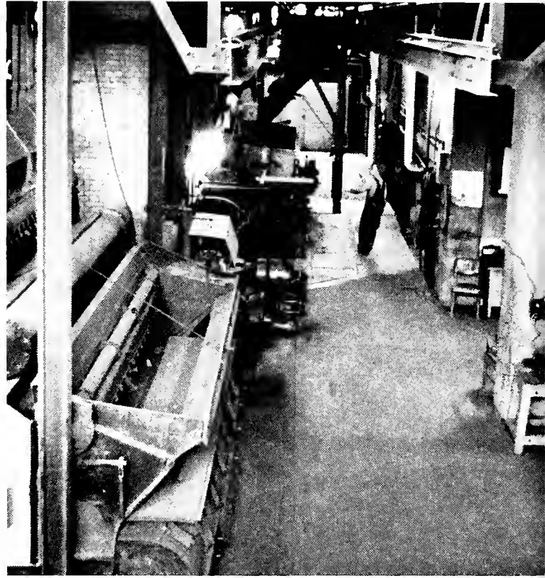
A camera's-eye view of a part of the vast machinery housed in the heating plant.
