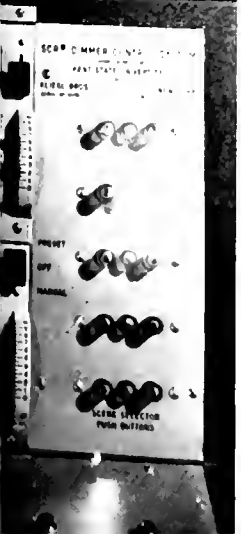
From this panel are produced the stage lighting and special effects for the E. Turner Stump Memorial Theater
