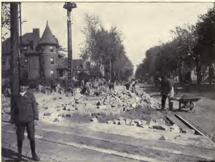
Setting Medina sand-stone blocks on six-inch concrete base covered with one and one-half inches to two inches of sand-cushion.
