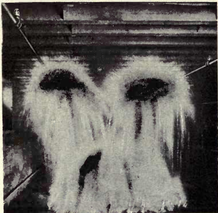
These sprinkler heads opened very soon after a small fire was started on the floor and the fire was quickly extinguished.
