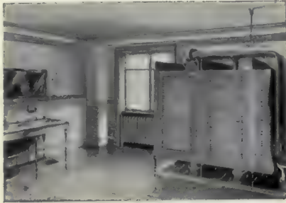
"Sirocco" neatly installed in Public Comfort Station.
