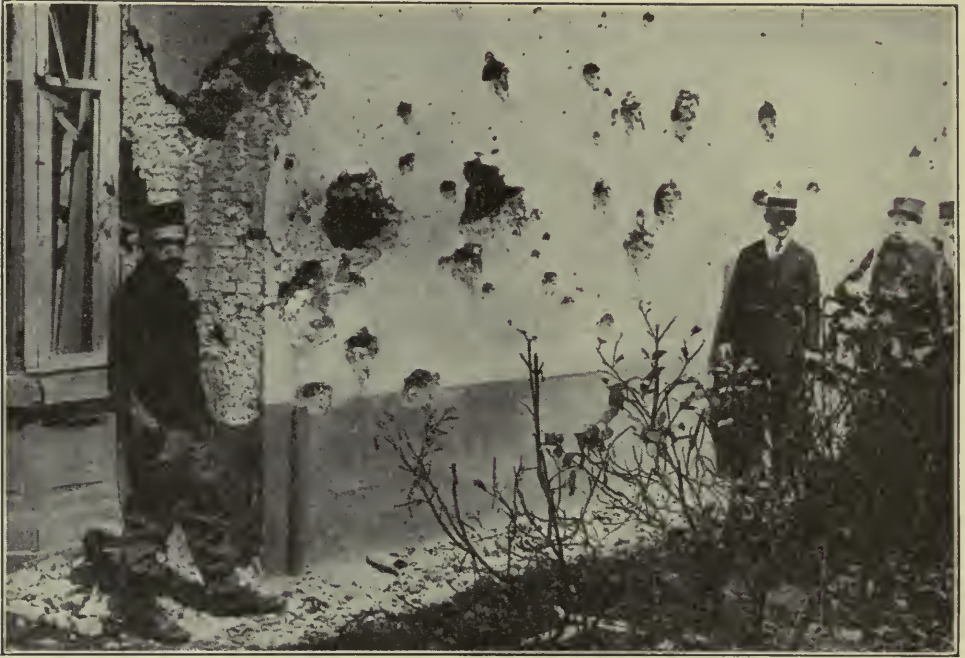
Wall of House Ten Yards from Where Bomb Struck Pierced by Fragments
