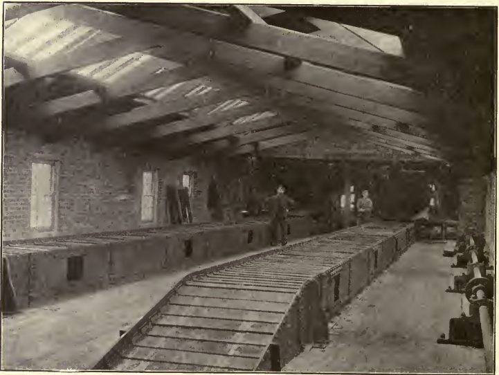
FIG. 36.—Plant constructed for the Cramlington Coal Co., Northumberland, and arranged to screen and pick 800 tons per day.
