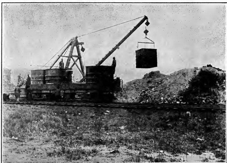
FIG. 14.—METHOD OF DISCHARGING ASH BINS, BROOKLYN.
