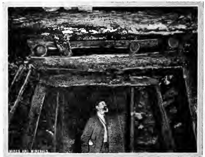
FIG. 4. TIMBERS AND LAGGING SHOWING FUNGUS GROWTH
