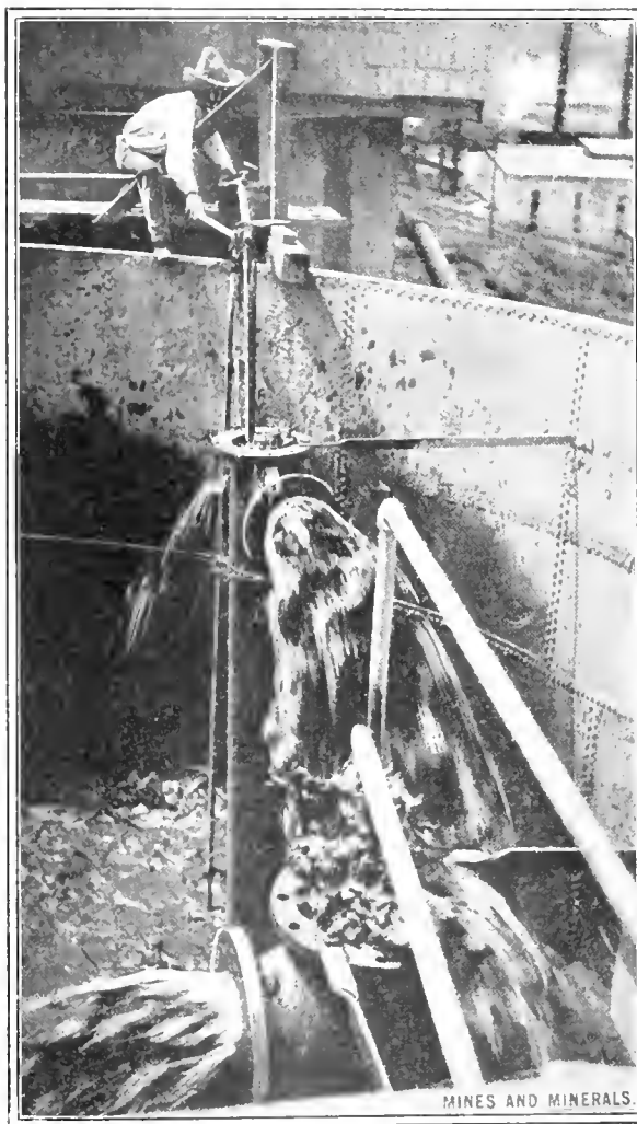
FIG. 1. TRANSFER PIPES IN TANK
