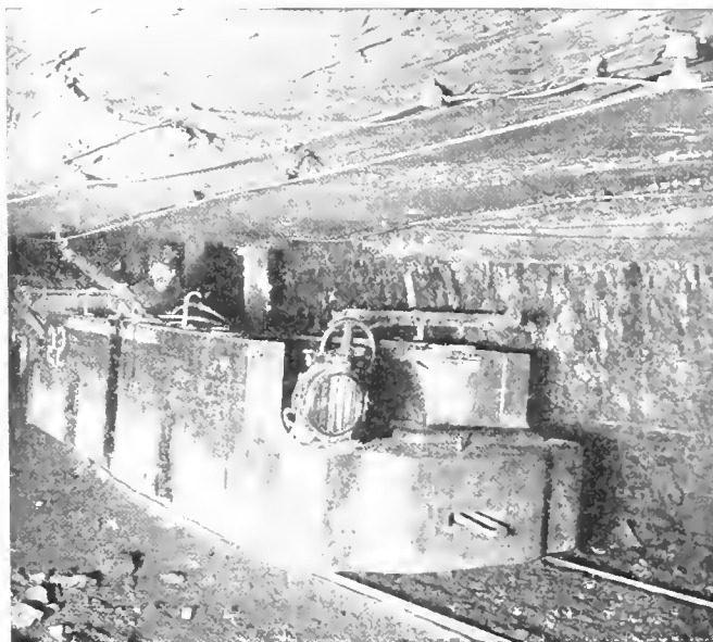
FIG. 2. SHOWING UNEVEN TROLLEY WIRE CAUSED BY HANGER BEING OUT OF PLUMB
