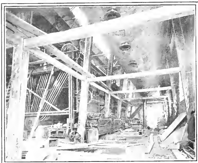
FIG. 15. INTERIOR OF BOILER PLANT
