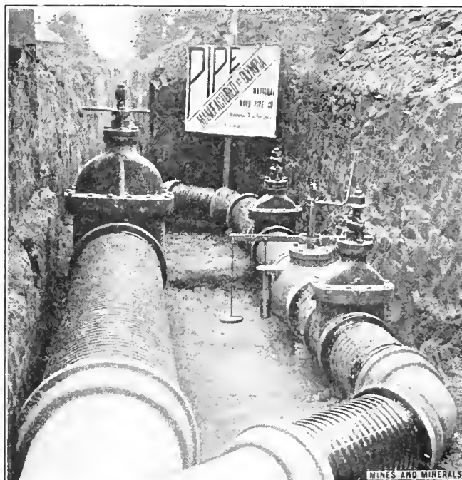
FIG. 3. IRON VALVES, BY-PASS AND PRESSURE REGULATOR ON WOODEN PIPE
