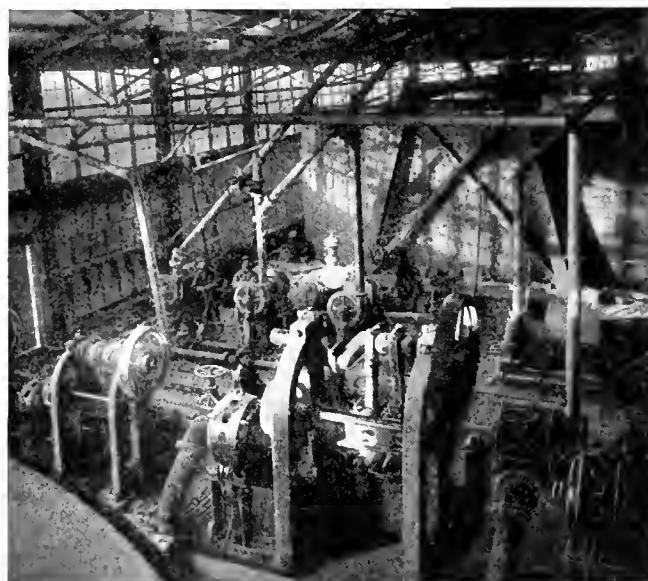
FIG. 2. CENTRIFUGAL PUMPS FOR RETURNING SURPLUS PULP SOLUTION TO STORAGE TANK
