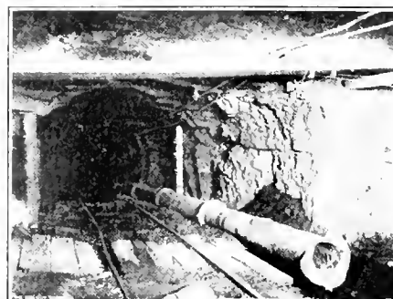
FIG. 2. SHOWING CORROSION OF PIPE
