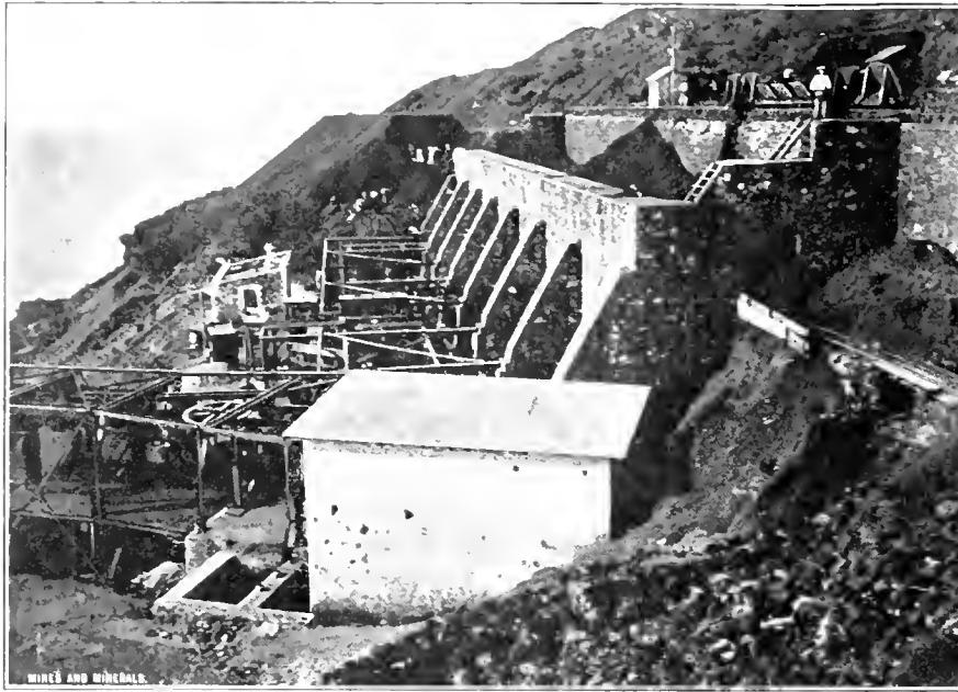
FIG. 2. ORE HOPPER AND LOADING STATION FOR TRAMWAY
