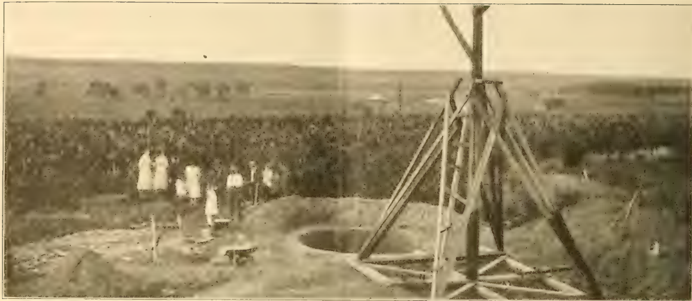
A pit silo in Eastern Colorado. Dry-land sections are well adapted to the construction of the pit silo and it may be built without expert labor at very little cost. It is a good insurance policy for the dry-land farmer.
