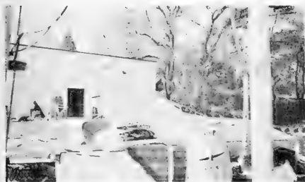
Hurricane damage to Chesapeake Bay shucking house, October 15, 1954.
